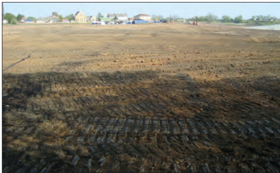
Plate 72: Continuation of linear drains [057] and [065] to the south of the excavation area, from the south.
