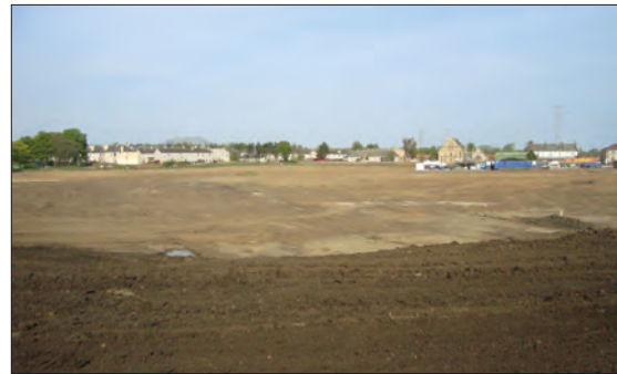
Plate 73: General view of the southern part of the development site after stripping, from the south.
