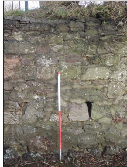
Plate 4: Retaining wall at the churchyard, showing depth of St Mary's Hall site.
