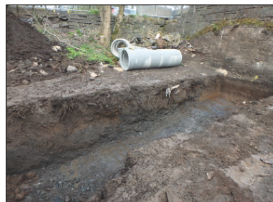
Plate 2: Oblique shot of pipe trench with 005 visible in section – taken from the east.
