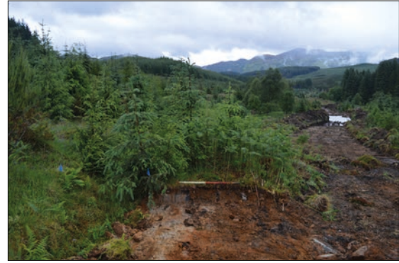
Plate 15: South-west facing section across track at Cuil Muilinn which leads to Big Bruach Caoruinn homestead, blue flags to left of track indicate position of construction trench.
