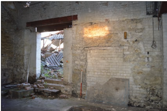
Plate 20: East facing internal elevation earlier mill building with blocked opening and later slapped through large doorway. Steel lintel over doorway rests on top of earlier sandstone building wall heads.
