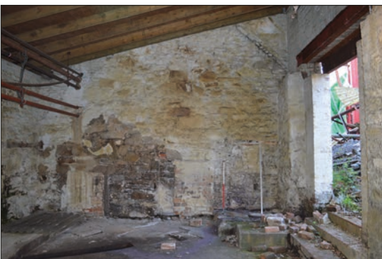
Plate 12: North facing internal elevation of gable wall in the earlier mill building with two blocked fireplaces and a small wall press, three roof scars corresponding to the height of the mill building, later sandstone built extension and the subsequent brick enlargement of the building are visible on top of and above the gable wall top right of frame.
