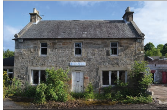
Plate 2: South facing, front elevation of the mill house, enlarged window openings on ground floor.
