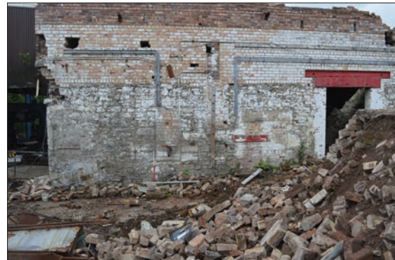
Plate 8: West facing elevation north end of earlier mill building with bricked up openings.
