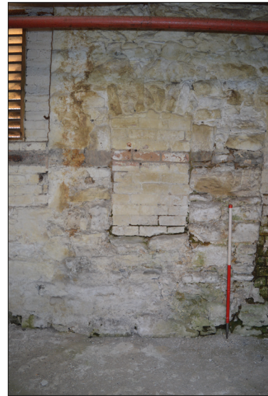
Plate 19: Detail of blocked opening and possible later slapped through opening or remodelled original opening left of frame in west facing internal elevation earlier mill building.
