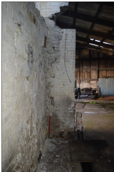
Plate 24: South facing internal elevation of stub end of northern partition?/gable? wall with brick consolidation earlier mill building.
