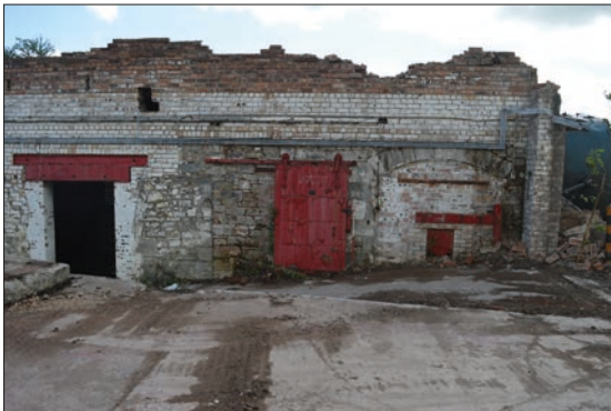
Plate 7: West facing external elevation of south end of earlier sandstone mill building and later sandstone extension showing brick blocking under sandstone arch.
