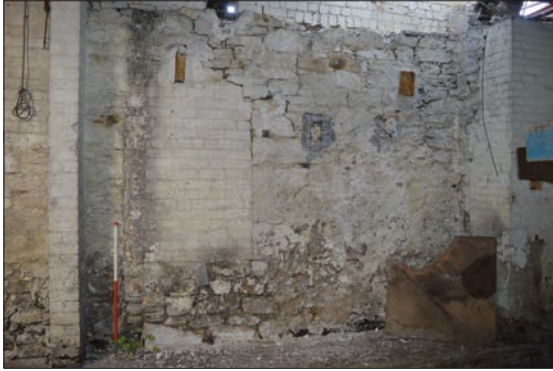
Plate 22: East facing internal elevation earlier mill building (north of previous shots) blocked opening.
