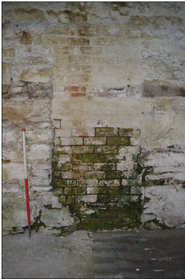
Plate 18: Detail of blocked opening in west facing internal elevation earlier mill building.
