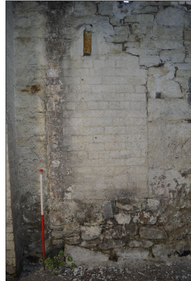
Plate 23: Detail of blocked opening in east facing internal elevation earlier mill building.
