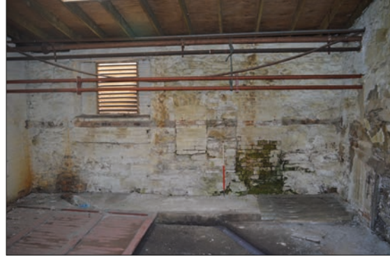
Plate 17: West facing internal elevation earlier building with blocked openings and possible later slapped through opening or remodelled original opening, deep concrete floor with channels visible base of frame.
