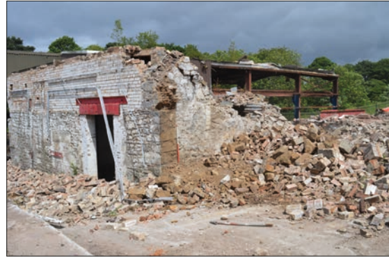
Plate 11: General view of original mid 18 th Century Mill building after removal of 19 th Century extension from the south-west.
