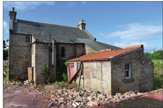
Plate 4: North facing, rear elevation of the mill house with later brick extensions.
