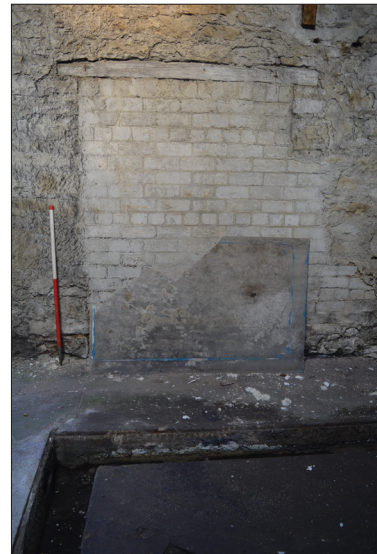
Plate 21: Detail of blocked opening in east facing internal elevation earlier mill building.
