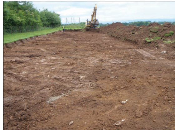
Plate 2: Philipshill Road TRS: East Kilbride. Topsoil stripping within pipeline area viewed from south-east.
