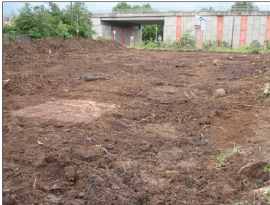
Plate 1: Philipshill Road TRS: East Kilbride. Topsoil stripping within TRS area viewed from north.
