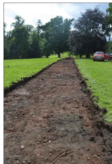
Plate 10: General view after topsoil strip along the access road, from the east.
