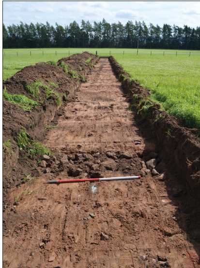
Plate 1: Rubble and tile drain, towards south end of Trench, in Trench 9, from the north.
