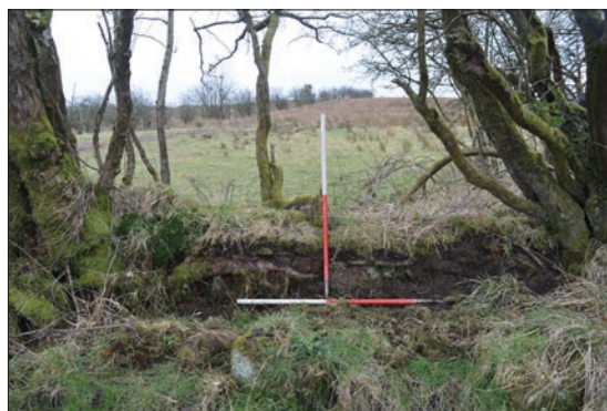
Plate 14: Tree root infiltration in stone wall 007.
