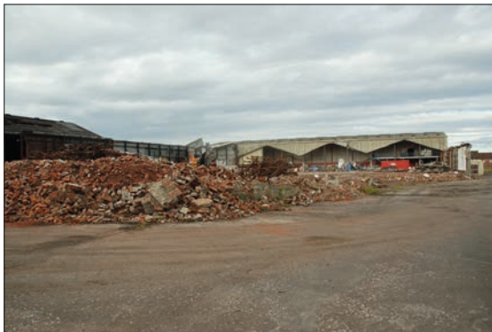
Plate 1: General view of the demolition process from over the Site from the south-east.
