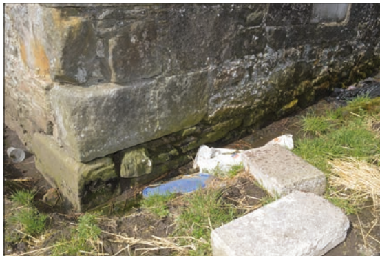
Plate 3: Missing mortar on east wall of West Range
