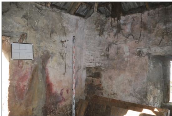
Plate 6: Room 1 of West Range with white wash on walls and brick flue in south-west corner
