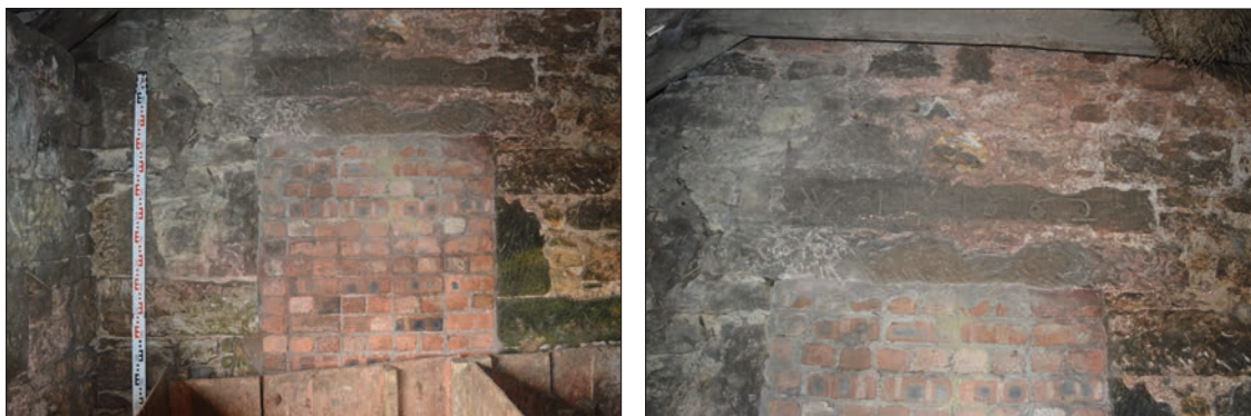
Plates 14 and 15: Brick blocked doorway in Room 4, East Range with inscribed lintel
