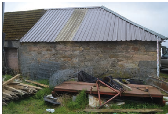
Plate 5: Corrugated sheeting on roof of North Range and crack in stonework
