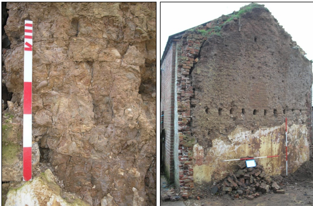
Figure 6 and 7. Detail of clay dabbins and eastern elevation showing clay dabbin wall
