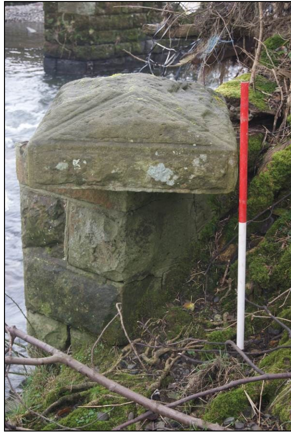
Figure 33. Surviving flank of western abutment
