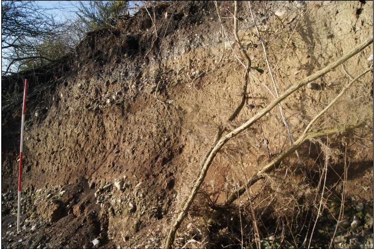
Figure 14. Eroded bank, location for the former western bridge abutment
