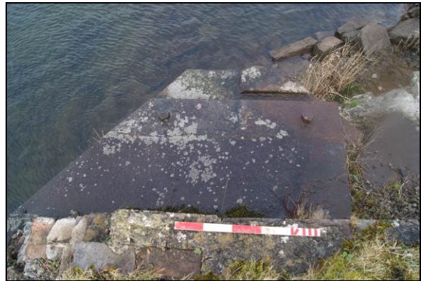
Figure 45. Iron plate on bridge abutment
