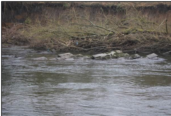
Figure 47. Location of fallen Pier 2
