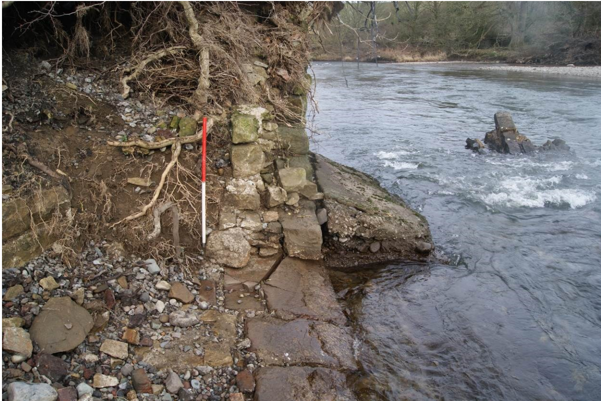
Figure 35. Western bridge abutment showing a cross-section through the former stone wall skin
