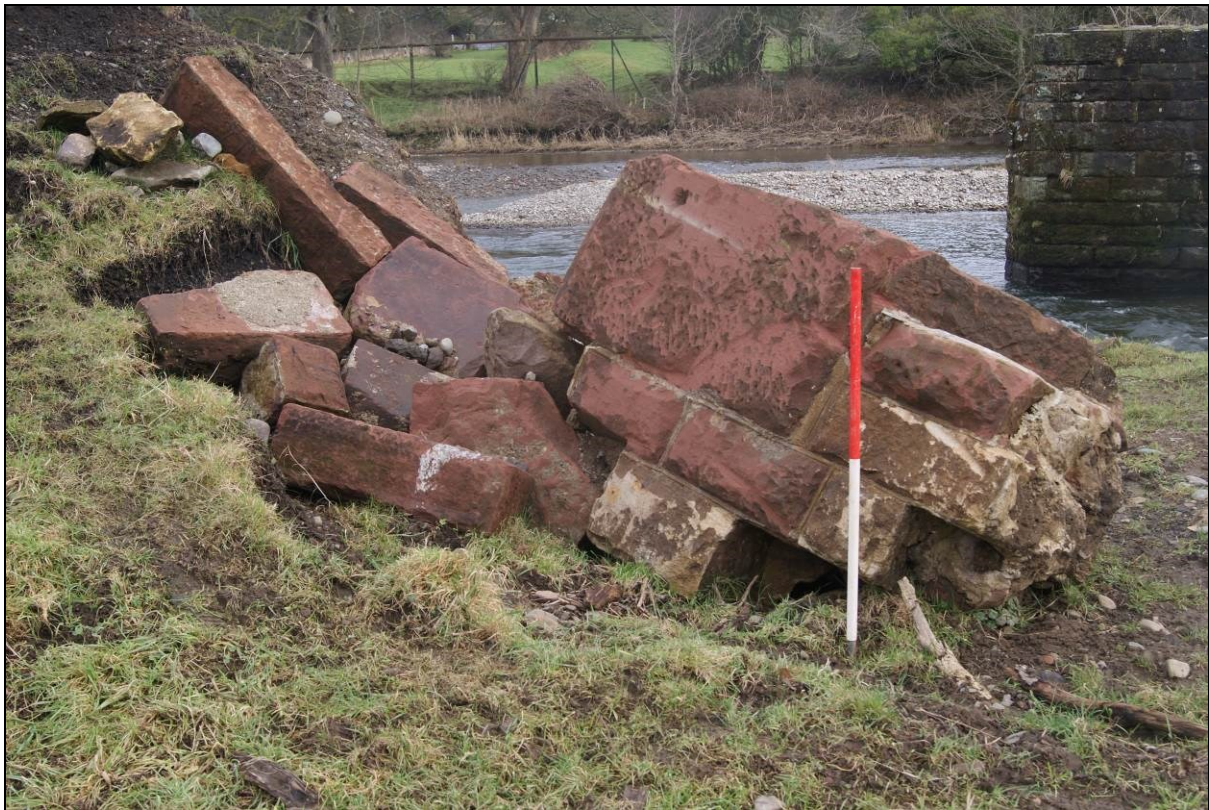
Figure 34. Debris from the former western bridge abutment
