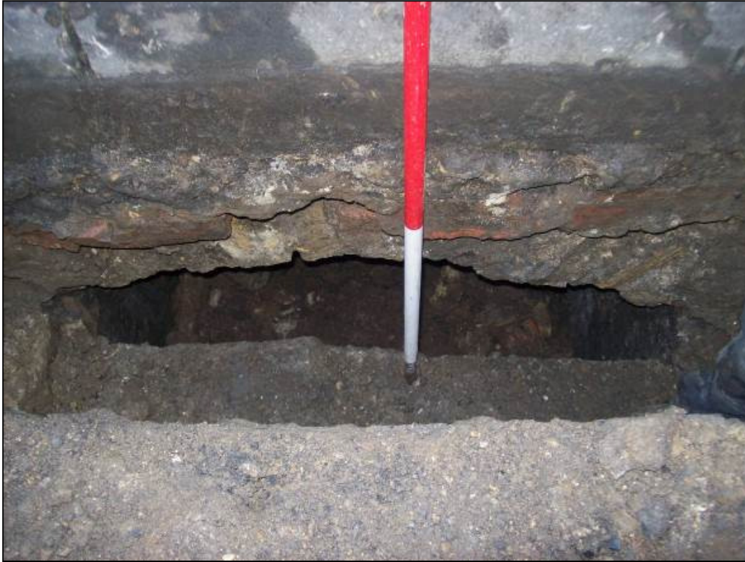
Figure 11 - Void Revealing Southern Vault
