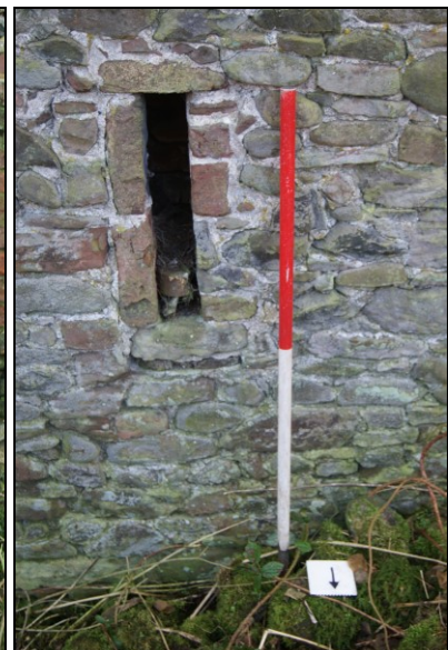
Figure 28. Air vent (13), Room 3
