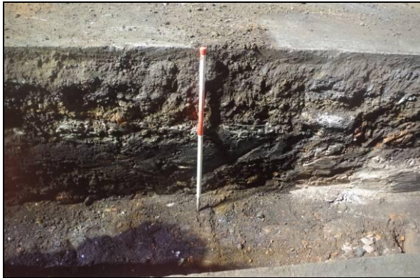
Figure 10. Section in the cable trench
