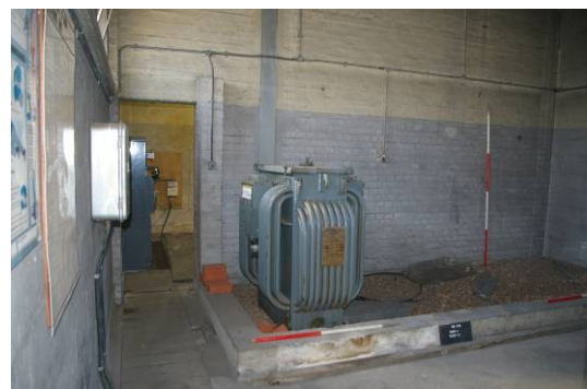
Figure 28. Transformer on south side of room 2 looking south.
