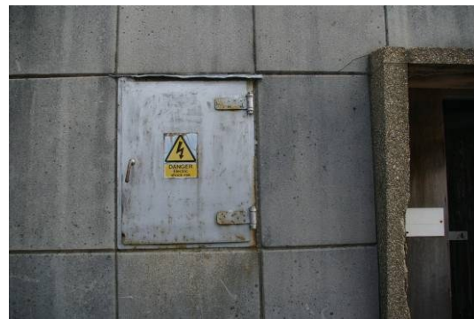
Figure 34. Hatch door to external switch box in south wall, looking north.
