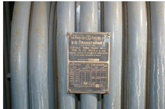
Figure 27. Maker's plaque on north-east transformer looking north.
