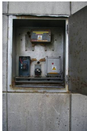
Figure 35. Interior of switch box looking north.
