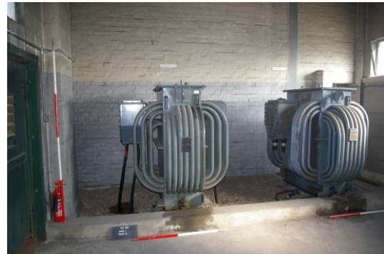
Figure 26. Transformers on north side of room 2 looking north.
