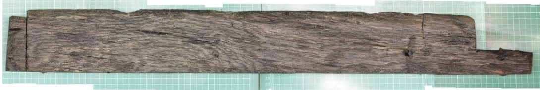
Figure 64 Photograph of timber 74
