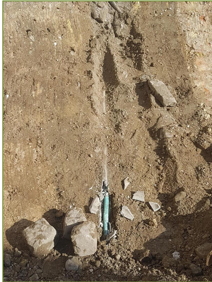
DP20; Test Pit 5 – Service pipe showing service run and level that excavation ceased.
