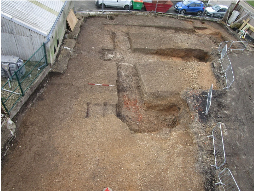
Photo 56. G36 concrete-lined air raid shelter construction trench cutting fills of G31 quarry pits, looking southwest (scale 2m)
