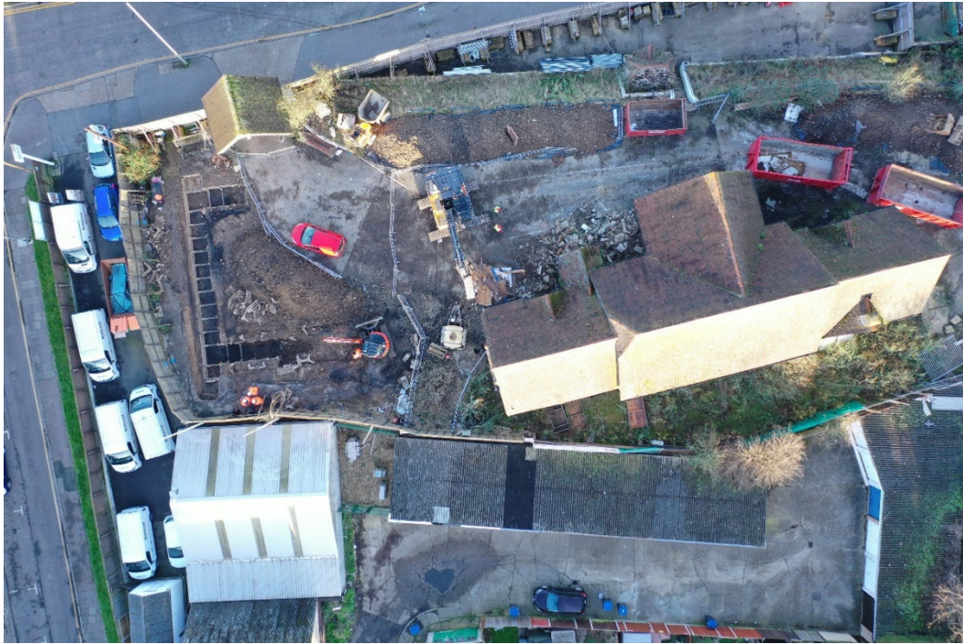
Photo 1. Aerial view of PDA showing G36 concrete-lined air raid shelter prior to demolition of former St Mary Bredin School building, looking northwest (no scale)
