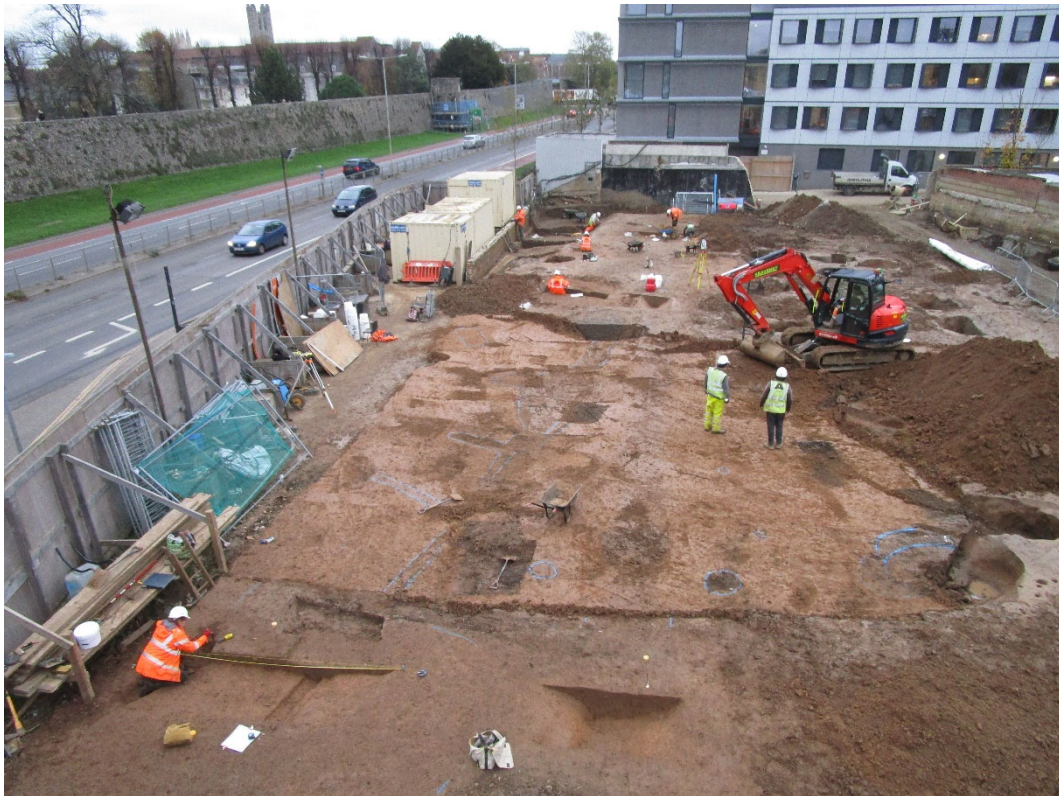
Photo 13. Machine removal of G9 soil horizon in progress, looking northeast (no scale)
