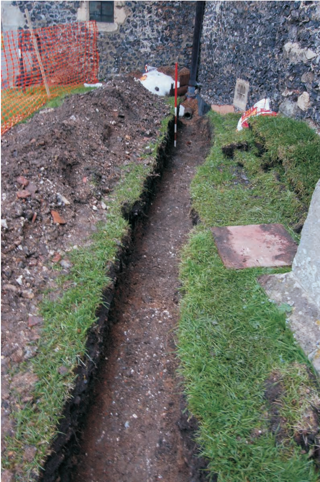
Plate 12: Southern pipe trench near the south porch, the southern edge straightened, looking west (Scale 1m)
