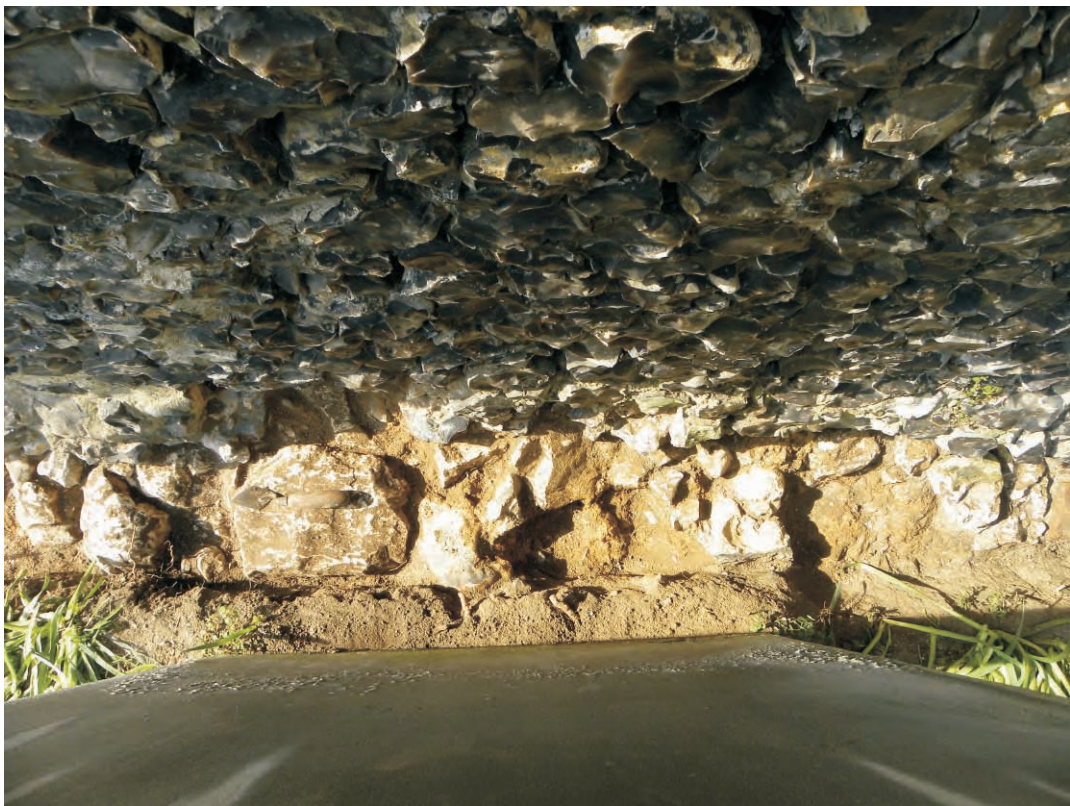
Plate 17: South transept foundation disturbed by gravestone foundation
