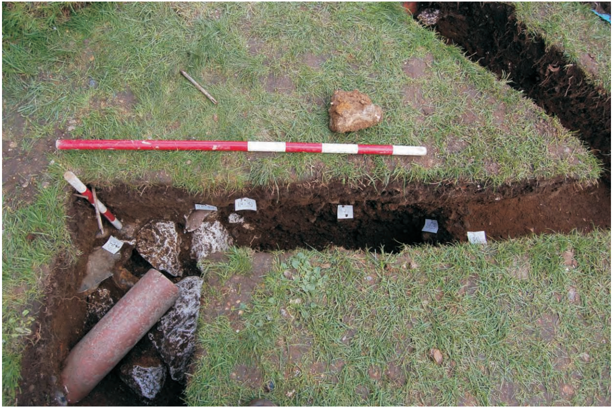
Plate 14: South-east pipe trench extension and void, looking east (Scale 1m and 0.5m)
