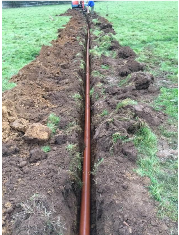
Plate 4: Trench for the new outfall pipe (in place) as viewed from the south. No scale.
