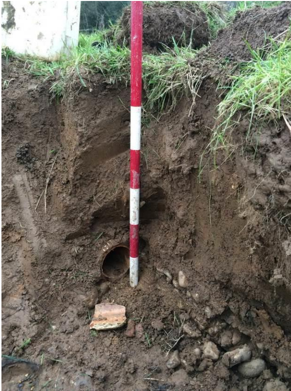
Plate 3: Existing outfall pipe as exposed in the northerly explorative test-pit. Scale 1m.
