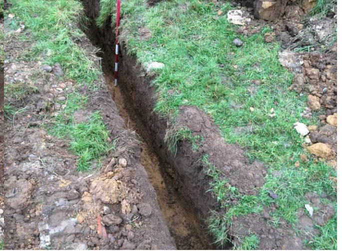
Plate 2: Deepest section of the service trench for the new outfall pipe. Scale 1m.
