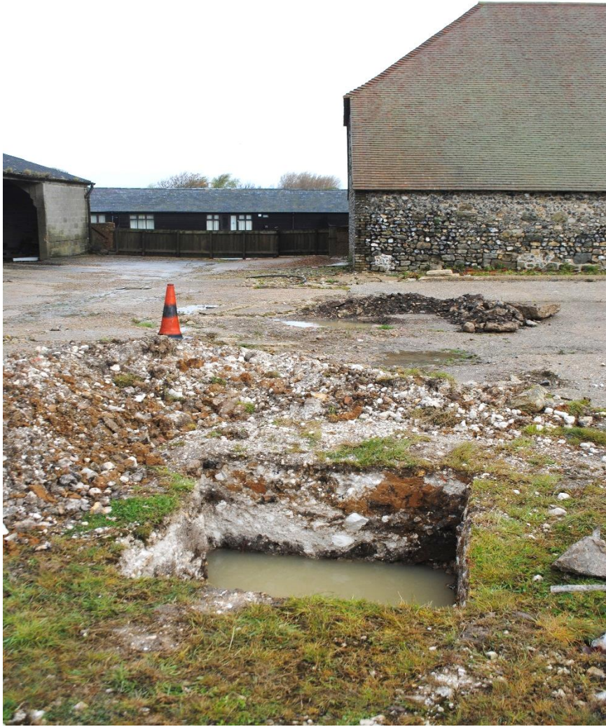
Plate III Position of Test Pit 1 (foreground) and Test Pit 2 in relation to the Stone Barn, looking north
