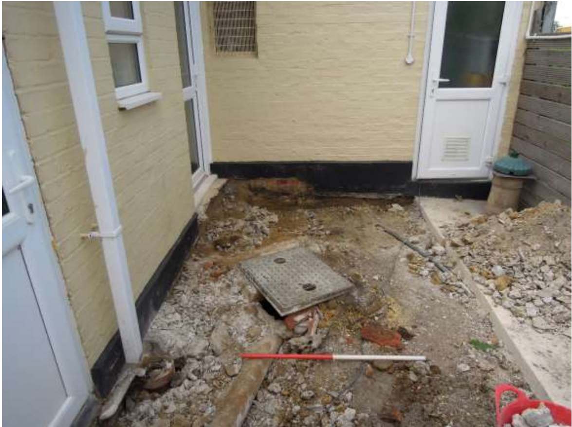
Fig. 4 General view of the excavated area, showing inspection chamber, looking west. Scale, 1m
