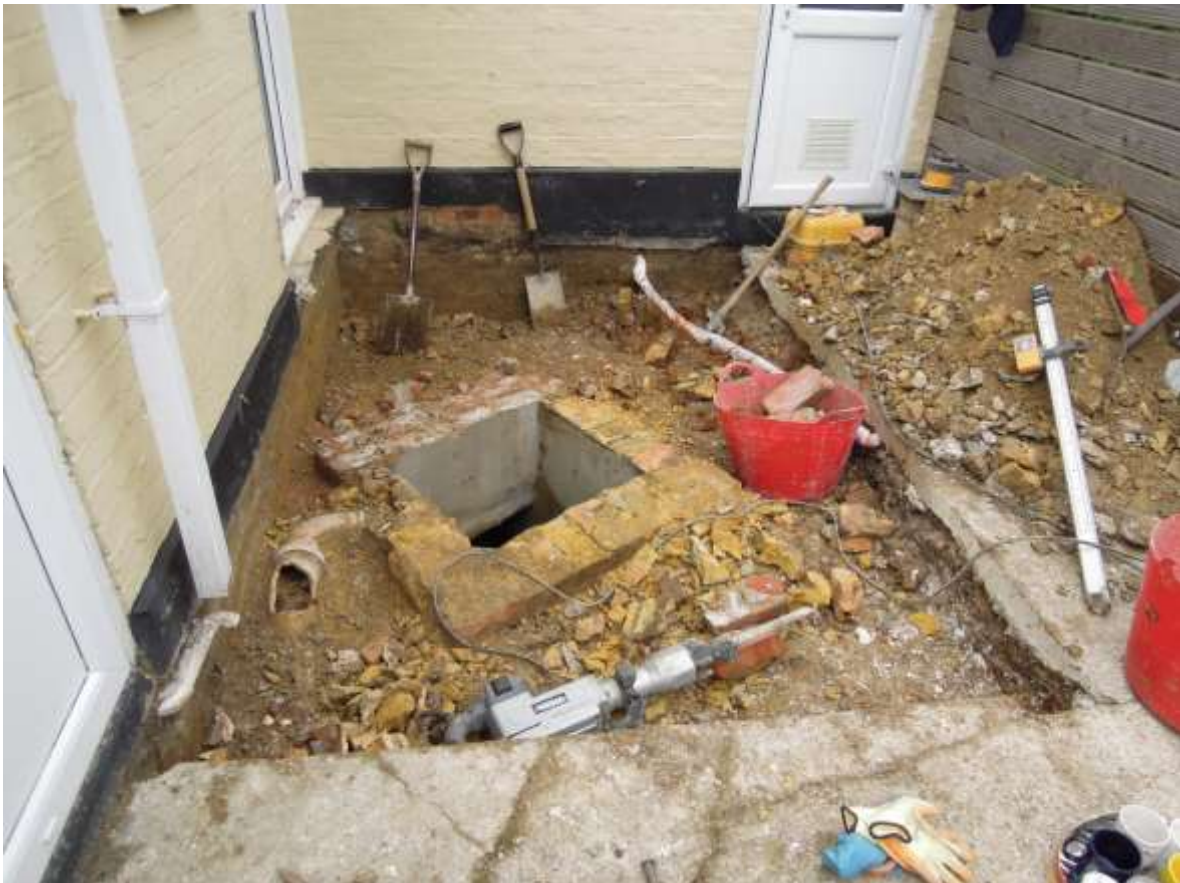
Fig. 5 The top of the inspection chamber removed and the area reduced to final level, looking west
