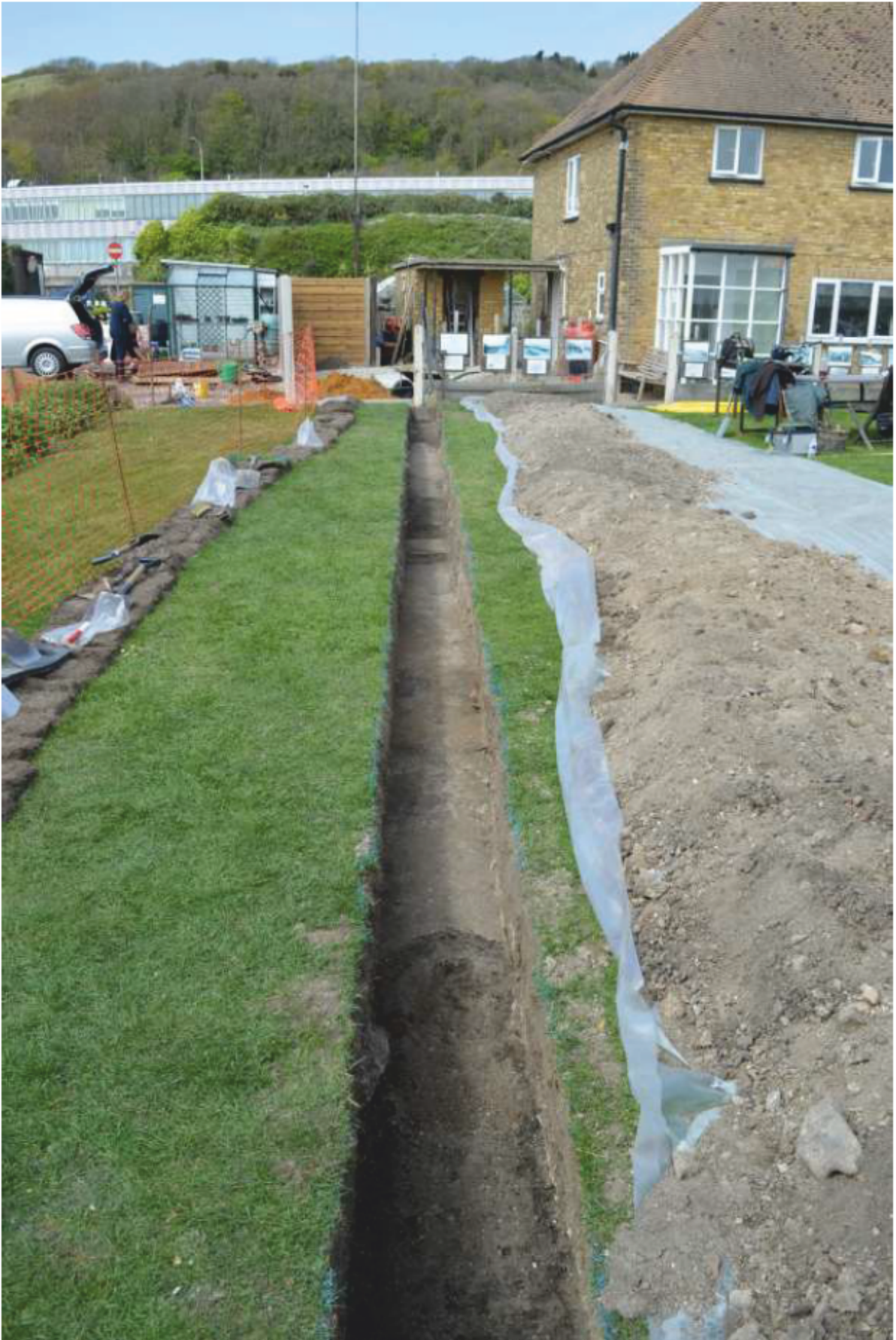
Frontispiece General view of the excavated trench showing buried yard surface, looking north-west
