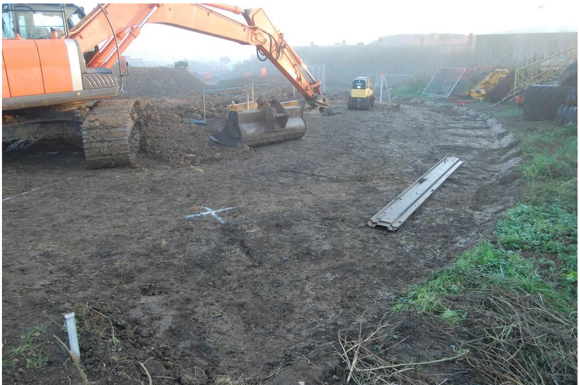
Plate 12. Southern end of Eastchurch Scheme (chainage 800–875m area), after topsoil strip, as viewed from the south-south-west. No scale.
