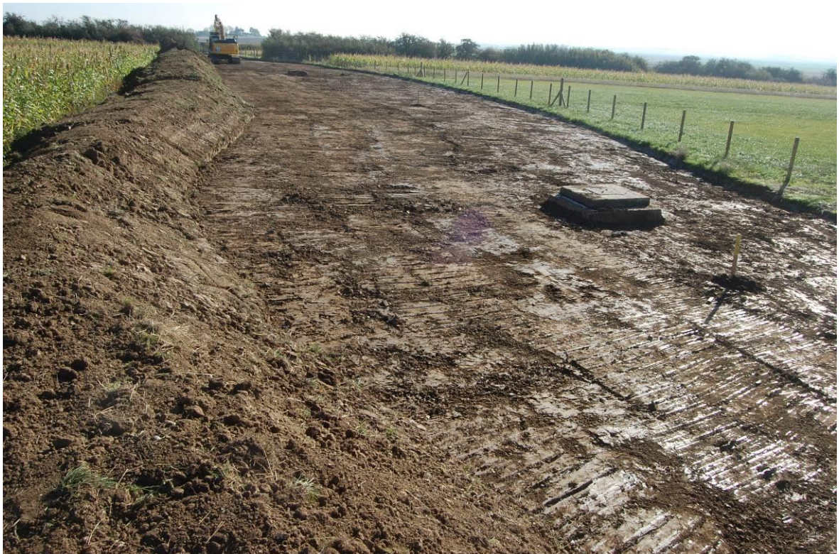
Plate 2. View taken from the extreme western end of the Eastchurch scheme (chainage 0–135m area) during the initial topsoil strip, as viewed from the west. No scale.
