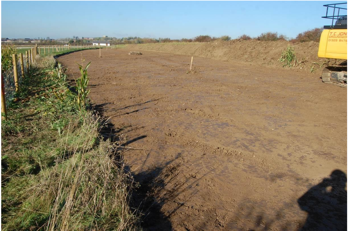
Plate 3. View taken from the eastern end of the Eastchurch scheme (chainage 0–135m area) during the initial topsoil strip, as viewed from the east. No scale.
