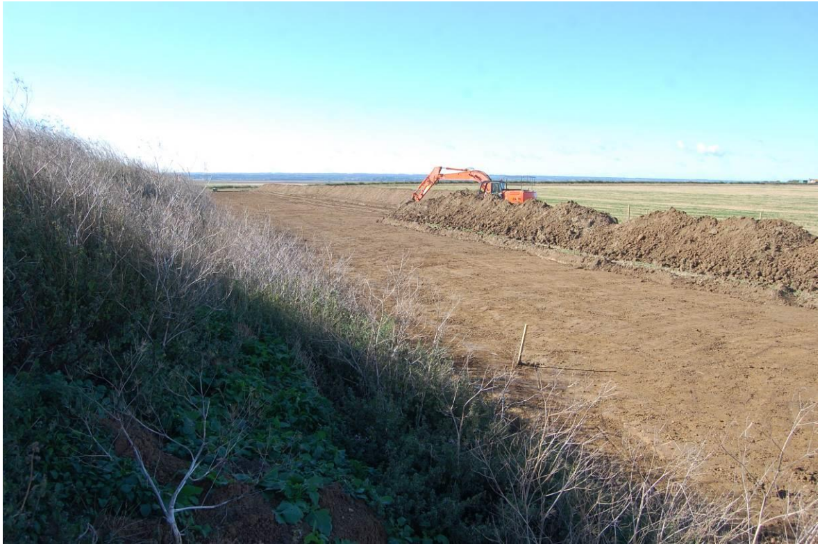
Plate 9. Northern end of Eastchurch Scheme (chainage 575–800m area), after machine reduction down to the upper surface of the exposed London Clay, as viewed from the north-east. No scale.
