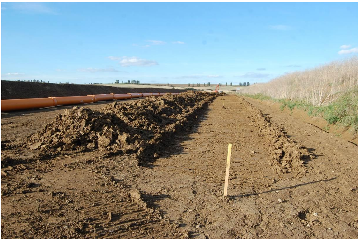
Plate 10. Southern end of Eastchurch Scheme (chainage 575–800m area), after further machine reduction of the disturbed London Clay upper horizon, as viewed from the south. No scale.
