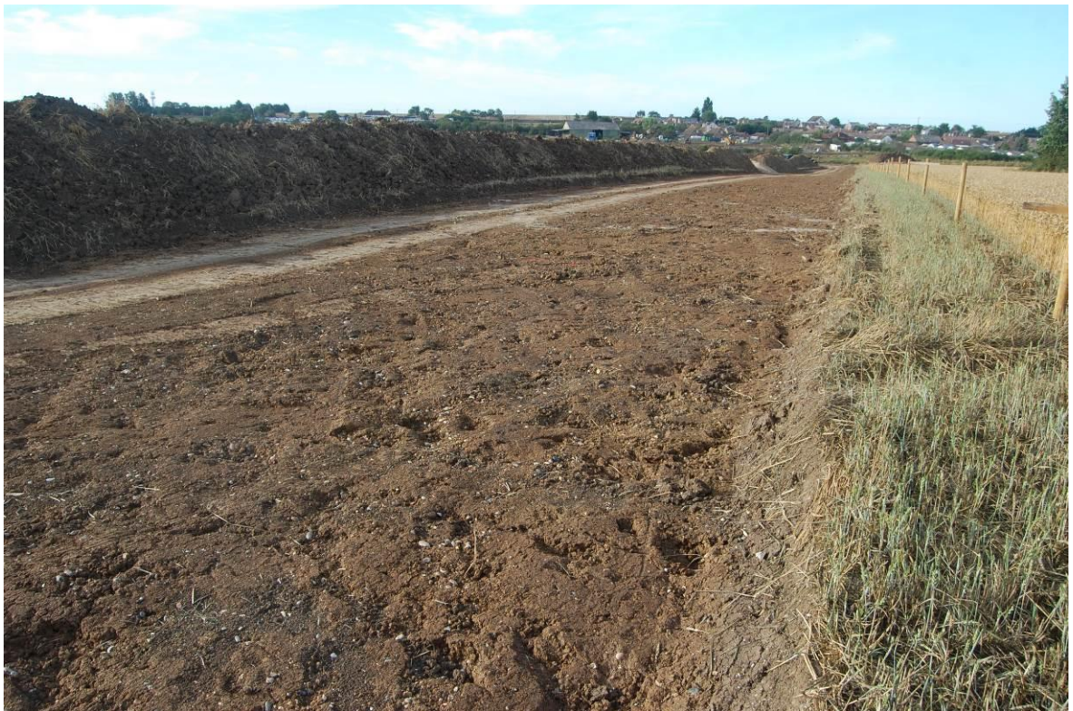
Plate 16. View of the north-north-east to south-south-west section of the Warden Bay scheme, from its north-eastern end, after machine reduction to the exposed upper surface of the London Clay. No scale
