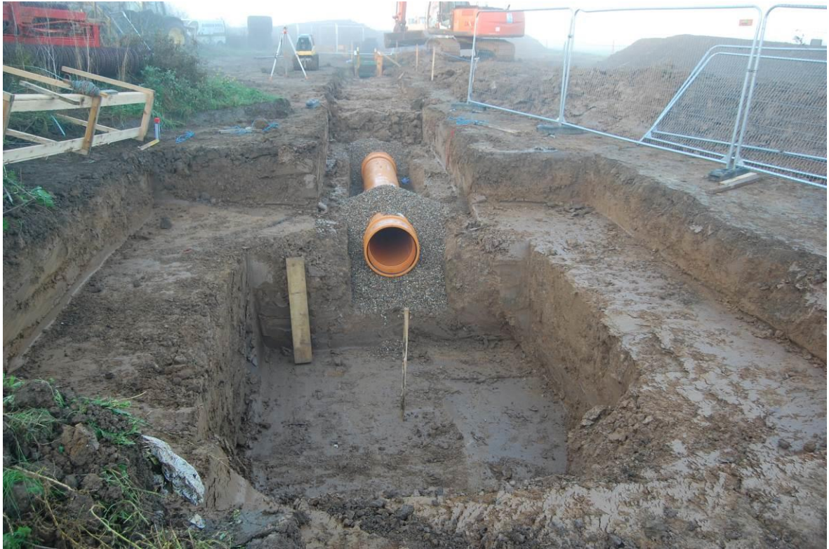
Plate 13. Reduced area for man-hole location at the northern end of the Eastchurch Scheme (chainage 575–800m area), as viewed from the east. No scale.
