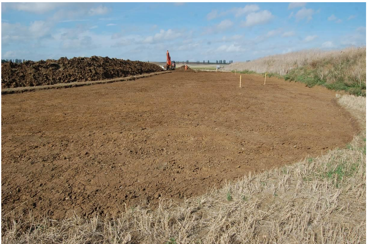
Plate 8. Southern end of Eastchurch Scheme (chainage 575–800m area), after machine reduction down to the upper surface of the exposed London Clay, as viewed from the south. No scale.
