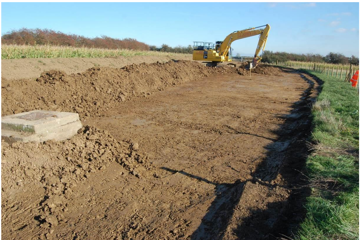
Plate 4. View taken from the eastern end of the Eastchurch scheme (chainage 0–135m area) during the lower subsoil strip down to natural London Clay as viewed from the west. No scale.
