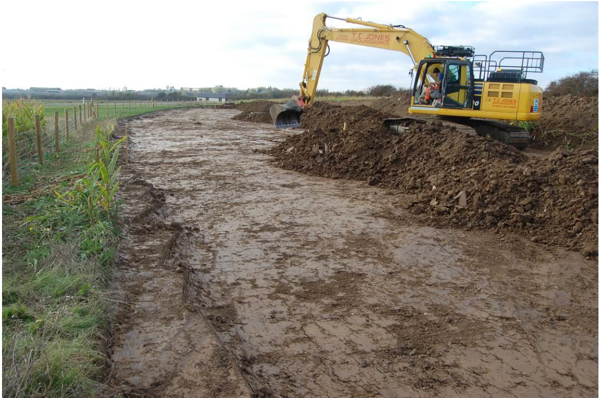
Plate 5. View taken from the extreme eastern end of the Eastchurch scheme (chainage 0–135m area) during the lower subsoil strip down to natural London Clay as viewed from the east. No scale
