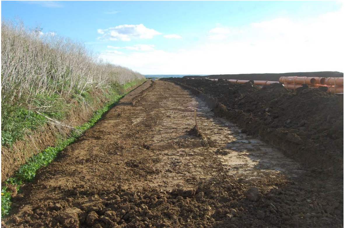
Plate 11. Northern end of Eastchurch Scheme (chainage 575–800m area), after further machine reduction of the disturbed London Clay upper horizon, as viewed from the north. No scale.
