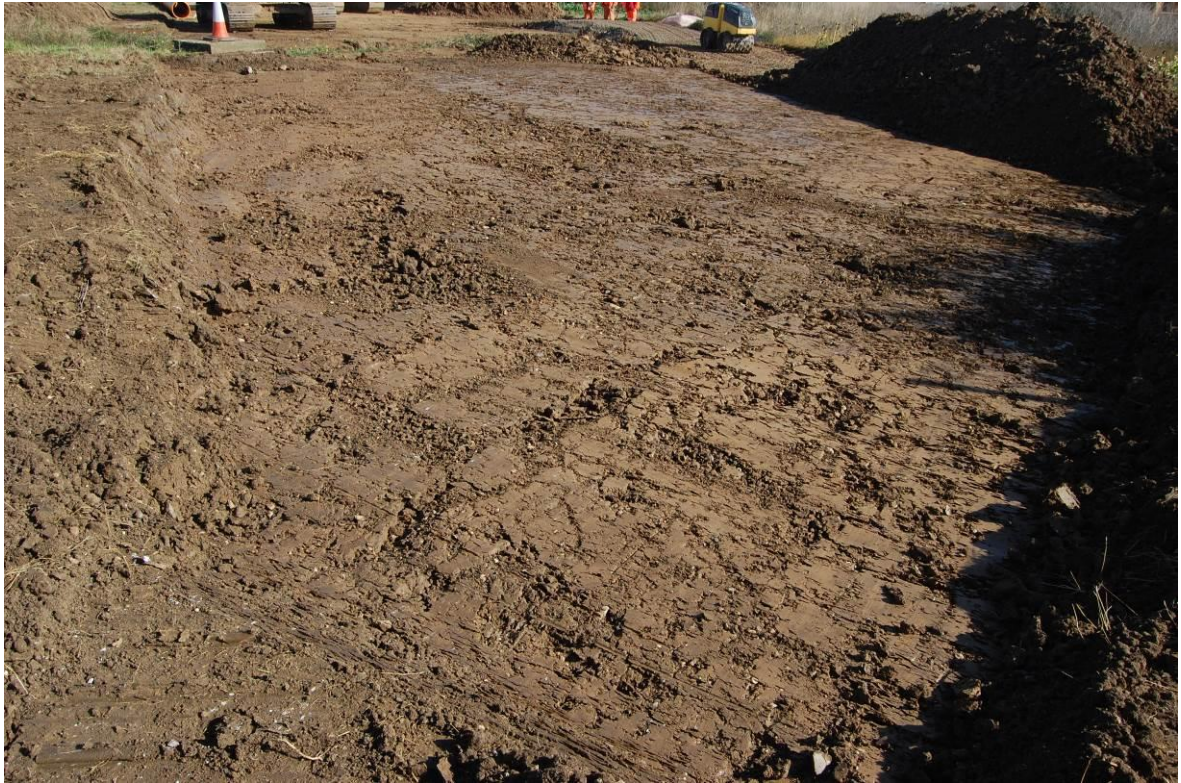
Plate 7. Eastchurch Scheme (chainage 540–575m area), after machine reduction down to the upper surface of the exposed London Clay, as viewed from the south-south-west. No scale.
