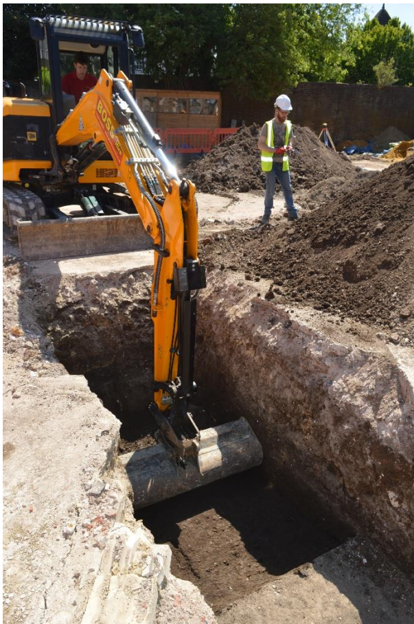
Plate 5. Trench 1 machine excavation of deep sondage at south-east end, looking south (no scale)
