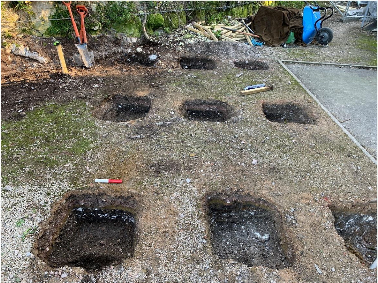
Fig. 4 General view of hand excavated pits looking north-east to the corner of the site. Scale, 20cm
