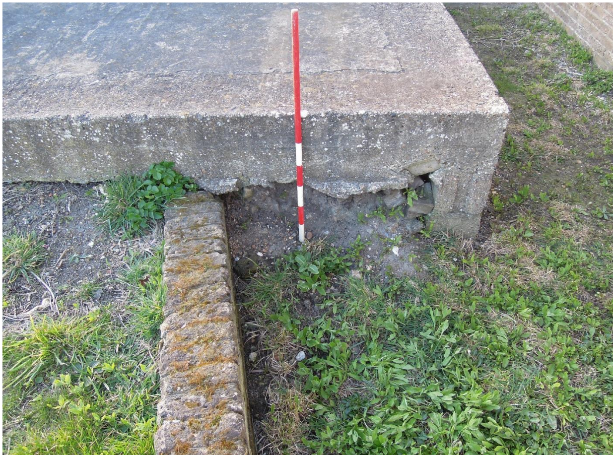
Fig. 10 Detail of concrete building platform at east corner, looking north-west. Scale, 1m
