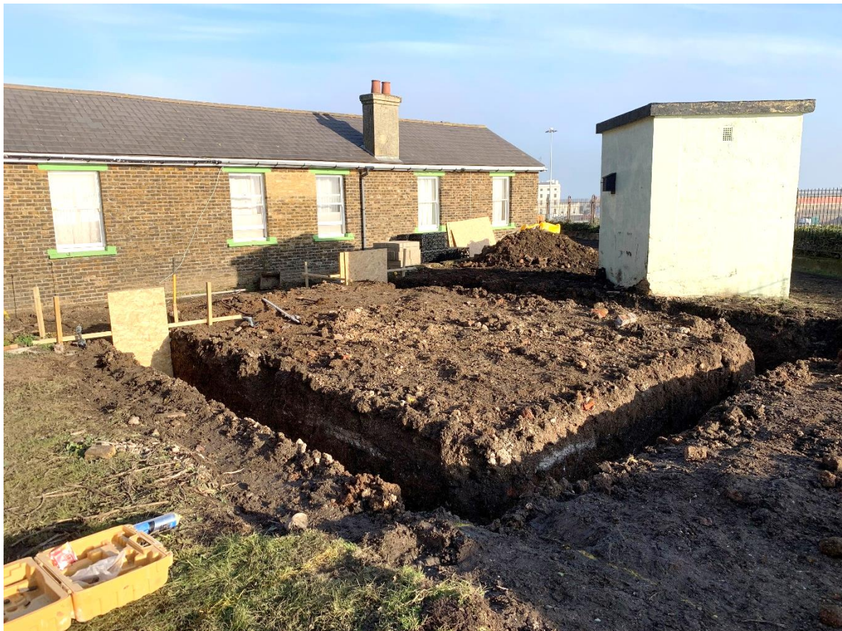
Fig. 10 General view of excavated foundation trenches, looking east with Buildings 4 and 5 in background
