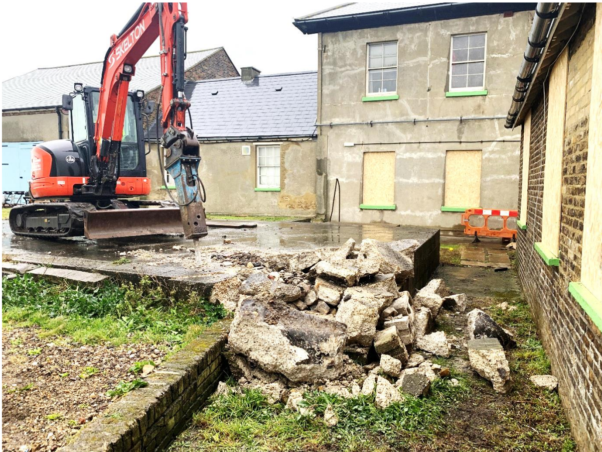
Fig. 9 Breaking out the concrete platform of Building 9, looking west (note brick retaining wall 403)
