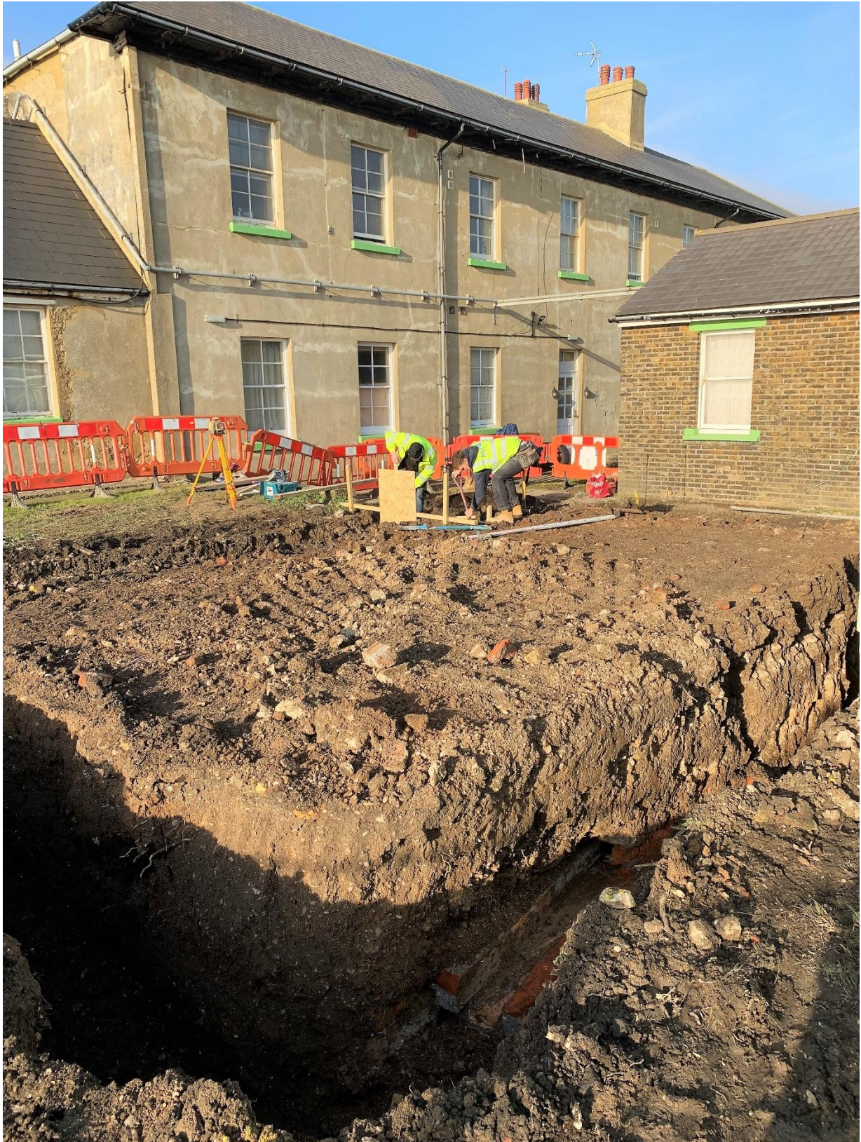
Frontispiece General view looking north across the site with concrete platform of Building 9 removed and new foundation trenches cut (Buildings 2 and 4 in background)
