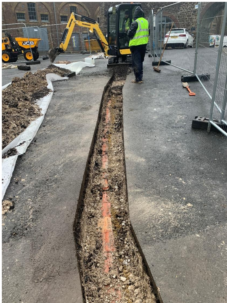
Fig. 5 Trenching between Test Pits 6 and 1, showing earlier cable line marked by cover tiles, looking north
