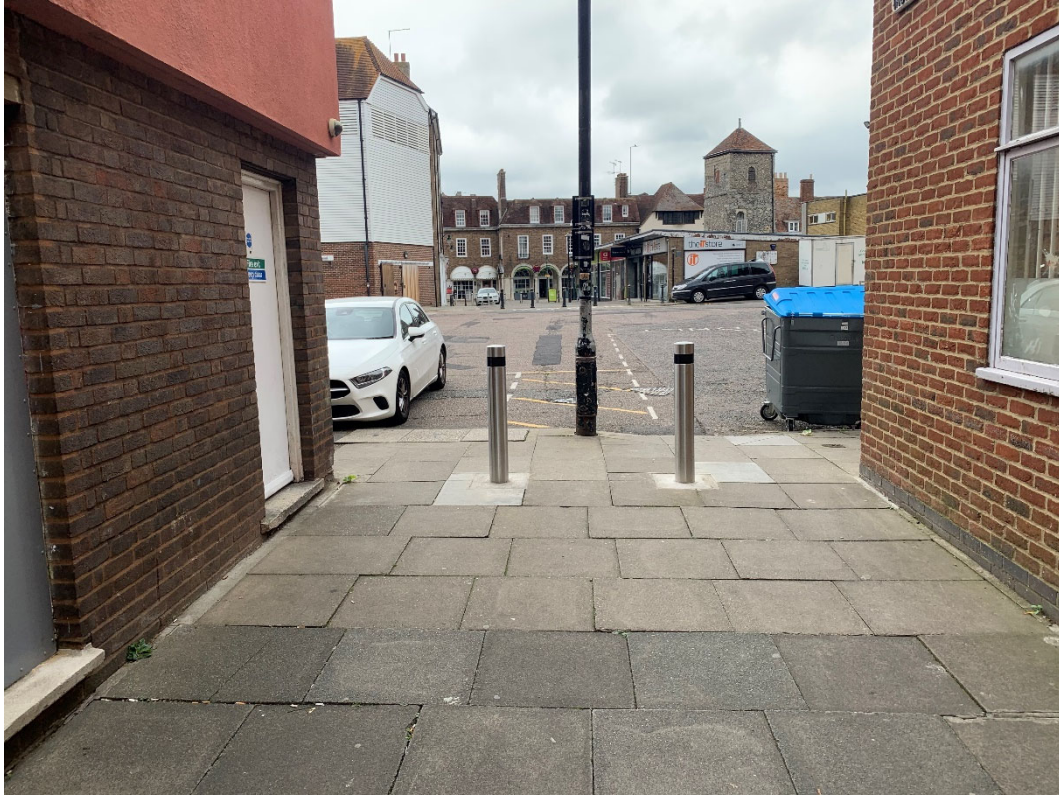
Photo 40. Site 20 St George's Street to Iron Bar Lane Passage, trench location post-installation, looking north-east (no scale)
