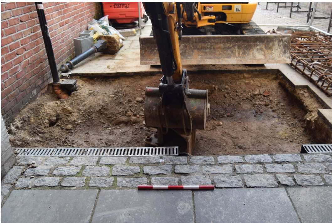
Photo 39. Site 19 Longmarket to Iron Bar Lane Passage, excavated trench, looking south-east (scale 0.5m)
