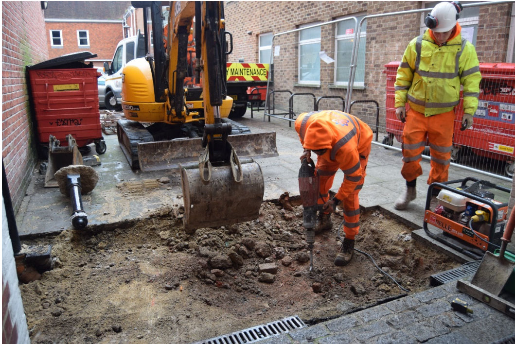
Photo 39. Site 19 Longmarket to Iron Bar Lane Passage, trench location, looking south-east (no scale)
