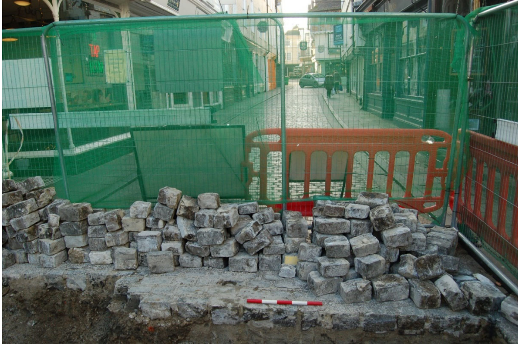
Photo 19. Site 10 Sun Street, trench location, looking south-east (scale 0.5m)
