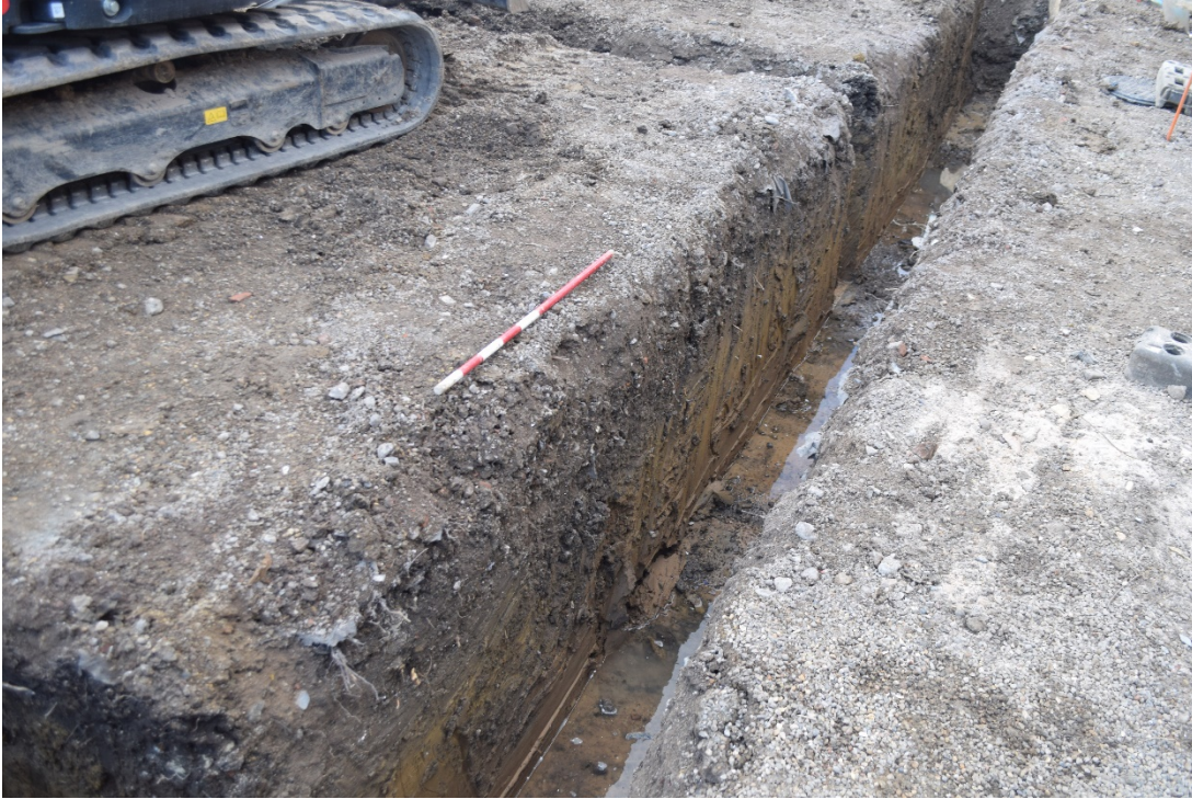
Plate 3. North-west facing section showing geology 115 overlain by deposit 114 looking west scale 1m
