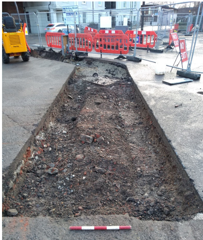
Photo 28. Watling Street Car Park, new entry/exit barrier island footprint, looking east (scale 0.5m)
