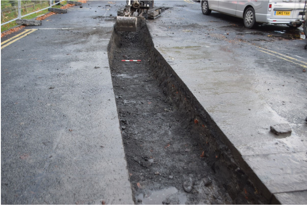
Photo 9. Miller's Field Car Park, fully excavated duct trench, looking west (scale 0.5m)
