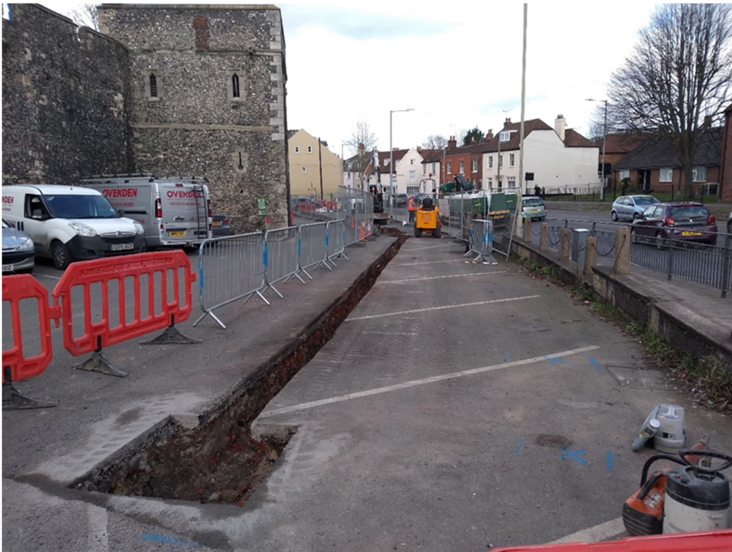
Photo 34. Queningate Car Park, general view of machine excavated duct trench looking north (no scale)
