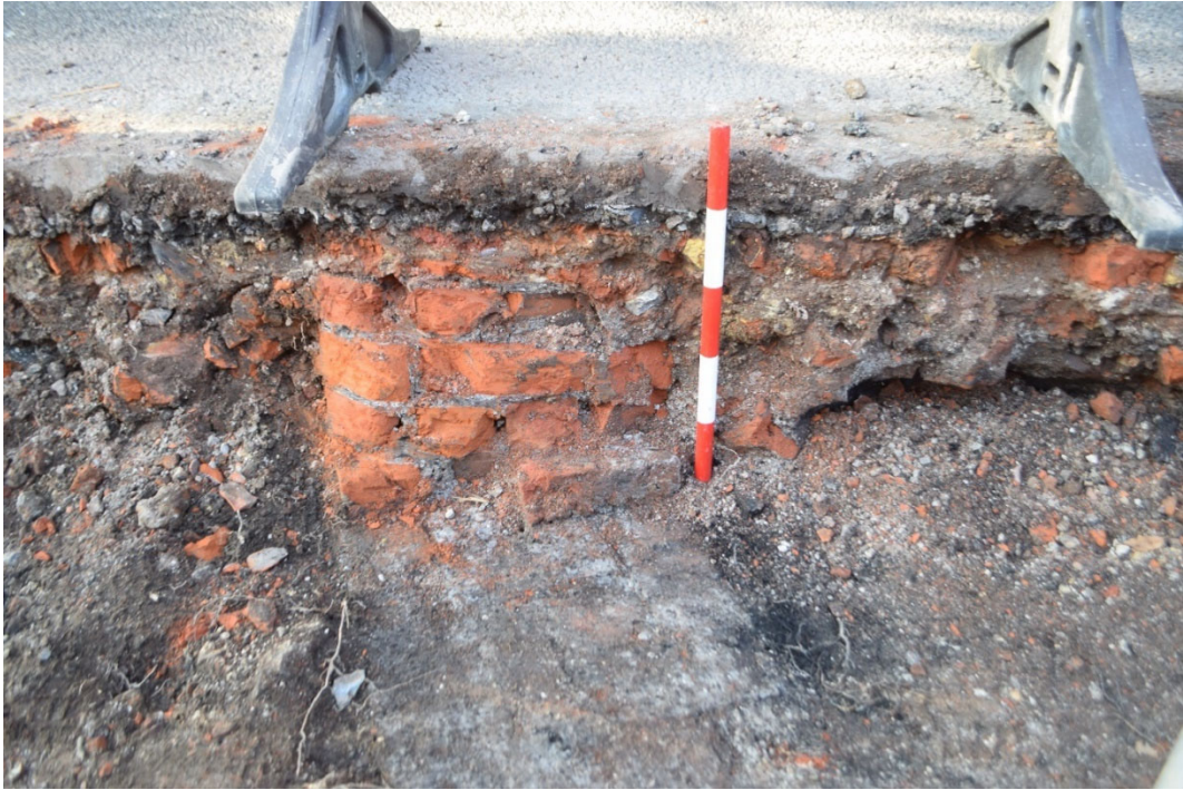
Photo 3. St Radigund's Car Park, trench section through brick wall 1501 and rubble deposit 1503, looking south-west (scale 0.5m)
