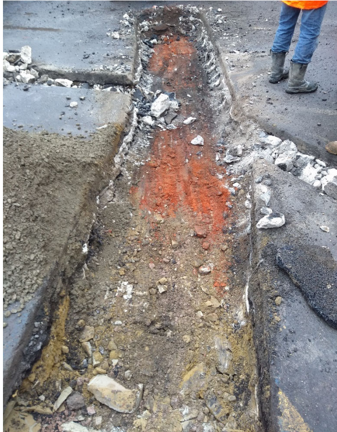
Photo 33. Queningate Car Park, machine excavated exit barrier island footprint, looking south-west (no scale)
