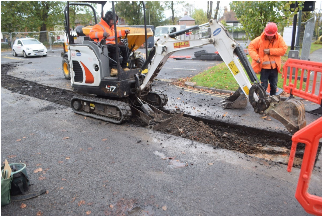
Photo 8. Miller's Field Car Park, general view of duct trench machine excavation, looking north-west (no scale)
