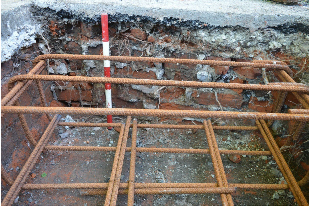
Photo 14. Marlowe Theatre Area 3 bollard installation trench, brick floor 3004 and brick wall 3005, looking south-east (scale 0.5m)
