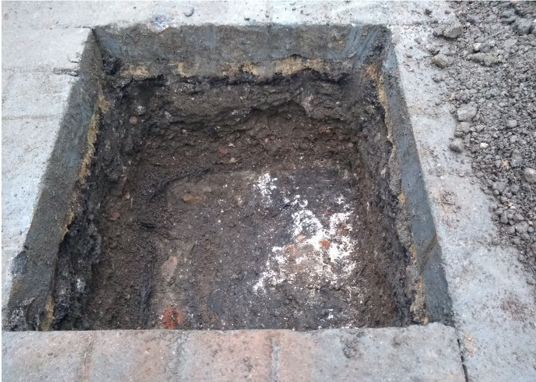
Photo 8. Marlowe Theatre Area 2 security gate installation trench P3, looking north-west (no scale)
