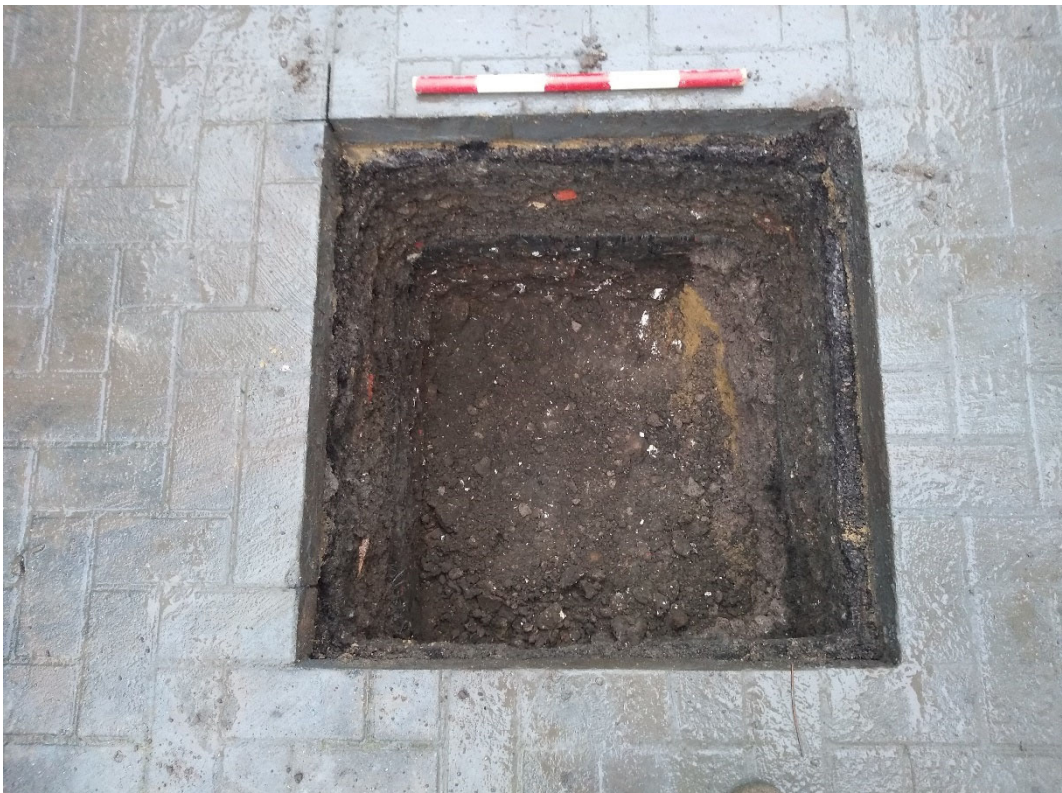
Photo 9. Marlowe Theatre Area 2 security gate installation trench P4, looking south-west (scale 0.5m)
