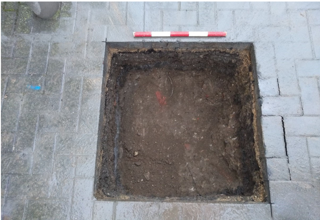
Photo 7. Marlowe Theatre Area 2 security gate installation trench P2, looking south-east (scale 0.5m)
