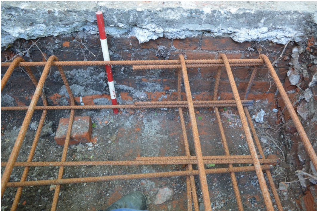
Photo 13. Marlowe Theatre Area 3 bollard installation trench, brick wall 3003 and brick floor 3004, looking north-east (scale 0.5m)
