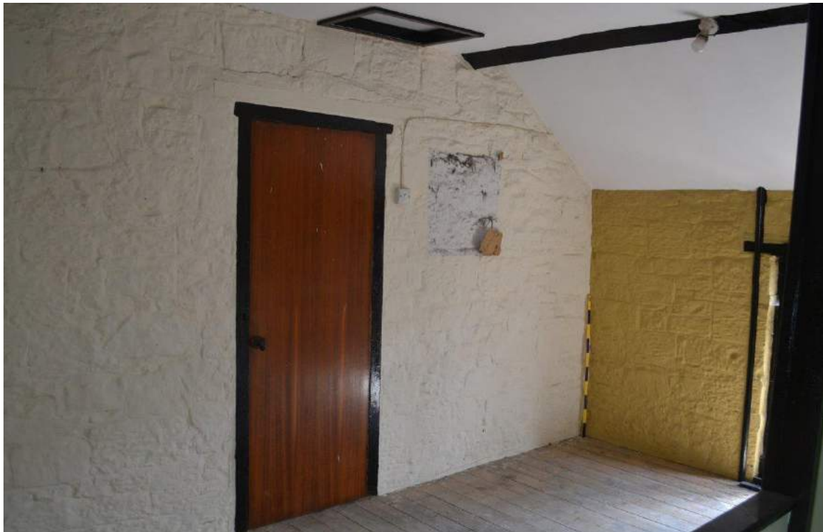
Plate 83: First floor, Workshop. View of the wall dividing the Workshop from the stable with doorway. The timber floor boards are 13.5cm wide
