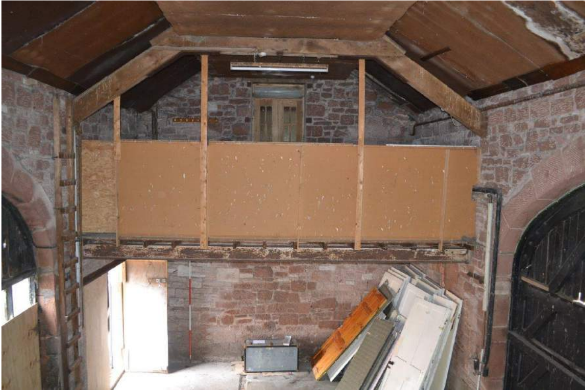
Plate 23: Sightline to the mezzanine floor at the northern end of the barn highlighting the joists, rolled steel joist and safety boarding. Also visible are the porte-fenêtre into the first floor of the stable.
