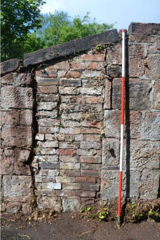
Plate 96: Detail of the bricked-up door way in the east-facing elevation of the pigsty
