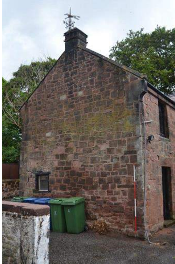
Plate 61: Oblique sightline to the north-east towards the west-facing gable elevation of the workshop. Highlights capped chimney-in-gable-wall, coping-at-gable, projecting corbelled gable skew and window opening to ground floor gable elevation.
