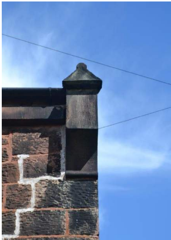
Plate 62: Sightline to the east-facing elevation of the workshop showing detail of the finely dressed projecting corbelled gable skew with roll-topped, pyramidal coping terminal and fascia
