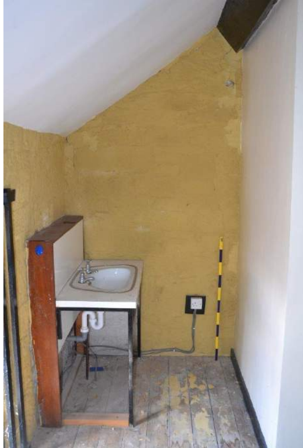
Plate 82: First floor, Workshop, view into alcove formed by partition wall to staircase. Note exposed canted purlin. Scale = 1m.
