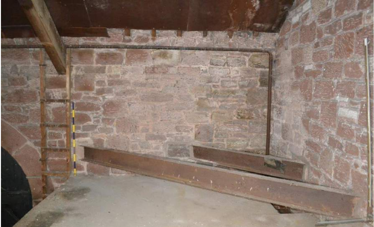
Plate 24: Detail of the diagonal pair of rolled steel joists linking the gable wall to the east-facing flank wall (scale = 1m)
