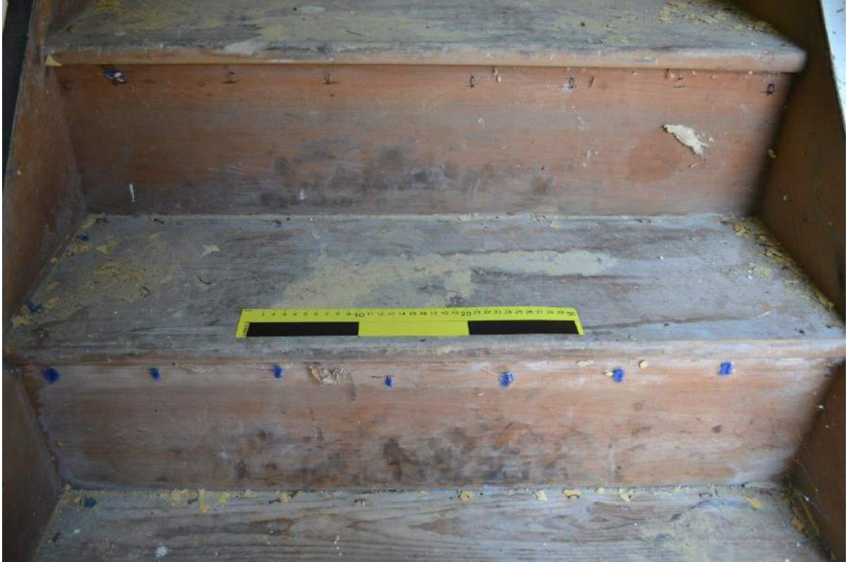
Plate 78: Ground floor, Workshop, detail of tread and riser of timber stair case Scale = 30cm.
