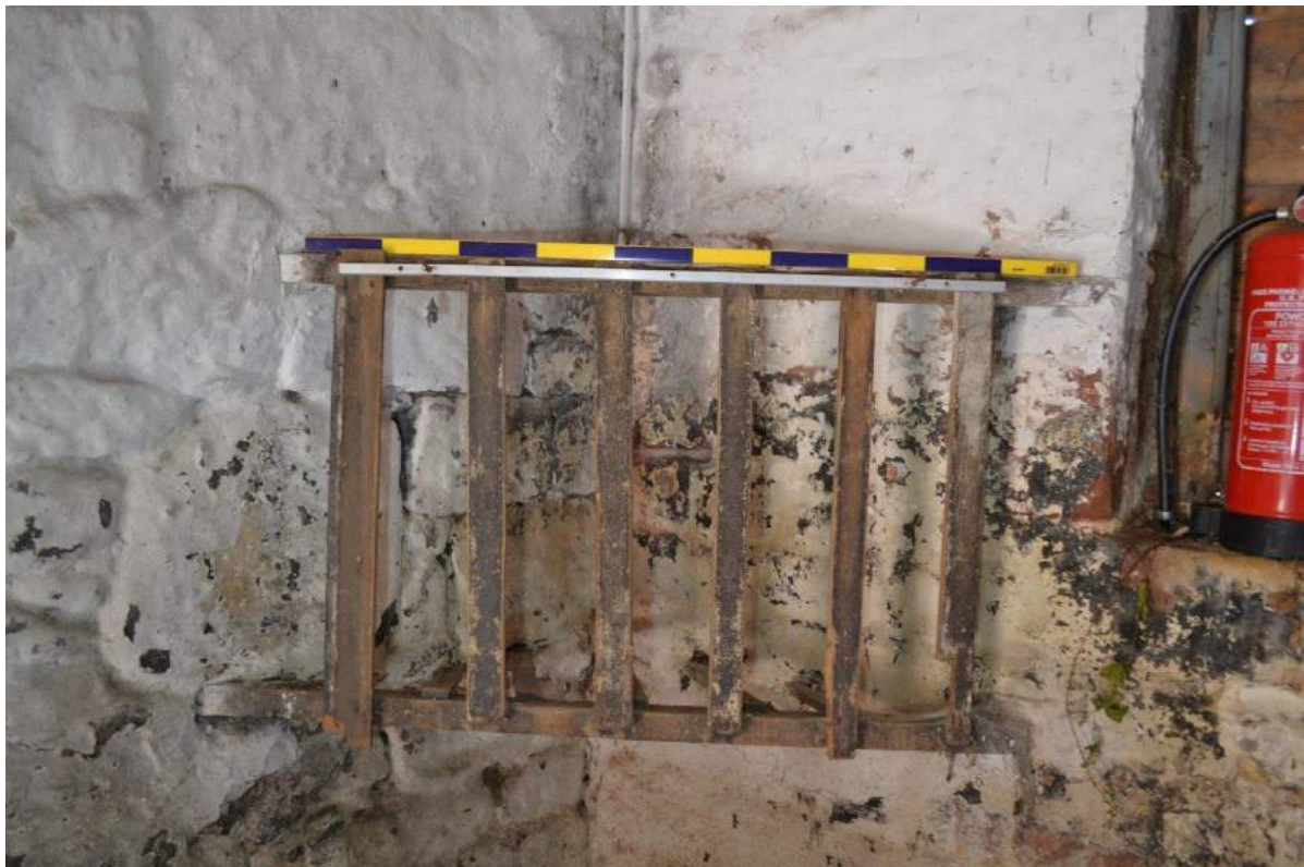
Plate 47: Stable ground floor, hay rack in corner formed by dividing wall to workshop and north-facing flank wall. Scale = 1m
