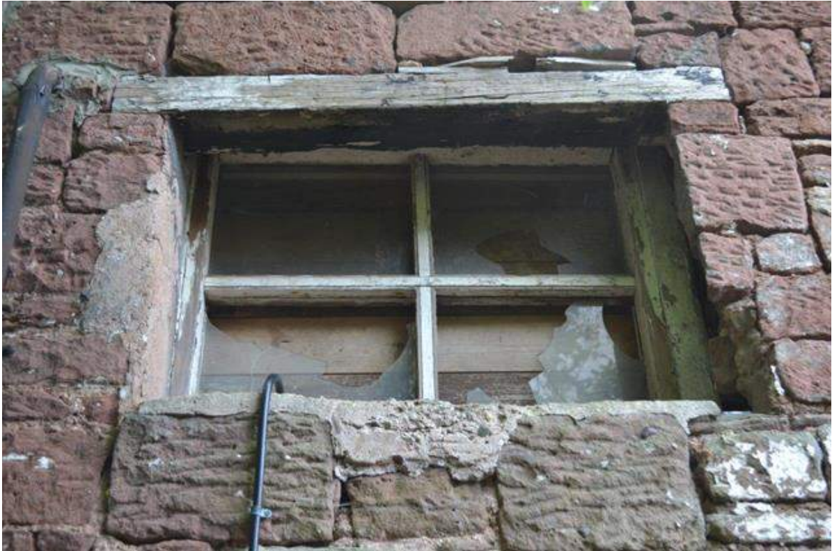
Plate 40: Sightline to the first floor widow opening in the north-facing elevation of the stable, with timber lintel, no sill, timber window frame and broken glazing.
