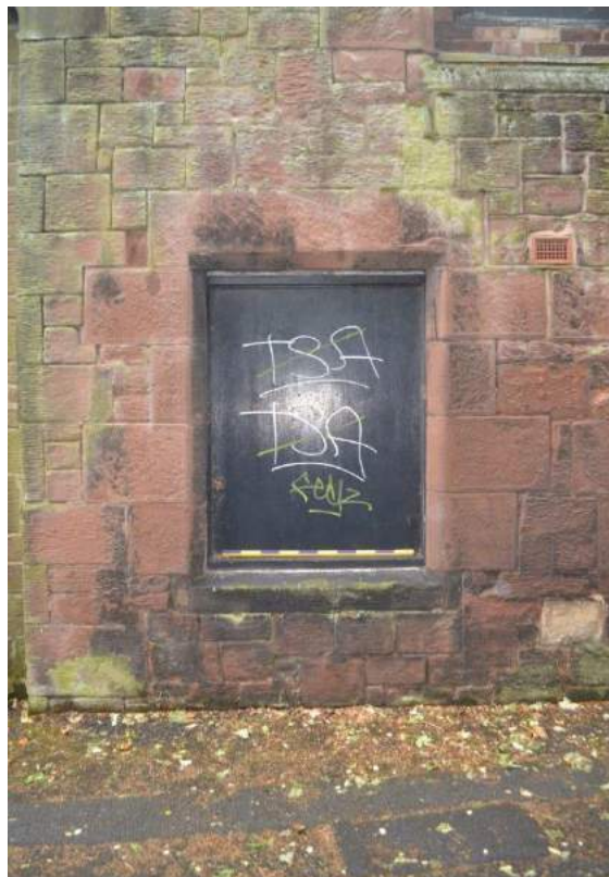
Plate: 34 Detail of boarded left-hand ground floor window with chamfered broached ashlar dressings.
