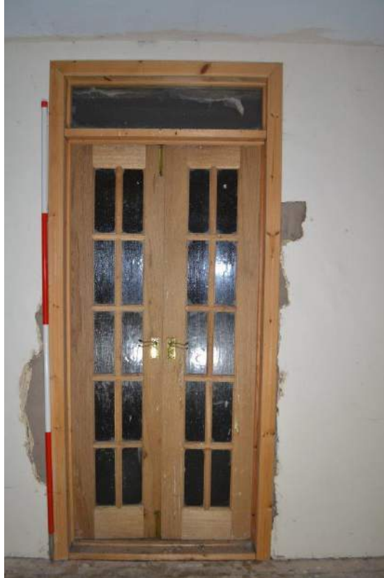
Plate 56: Stable first floor, detail of the porte-fenêtre into the mezzanine floor in the barn
