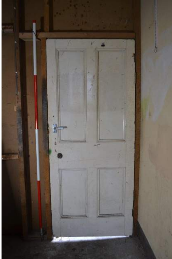
Plate 74: Ground floor, Workshop showing the partition wall and four panel, raised and fielded timber door.
