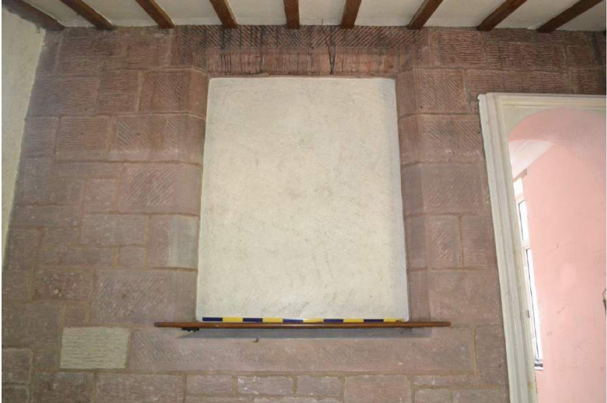
Plate 115: Sightline to the interior of the Store showing the stone-wall which was the ground floor portion of the gable end to the north-facing elevation of the western wing of the farmhouse. Blocked window with chamfered and broached stone dressings.
