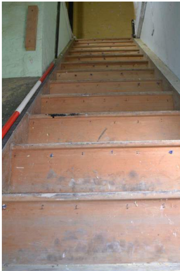
Plate 77: Ground floor, Workshop, timber stair case providing access to the first floor. There are 14 steps in the stair case. The rise is 20.cm and the tread width (with nosing) is 24.5cm
