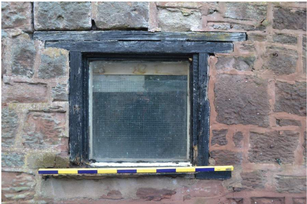
Plate 64: Detail of window opening in west-facing gable elevation of the workshop. Lintel formed from two planks with upper, longer than lower. Timber jambs.
