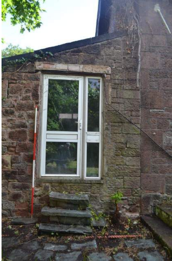
Plate 112: Sightline to the west showing the stone-built west-facing elevation of the Store. Shows, doorway in the Store providing access the garden with uPVC door and margin fenestration and butt-joint with the north-facing gable elevation of the western wing of the Farmhouse.
