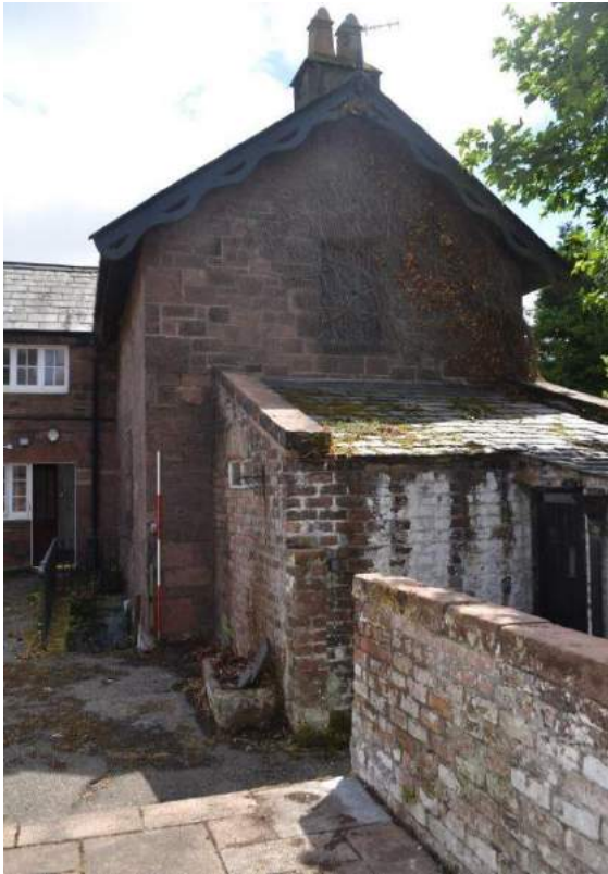
Plate 107: Sightline to the south from the eastern bay of the pigsty towards the brick-built, north-facing and west-facing elevations of the Store showing the mono-pitch roof and verge coping.
