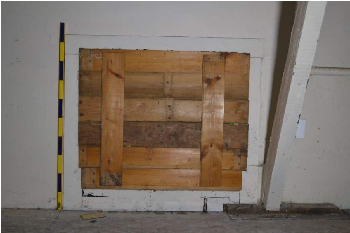
Plate 55: Stable first floor, detail of boarded window in the north-facing flank wall. Possible pitching eye, but unusual in that it does not face the yard and does make sense with respect to the building which onve ran along this north-facing elevation. Scale = 1m
