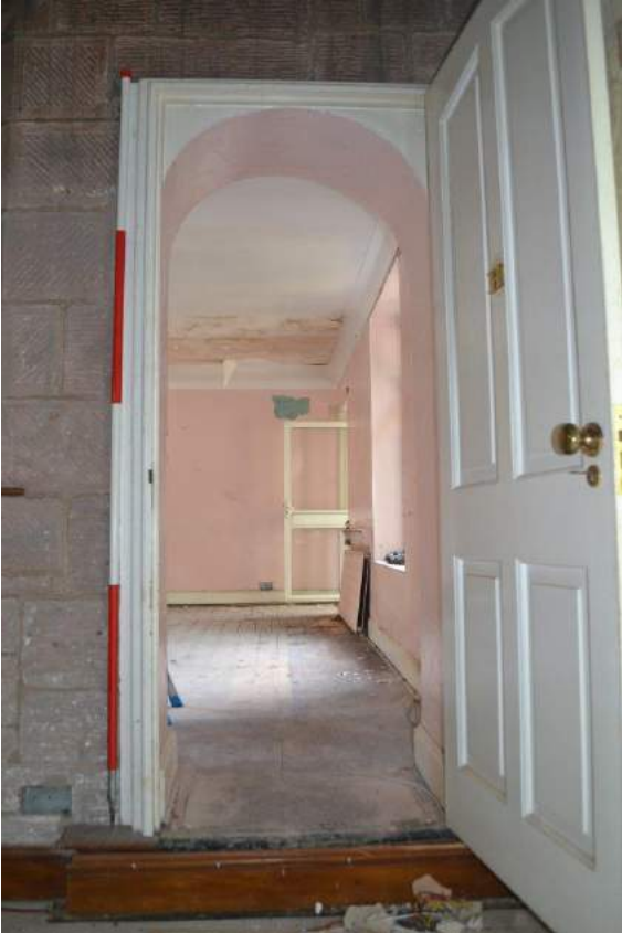
Plate 116: Sightline to the interior of the Store showing the doorway inserted into the ground floor portion of the gable end to the north-facing elevation of the western wing of the farmhouse.
