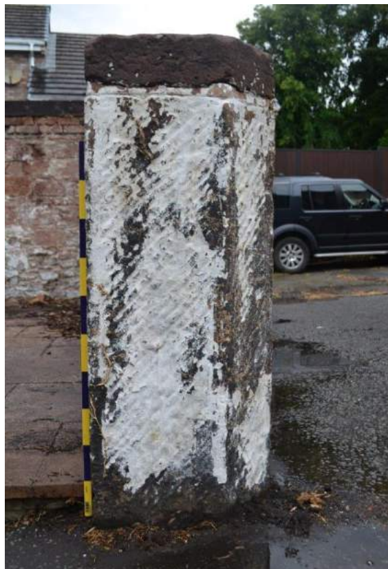
Plate 98: Sightline to the north, showing the broached, chamfered stone pillar at the southern terminal of the south-facing elevation of the pigsty. Scale = 1m
