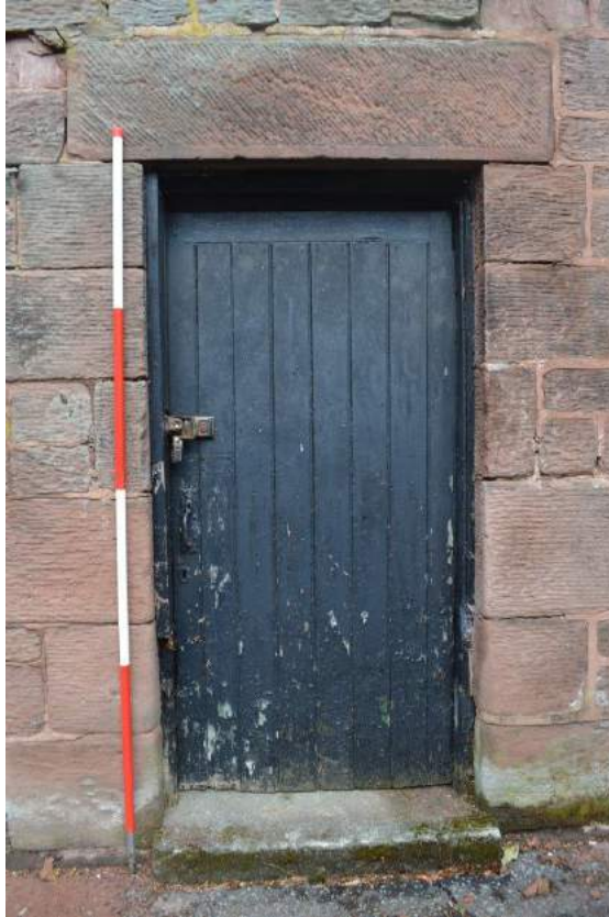
Plate 69: Sightline to the north to the south-facing elevation of the workshop showing detail of the ground floor door showing massive lintel, broached ashlar dressings and step up from the farmyard surface.
