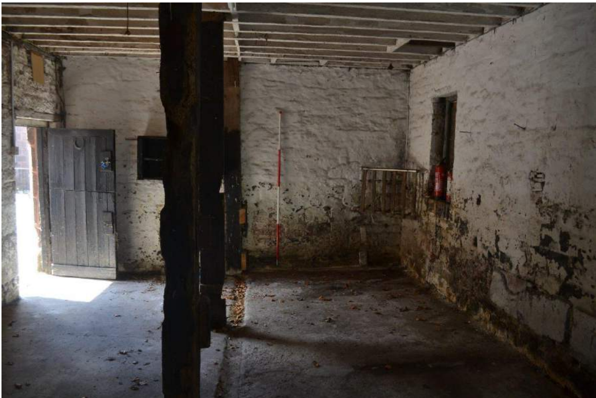
Plate 45: Sightline within the ground floor of the stable towards the wall dividing the stable from the workshop. Showing the concrete floor, the two posts defining the stalls, the corner hay rack, the joists supporting the first floor and the channel in the floor to direct urine etc. to the drain.
