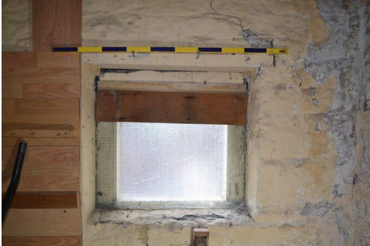
Plate 76: Ground floor, Workshop, showing the case and glazing of the window opening in the east-facing elevation. Scale = 1m
