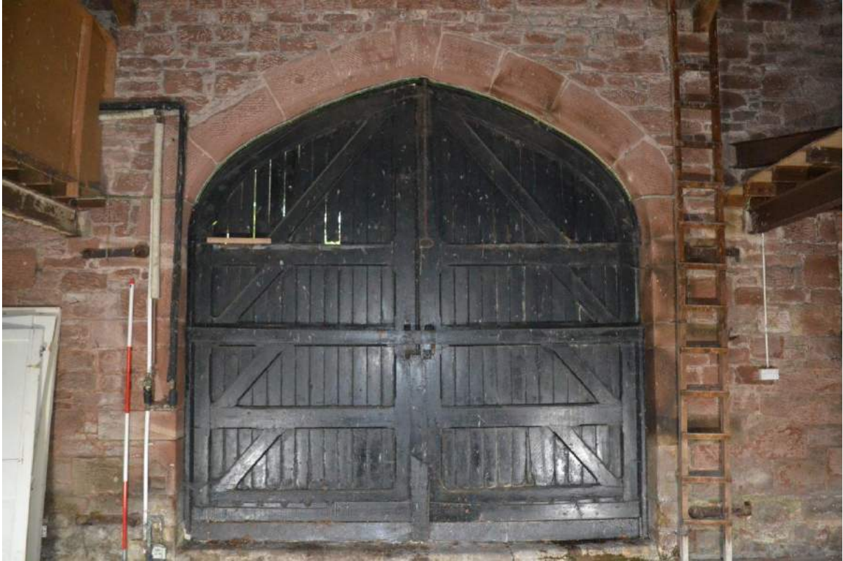
Plate 18: Inside details of the cart-entrance door construction (frame, ledges and straight braces) in the east-facing elevation.
