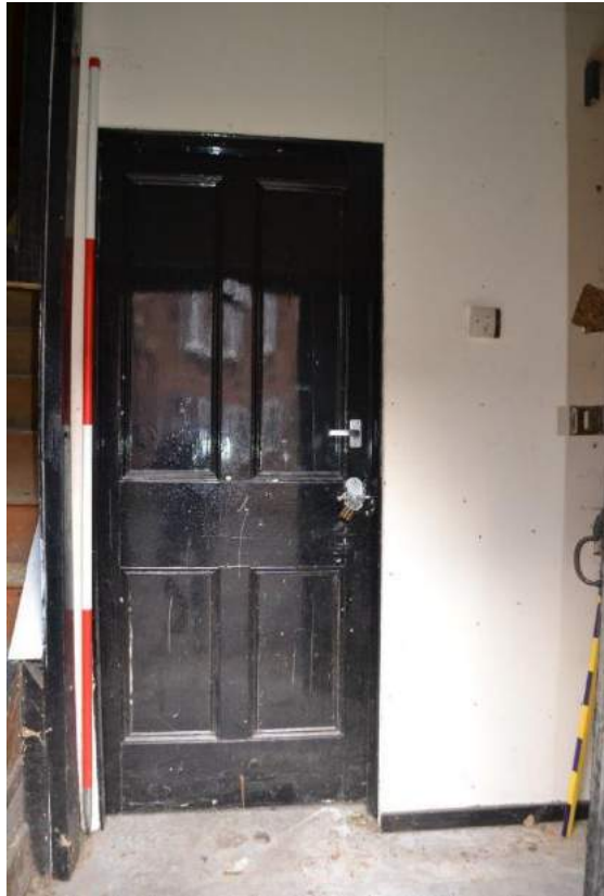
Plate 70: Sightline into the Workshop, ground floor showing the partition wall and four panel, raised and fielded timber door.
