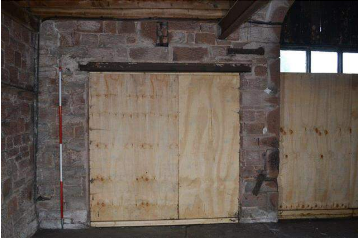
Plate 21: The inserted doorway in the elevation opening onto the farmyard (east-facing) showing rolled steel joist lintel
