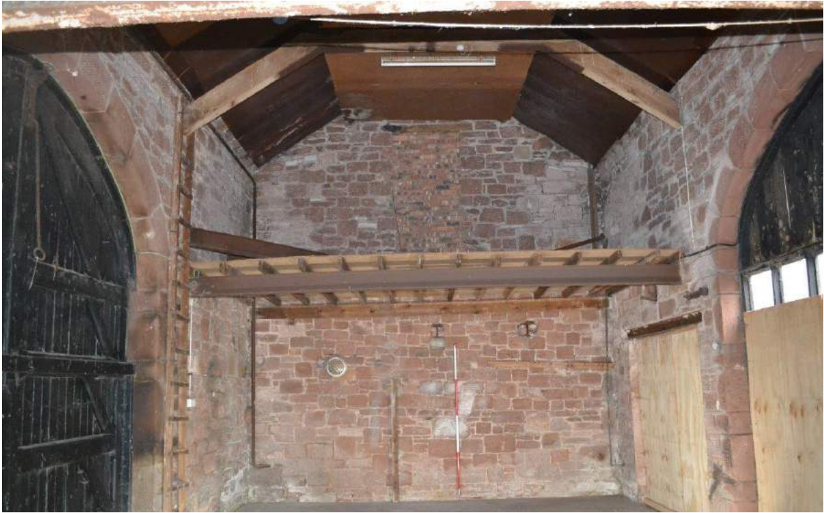
Plate 16: Sightline to the southern wall, showing inserted mezzanine floor on longitudinal joists in turn supported on a timber beam attached to the wall and a rolled steel joist the ends of which have been inserted into the wall of the east-facing elevation. Also shows ladder access and infilled doorway at first floor level into the wing of the farmhouse
