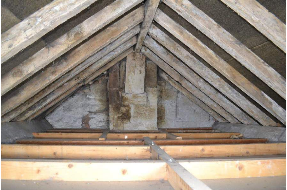
Plate 86: Roof space, Workshop, recently inserted ceiling joists fixed to canted purlins, with long and short header-joists (noggings), the shorter ones trimmed to get around the chimney breast. Common rafters fixed to ridge beam. The underlayment suggests the roof was reconstructed, possibly in the late 20 th century. The material composition was not examined – possibly asphalt-saturated felt, rubberized asphalt; or non-bitumen synthetic felt. Chimney breast on west-facing gable elevation.
