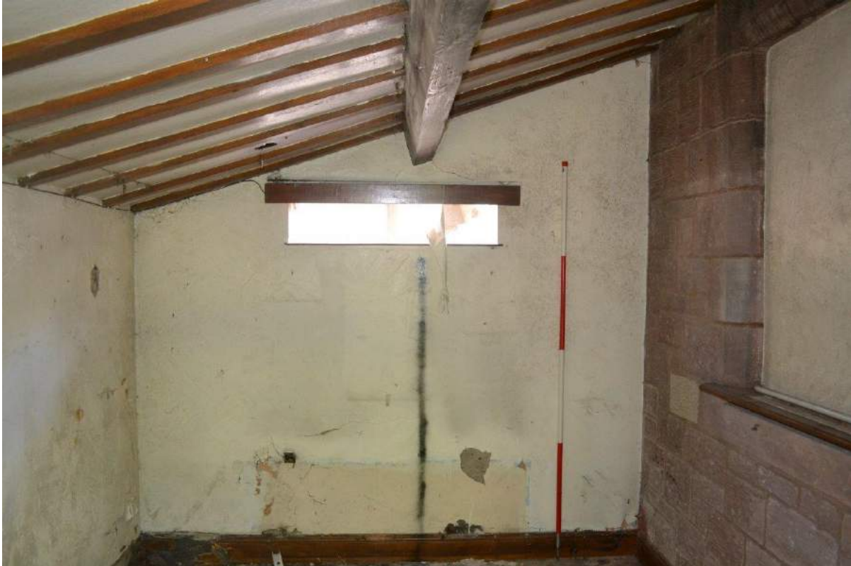
Plate 113: Store, interior, sightline to the inside face of the east-facing elevation showing plastered wall and window. Common rafters and canted purlin forming mono-pitch roof structure.
