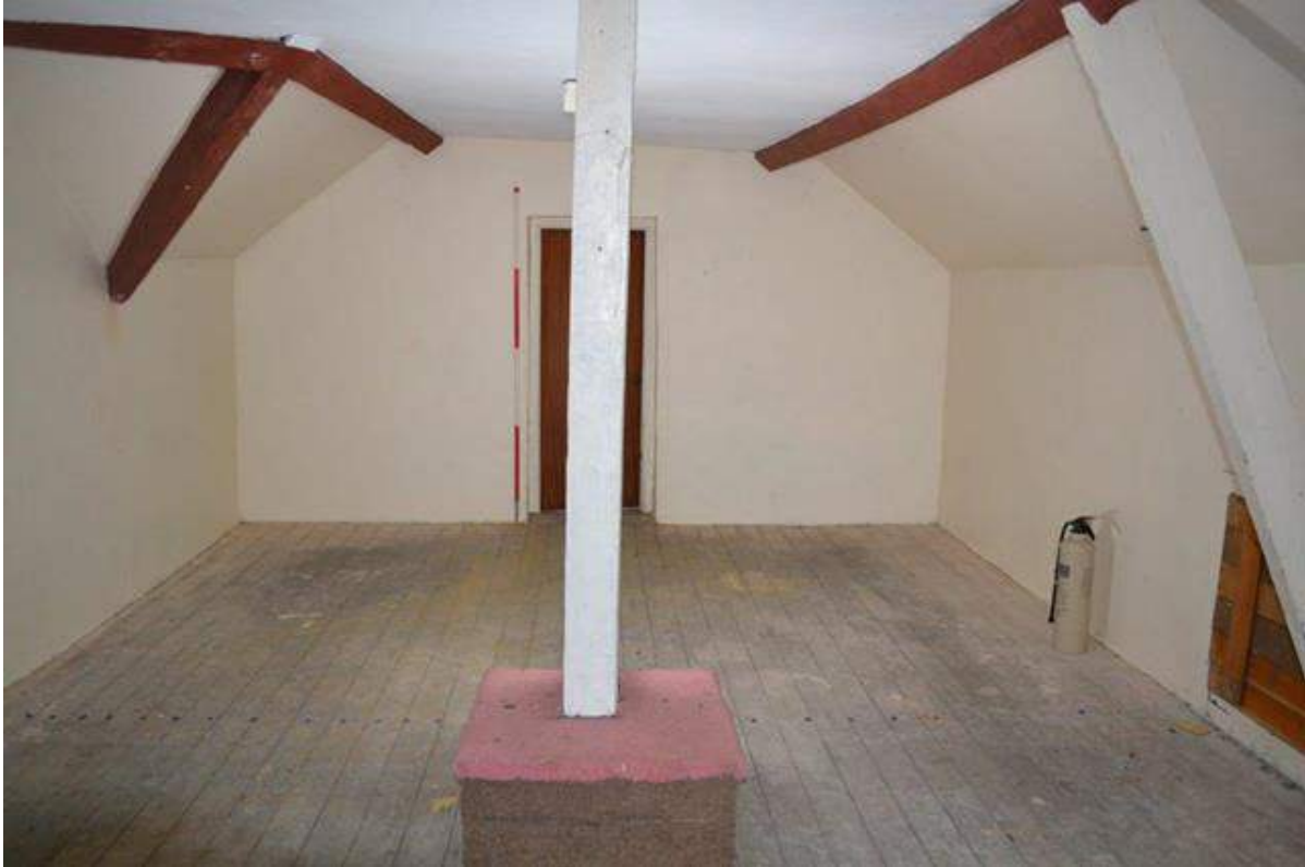
Plate 54: Stable first floor, sightline to the door in the party wall with the first floor of the workshop showing the valley rafter, jack rafters and purlin supported on a notched brace. Also shows a post extending into the roof space.
