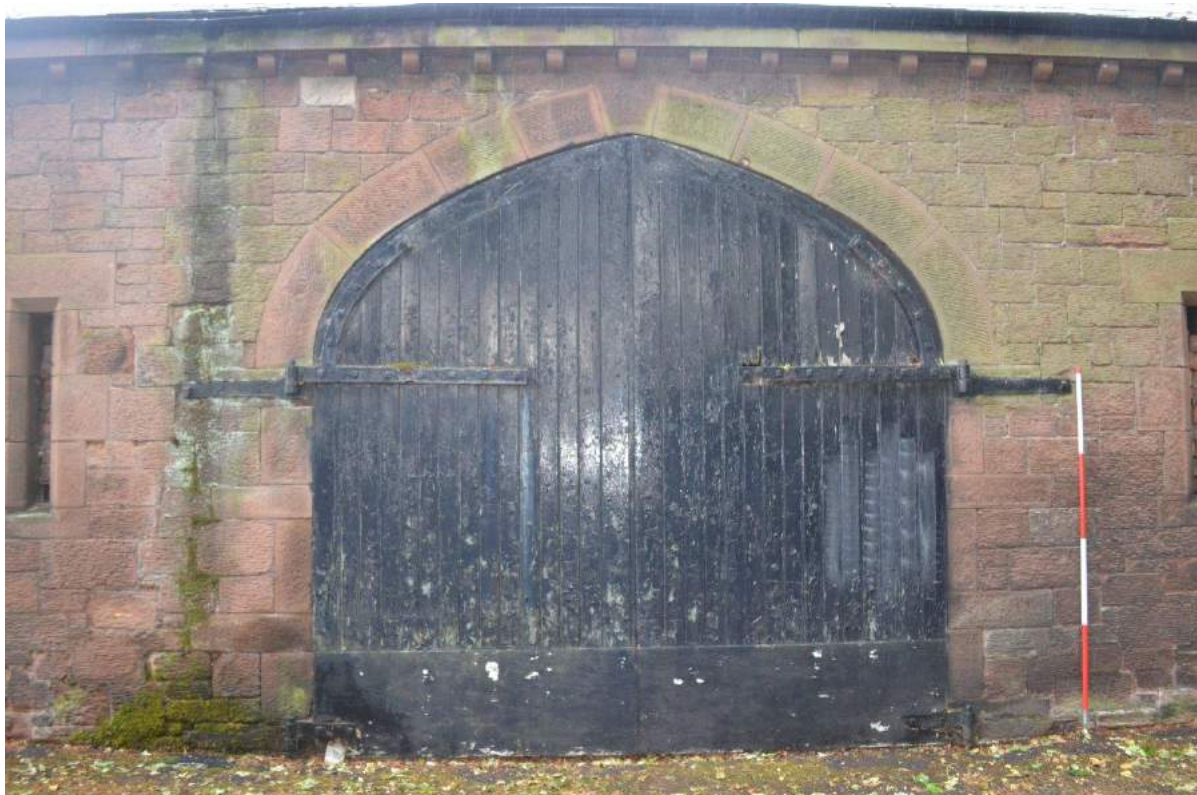
Plate 8: Detail of cart-entrance door showing hinges to exterior comprising carcass leaf and door leaf with knuckle and pintle. The door leaf is in two parts, with a secondary leaf arcing up and along the stile
