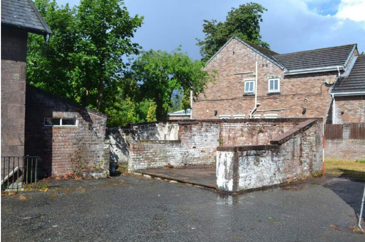
Plate 89: Sightline to the north-west to the pigsty from the farmyard. It is notable that the dividing brick-built wall between the original second and third stalls survives, but the other two dividing walls do not. The roofing arrangement was probably a mono-pitch roof terminating to provide a small, open exercise yard the front wall to which (which probably contained access doors and feeding chutes) is no longer present.
