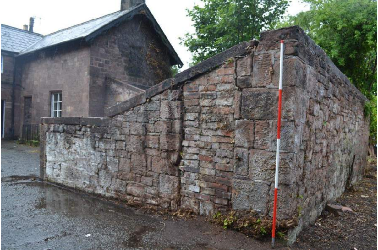
Plate 91: Sightline to the south-west from the access track towards the east-facing elevation of the pigsty (with blocked up doorway)
