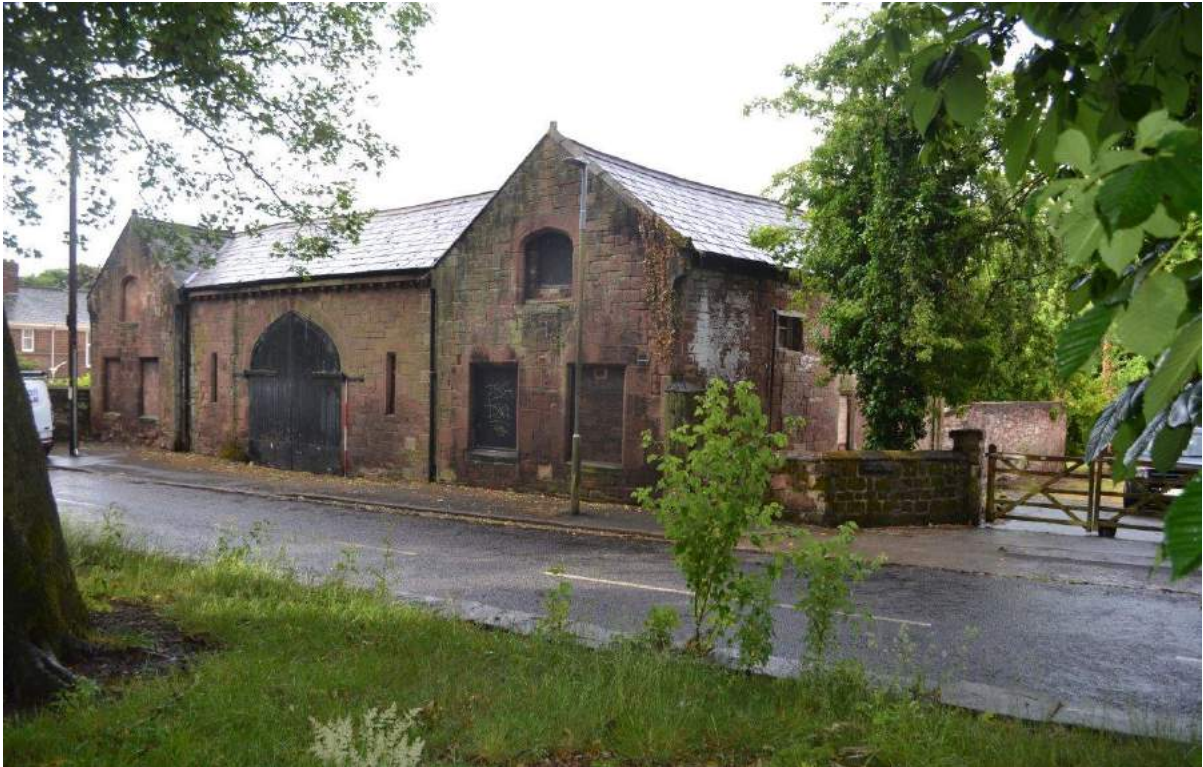
Plate 4: Sightline to the south showing the east-facing elevation of (from left to right) the east-facing gable elevation of the farmhouse (with three blind windows), the barn with its cart-entrance doors and two arrow-slit vents and the east-facing gable elevation of the stable with its blind window and boarded-up windows. Boundary wall, driveway pocket, gatepost and wooden gates to right.
