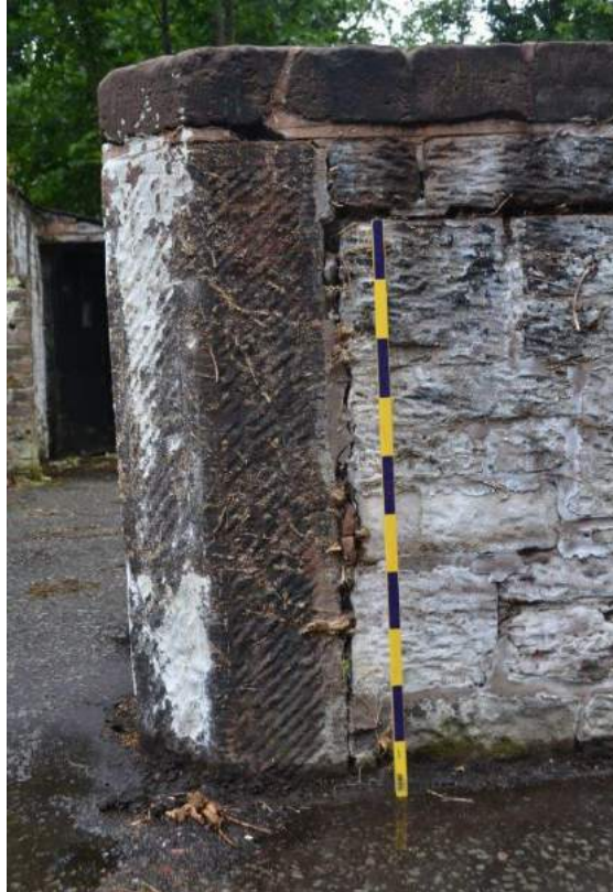
Plate 97: Sightline to the south, showing the broached, chamfered stone pillar at the southern terminal of the east-facing elevation of the pigsty. Scale = 1m
