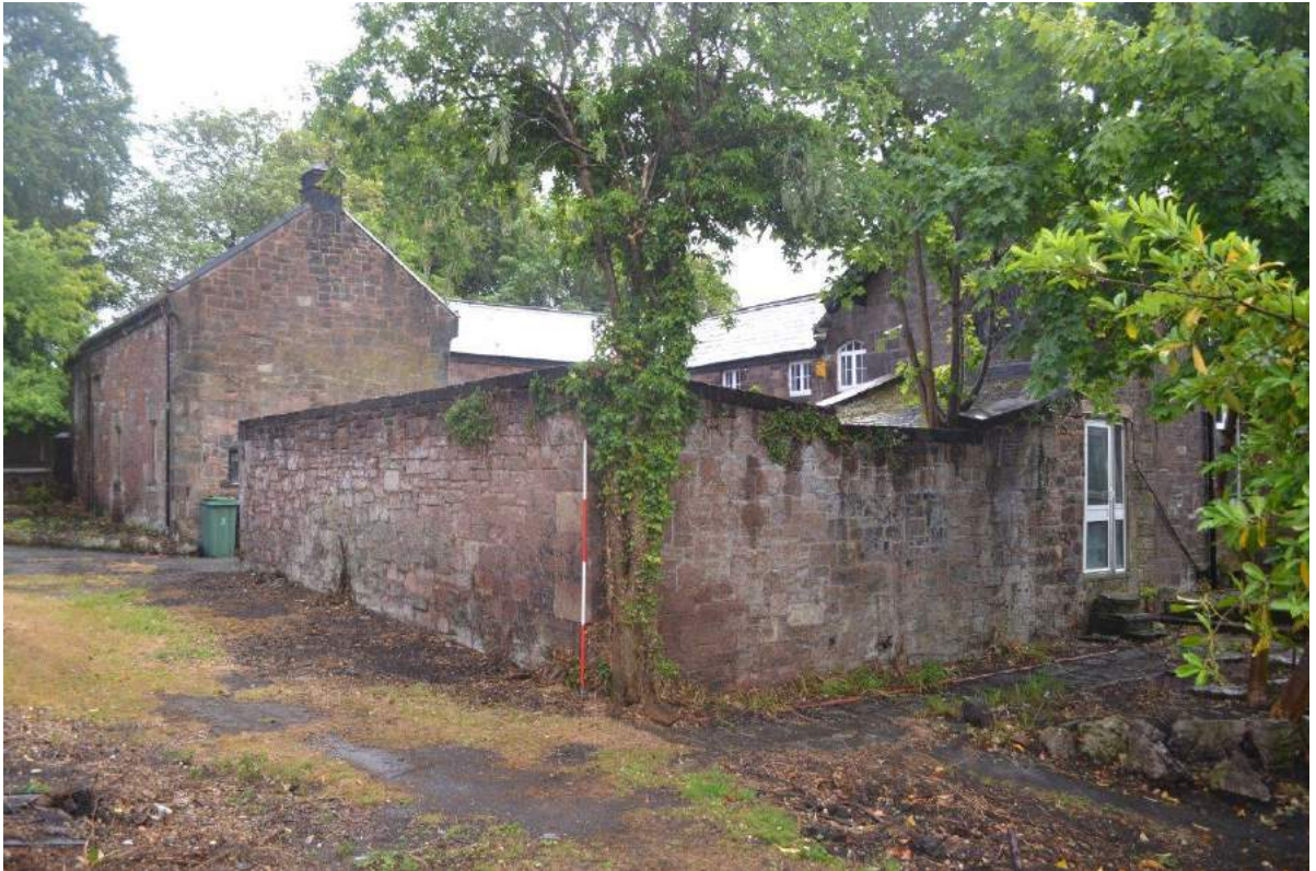
Plate 92: Sightline looking south-east towards the north-facing and west-facing elevations of the pigsty
