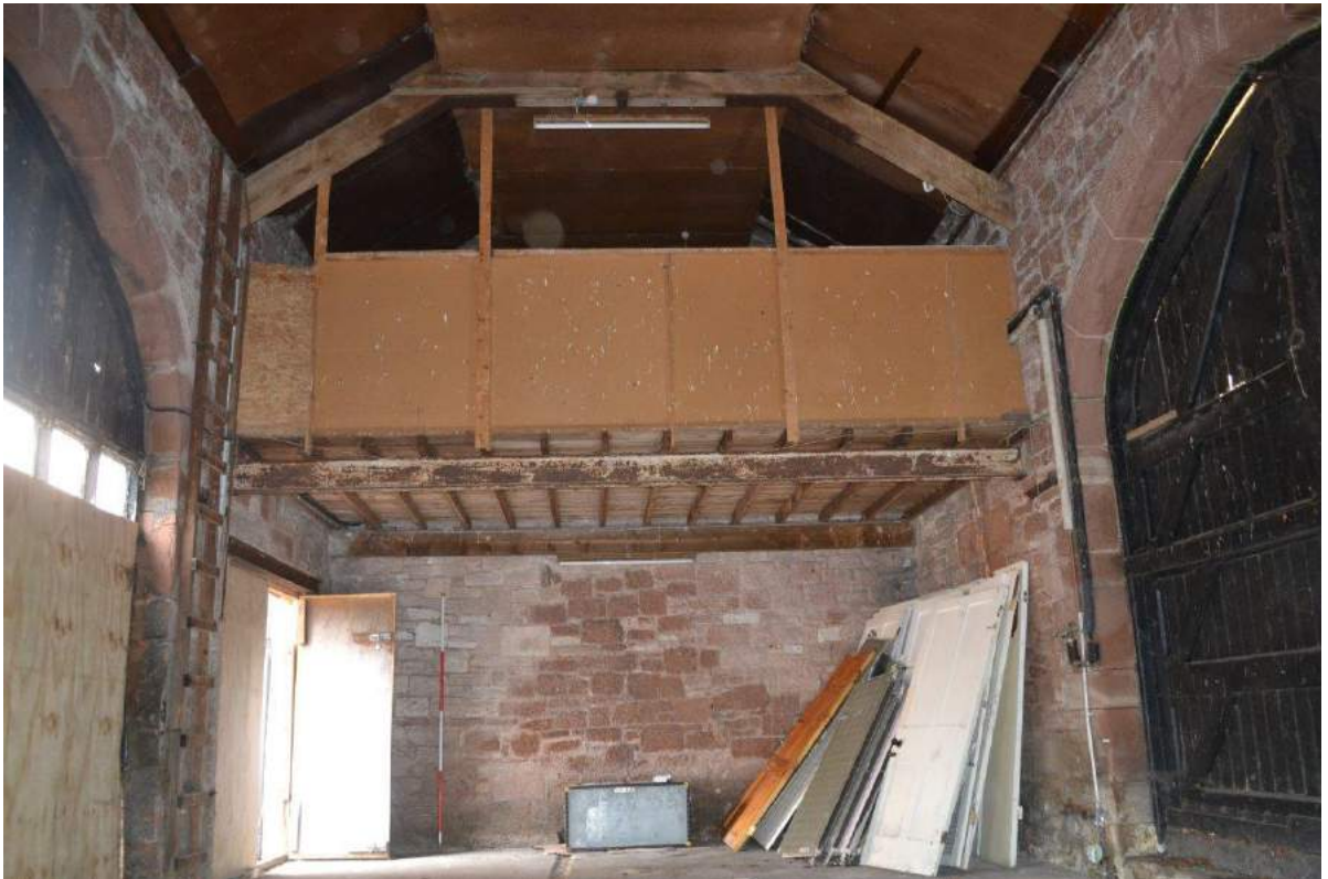
Plate 17: Sightline to the northern wall, showing inserted mezzanine floor on longitudinal joists in turn supported on a timber beam attached to the wall and a rolled steel joist the ends of which have been inserted into the west-facing east-facing walls. Also shows ladder access.
