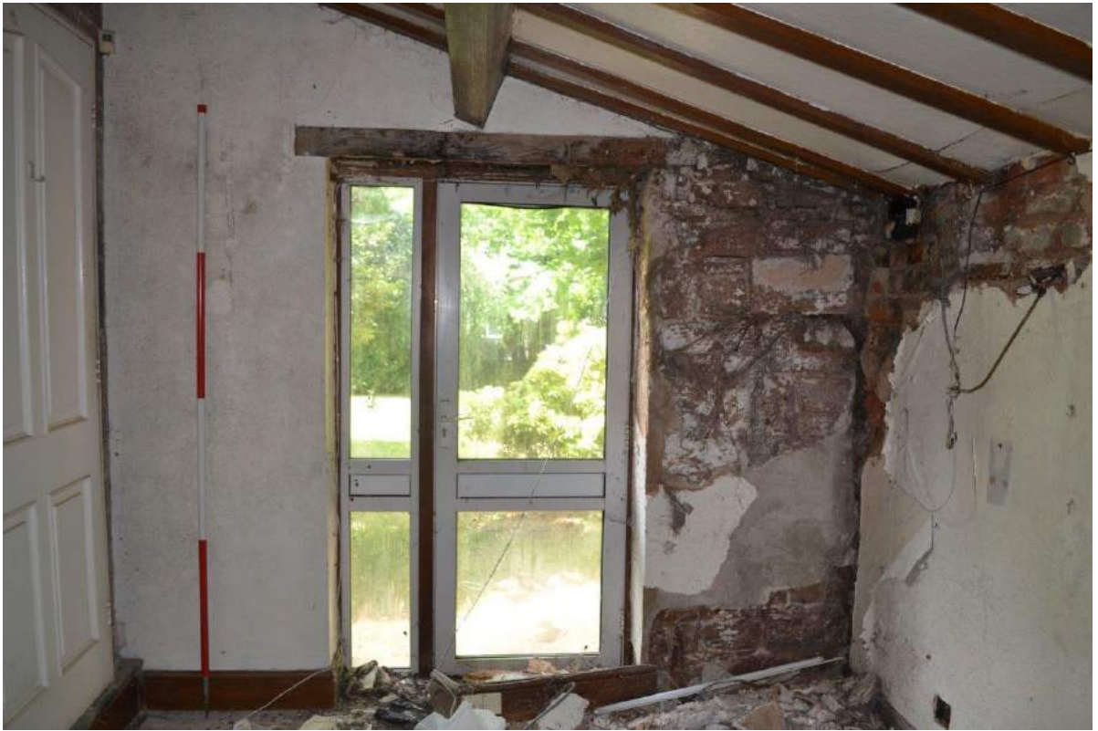
Plate 114: Store, interior, sightline to the interior of the west-facing elevation showing the uPVC door into the garden
