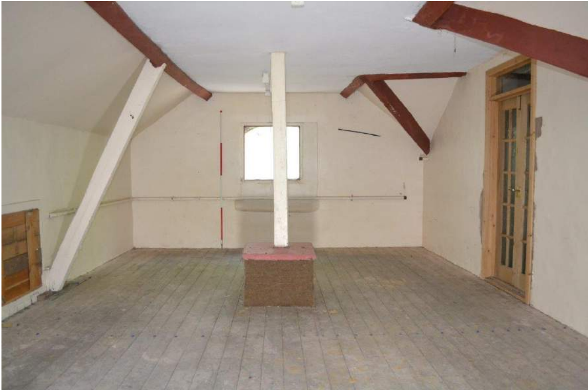
Plate 51: Stable first floor, sightline towards the east-facing gable elevation showing the partially stopped-up window opening, the valley rafter, jack rafters and canted purlin supported on a notched brace, Also shows the porte-fenêtre into the mezzanine floor in the barn and a post extending into the roof space.
