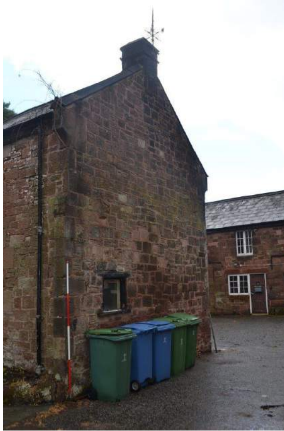
Plate 59: Sightline to the south-east showing oblique view of the north-facing gable elevation. Highlights capped chimney-in-gable-wall, coping-at-gable, projecting corbelled gable skew and window opening to ground floor gable elevation.
