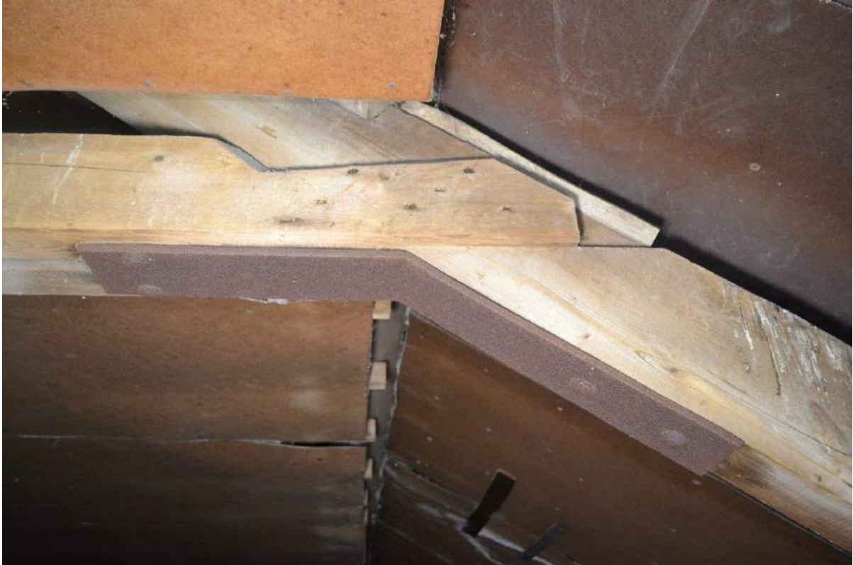
Plate 28: Detail of the arrangement in the roof truss between the principal rafter, the ledger strip on the raised tie beam and the pinned iron plate supporting both members.
