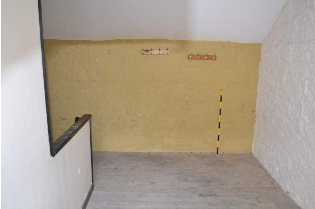
Plate 84: First floor, Workshop, sightline to the inside face of the north-facing elevation. Scale = 1m.
