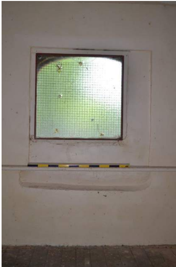
Plate 52: Stable first floor, detail of partially stopped-up window opening with security glass in a wooden frame.
