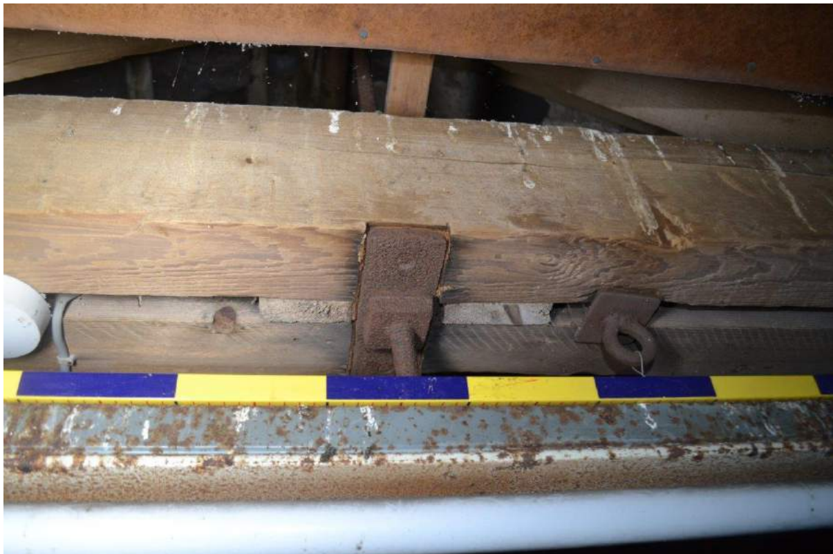
Plate 27: Detail of the king rod engagement with the raised tie beam (scale = 1m). The plate is recessed in a rebate cut into the tie-beam and secured by means of a nut on the threaded terminal of the rod.
