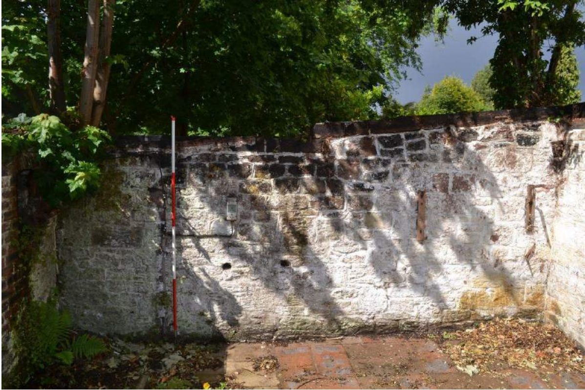
Plate 103: Sightline towards the interior side of the west-facing elevation, the first stall.
