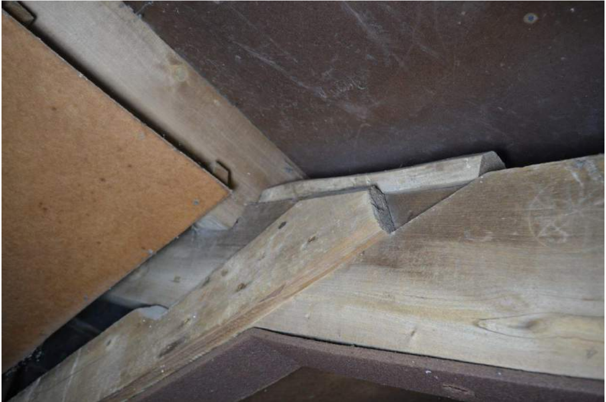
Plate 29: Alternative view of the detail of the arrangement in the roof truss between the principal rafter, the ledger strip on the raised tie beam and the pinned iron plate supporting both members. The trenced purlin is located by means of a cleat.
