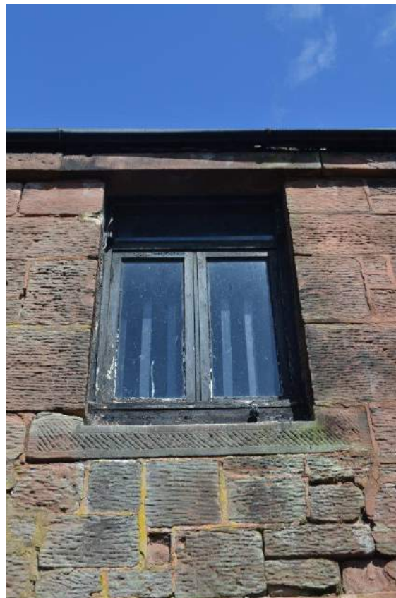
Plate 68: Sightline to the north to the south-facing elevation of the workshop showing detail of the first floor casement timber window with fixed light above, chamfered , broached sill and lintel formed by the finely dressed fascia
