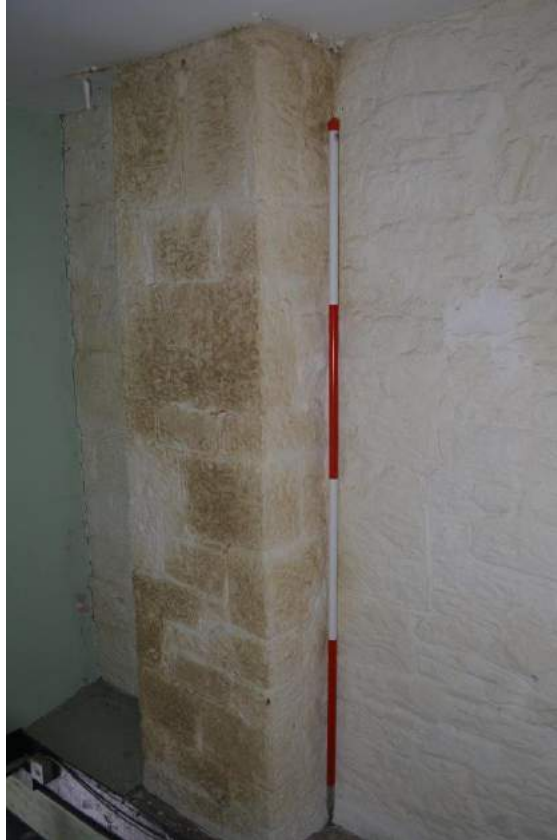
Plate 80: First floor, Workshop, view of the chimney breast, projecting inwards from the east-facing elevation. The chimney breast is 60cm wide and 28cm deep
