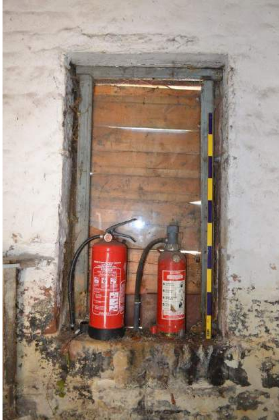
Plate 46: Stable ground floor, detail of boarded window opening in the north-facing flank wall. Timber lintel, timber frame and no sill. Scale = 1m
