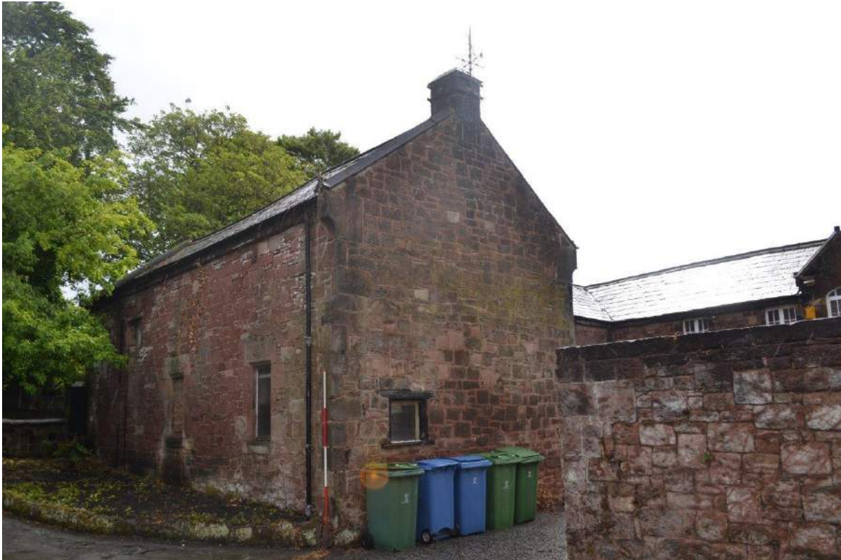
Plate 58: Sightline to the south-east showing oblique views of the north-facing elevation and west-facing gable elevation. Highlights capped chimney-in-gable-wall, coping-at-gable, dressed fascia, projecting corbelled gable skew and window opening to ground floor gable elevation.
