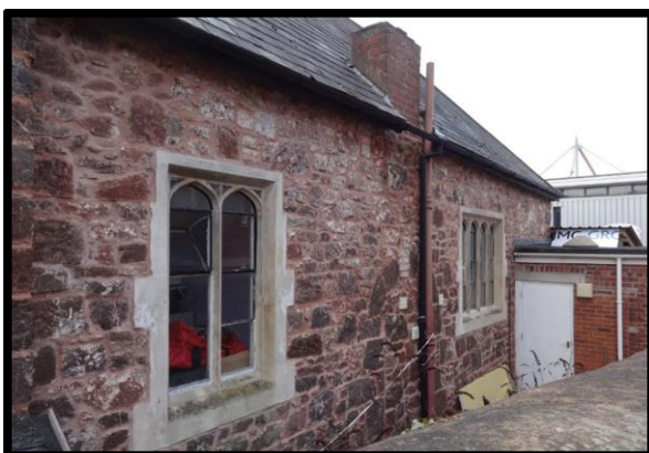
Fig. 17 Rear elevation of the Girls' Schoolroom, showing a blocked doorway to the yard and secondary chimney over it.
