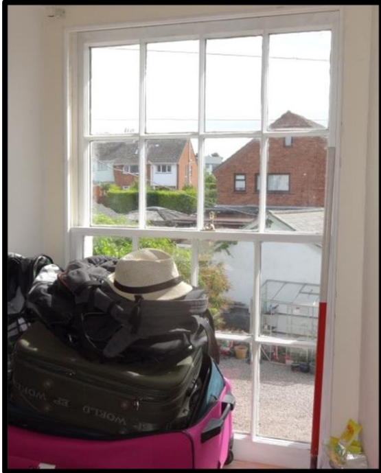
Fig. 11 Detail of the early 19th-century sash in the bedroom on the east side of the house, showing narrow glazing bars with typical mouldings of c.1800.
