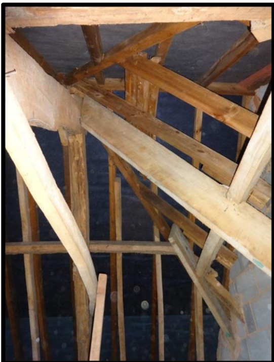
Fig. 16 Detail of the hipped gable at the north end of the house showing the original roof structure overlaid by later roof timbers.
