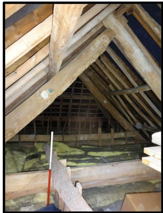
Fig. 17 View within the roof space showing the form of the trusses, and parts of partitions or timber 'stiffeners' protruding in to the roof space.
