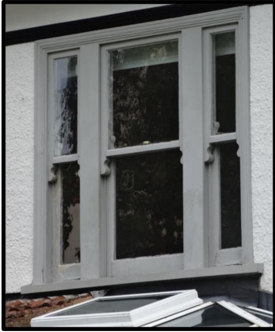
Fig. 6 Detail of the late 19th-century tripartite sashes in No. 2 Harringcourt House, possibly dating from the alterations of 1892.
