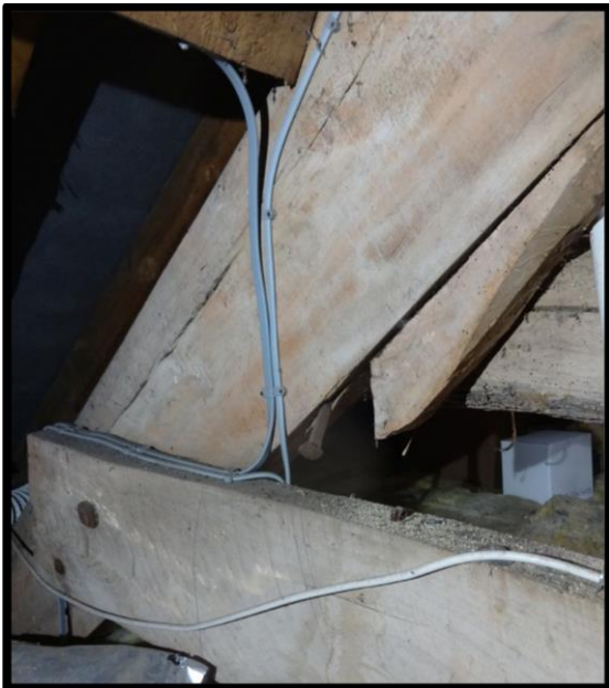
Fig. 19 Detail of the eastern foot of Truss III showing a timber cleat or wedge applied to the underside of the truss which may have related to a vertical post, now removed.
