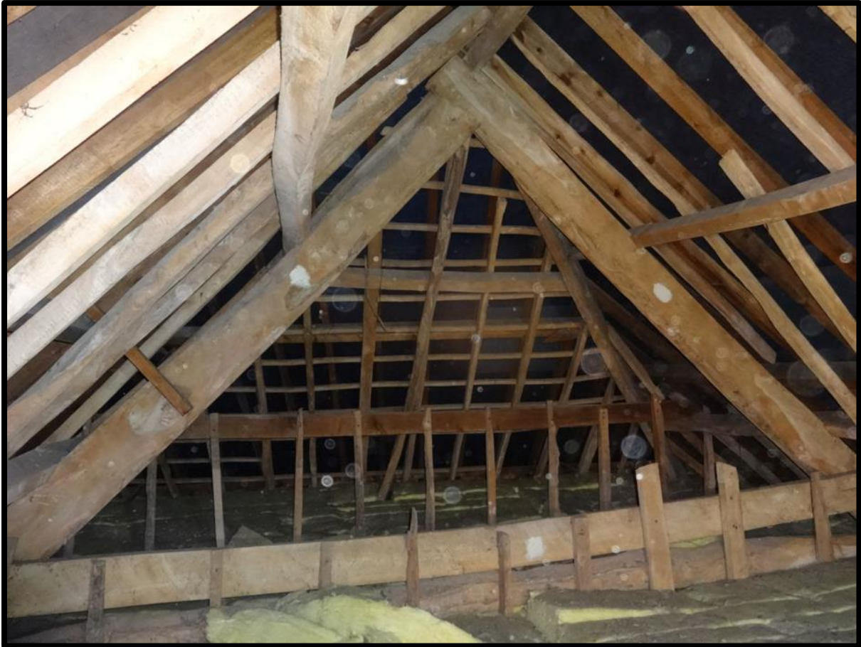
Fig. 18 Detail of the southern end of the roof showing Truss I, the remaining battens beyond and a possible partition protruding within the roof space.
