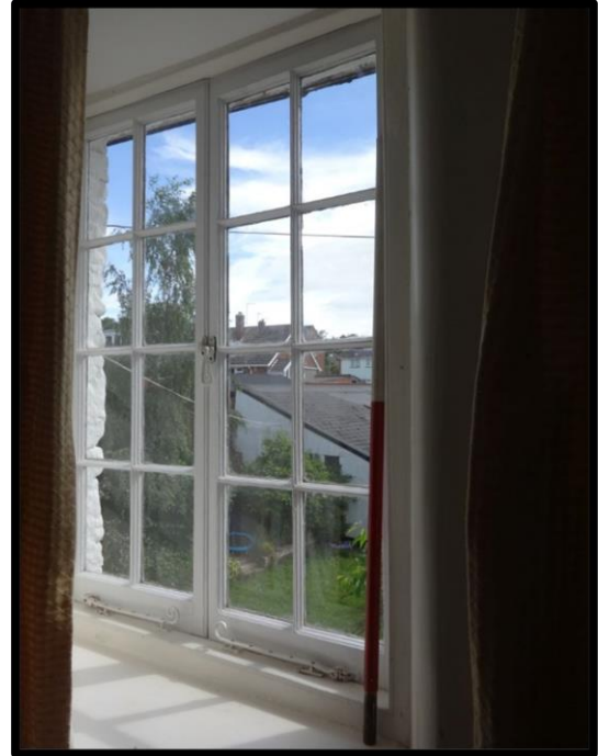
Fig. 12 The early 19th-century casement window in the north bedroom, with similar narrow glazing bars and 20th-century window furniture.
