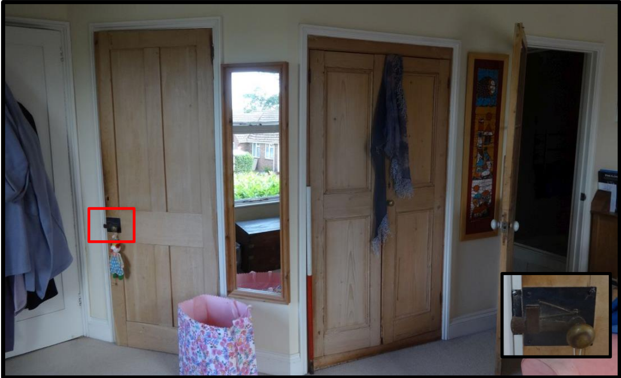
Fig. 15 View of the cupboards in the southern first-floor bedroom showing, historic doors reused in this position, one of which retains an 18th-century style sprung latch (inset).
