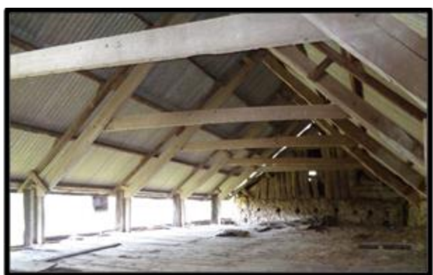
Fig. 34 The interior of the loft of Linhay II looking east, showing the redundant sockets for an earlier first-floor structure in the gable wall.
