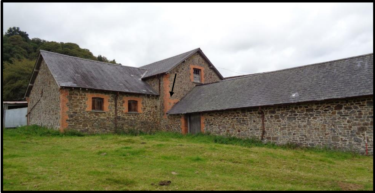
Fig. 19 The south elevation of linhay I (right) showing the differing masonry of the upper section of walling beneath the eaves, the partially blocked opening in the east wall of the threshing barn (arrowed) and the east elevation of the horse-engine house (left).
