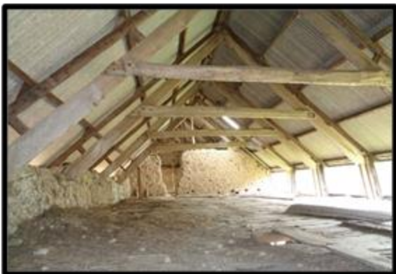
Fig. 33 The first-floor interior of Linhay II, looking west, showing the lapped collars of the roof trusses and the cob walling.
