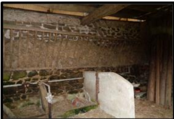
Fig 38 The interior of the north side of the double linhay showing the timber manger below the pitching void and the remains of modern cattle stalls.
