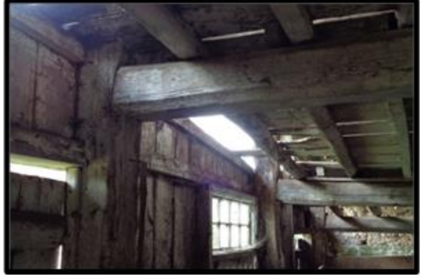
Fig. 32 Detail of the construction of the north front of Linhay II showing the junction of the wall posts and the principal first-floor beams.
