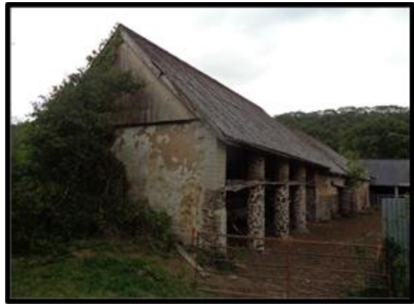
Fig. 37 The western gable of the double linhay III showing possible evidence for a half hip.
