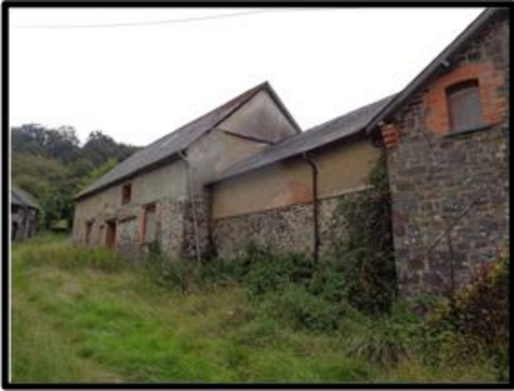
Fig. 46 The south elevation of the stable (left) and poundhouse (Right) from the farmyard.
