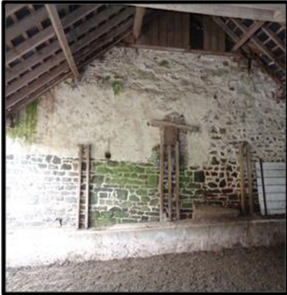
Fig. 28 The interior of the horse engine house showing the traces of beams and openings in the south wall.
