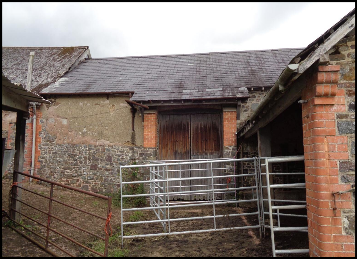
Fig. 24 The south elevation of the threshing barn, showing its relationship with the horse-engine house (right).
