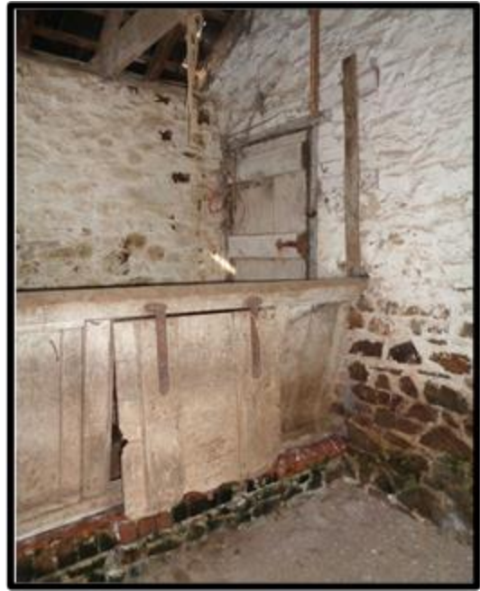
Fig. 57 The interior of the piggeries showing a feeding hatch from the headwalk.
