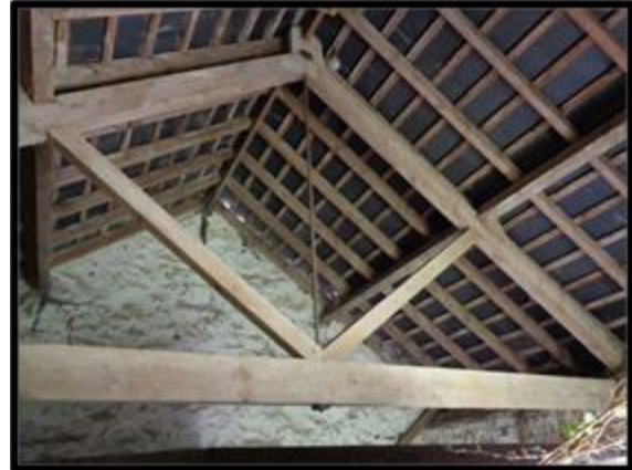
Fig. 17 The trap house roof showing the roof truss with raking struts and suspension rod.
