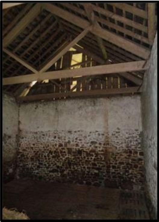
Fig. 25 The interior of the threshing barn, looking west, showing the roof structure.
