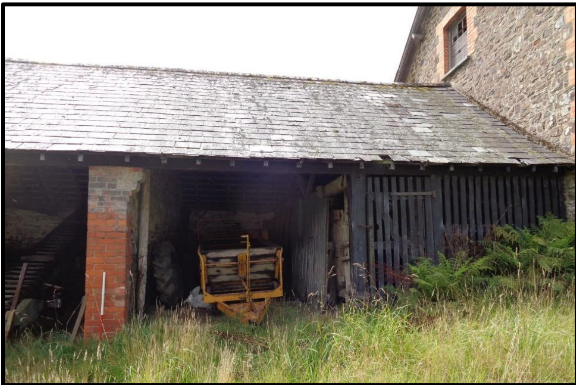
Fig. 20 The north elevation of linhay I showing the brick pier with corbelling marking the original western limit of the building (left) and the ventilation screens to the western bay of the extension (left).
