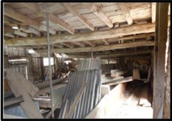
Fig. 31 The interior of Linhay II showing the staggered joists of the first-floor structure.
