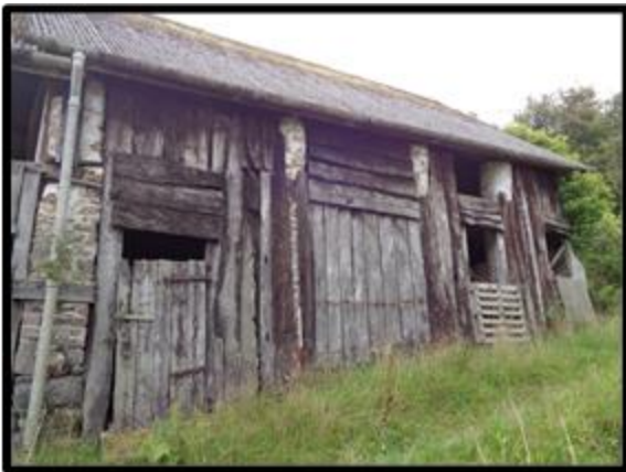
Fig 36 The north front of Linhay III showing later enclosure of the façade.
