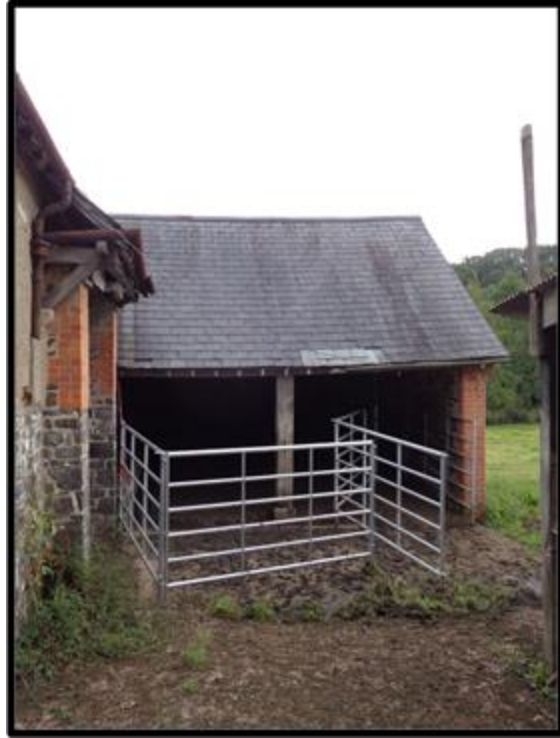
Fig. 26 The west-facing elevation of the horse engine house and the pent roofs over the barn doors.
