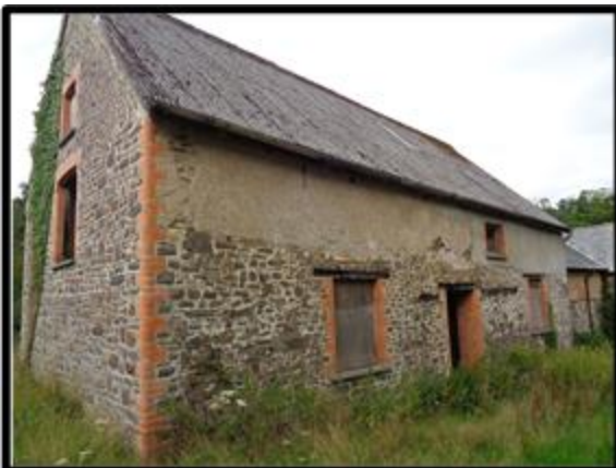
Fig. 50 The south elevation of the stable showing 19th-century red brick repairs to the openings and jambs.
