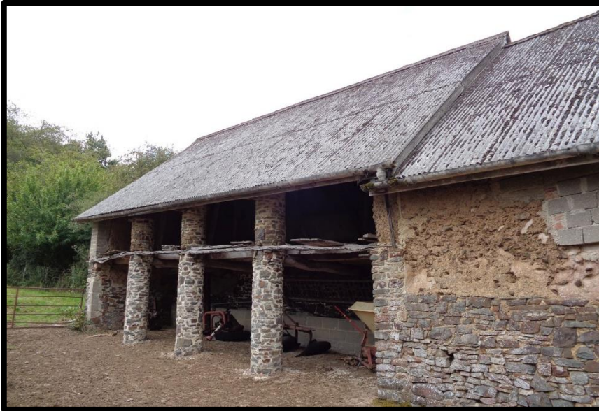
Fig. 35 The south elevation Linhay III, showing the cylindrical piers supporting the first-floor structure and roofs.
