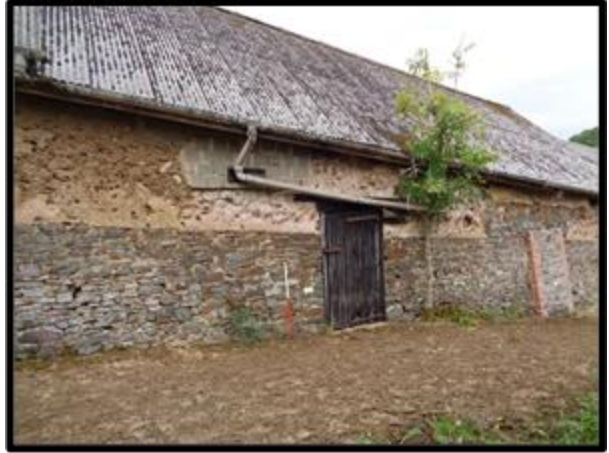
Fig. 30 The south elevation of Linhay II showing the much patched and buttressed rear wall of cob and stone with later buttresses.
