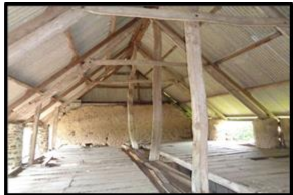
Fig 39 The interior of the first floor of the double linhay showing the single loft with a central pitching void serving both sets of mangers.
