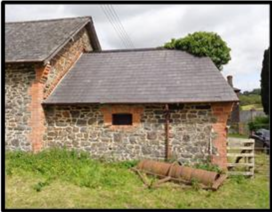
Fig. 16 The south elevation of the trap house, showing the brick weatherings built into the gable of the adjacent linhay.
