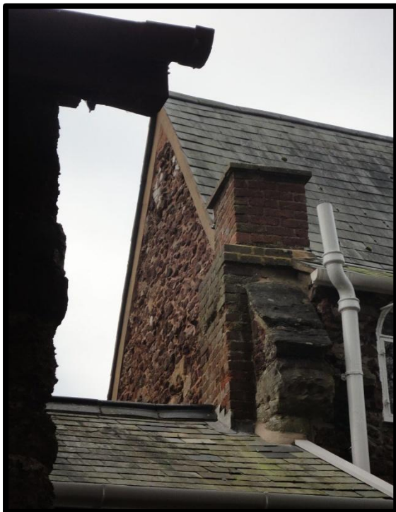
Fig.16 Detail of the eastern corner of the gatehouse showing the remains of a primary coping and decorative kneeler.
