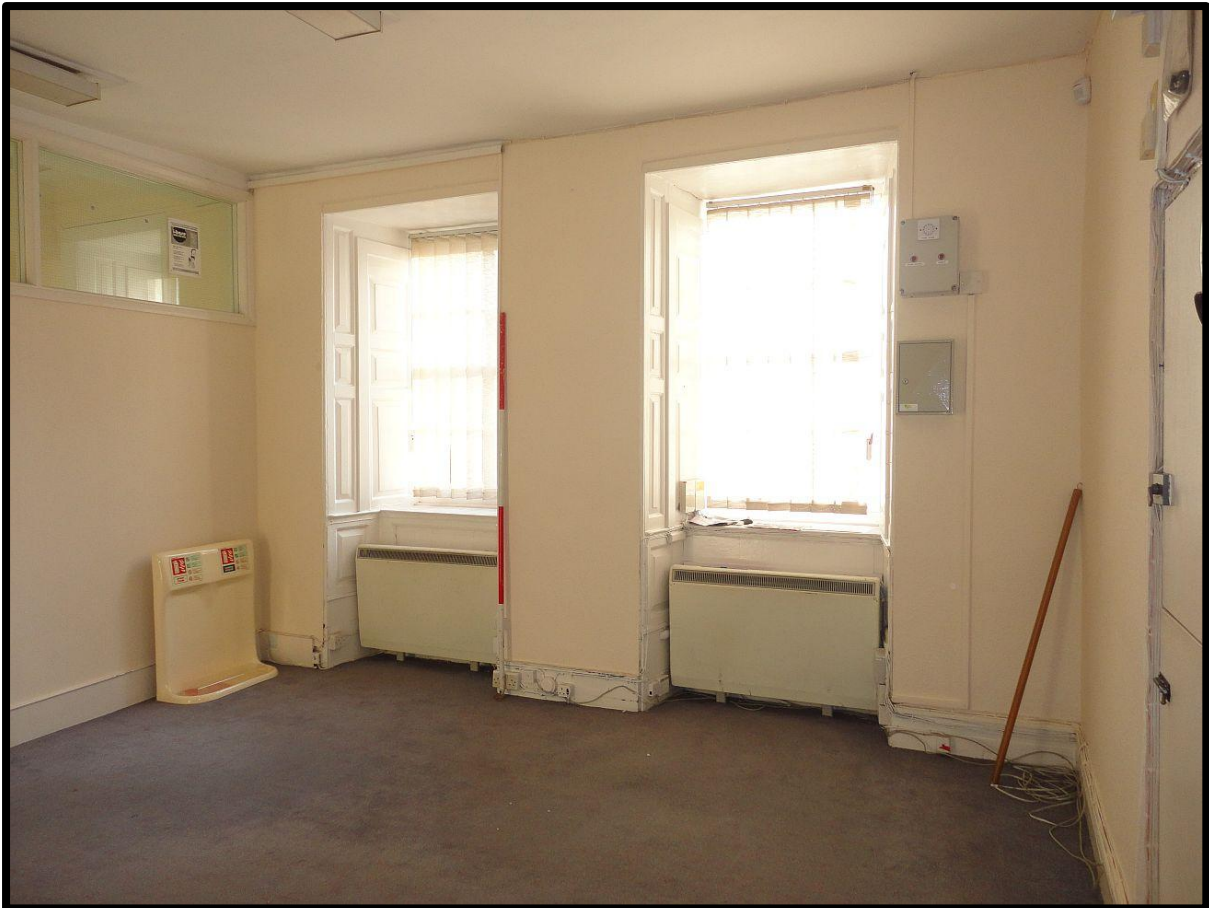
Fig. 22 View of the large ground-floor room to the west of the gate passage showing the extent of the post-medieval and modern alterations, concealing the medieval fabric.
