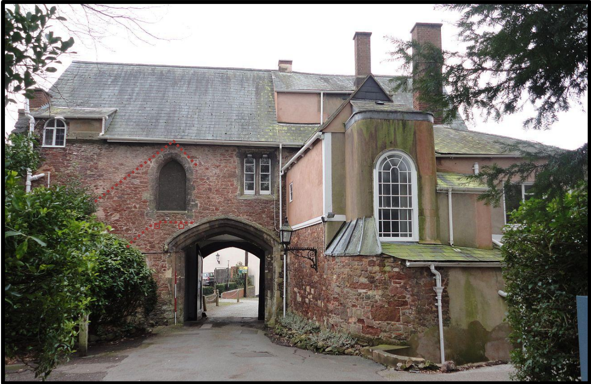
Fig. 15 View of the rear of the gatehouse, showing the first-floor doorway over the arch and the scar of the roof, sockets and string of an external covered staircase serving the principal chambers (dotted). The remains of the wall dividing the great court can be seen projecting from the rear of the gatehouse beyond the 19th-century bracket lamp. This wall was demolished beyond this point and rebuilt as a curved corner in c.1812.
