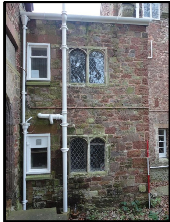
Fig. 21 Elevation of the small square building added at the eastern corner of the building, possibly to provide a replacement for the medieval newel stair.
