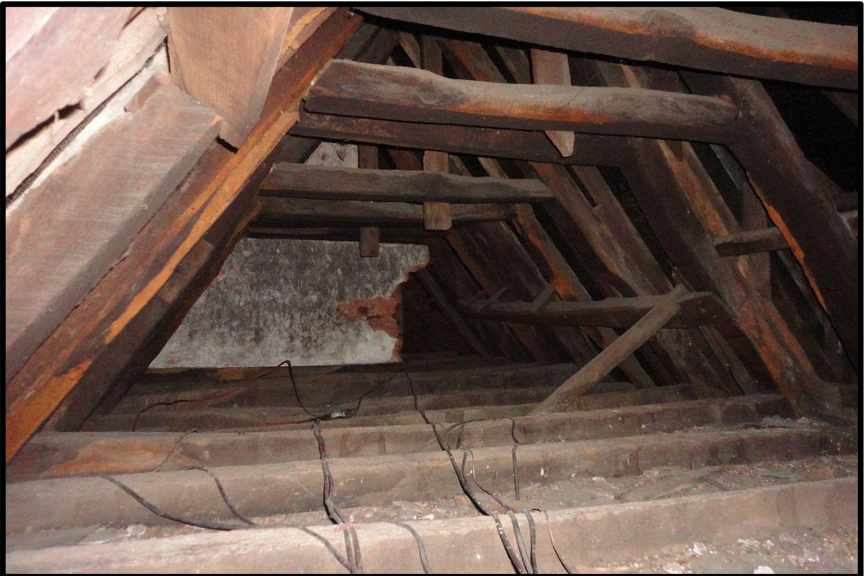
Fig. 32 View of the central section of the roof, looking east, showing common rafter trusses with upper and lower collars and the remains of a cob and timber partition to the eastern chambers.
