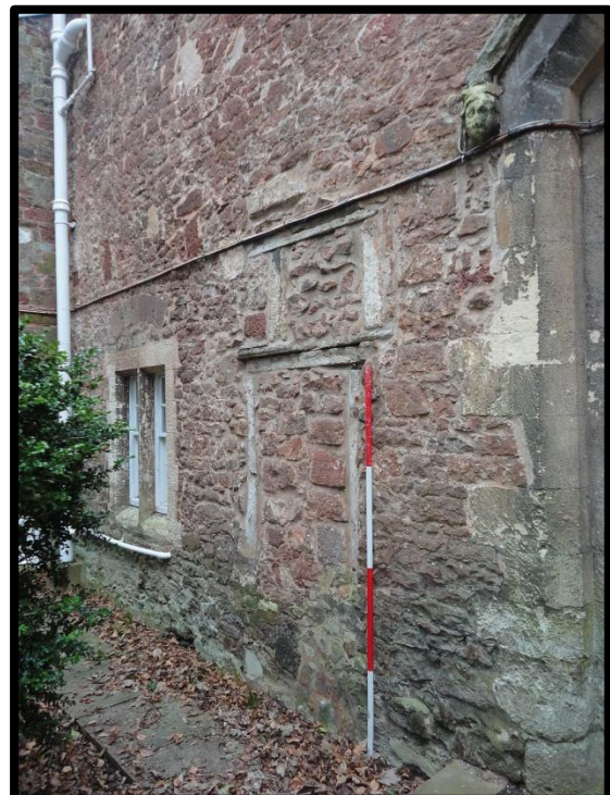
Fig. 17 Detail of the rear wall of the gatehouse to the east of the gateway, showing the remains of doorways and window openings cut into the walling.
