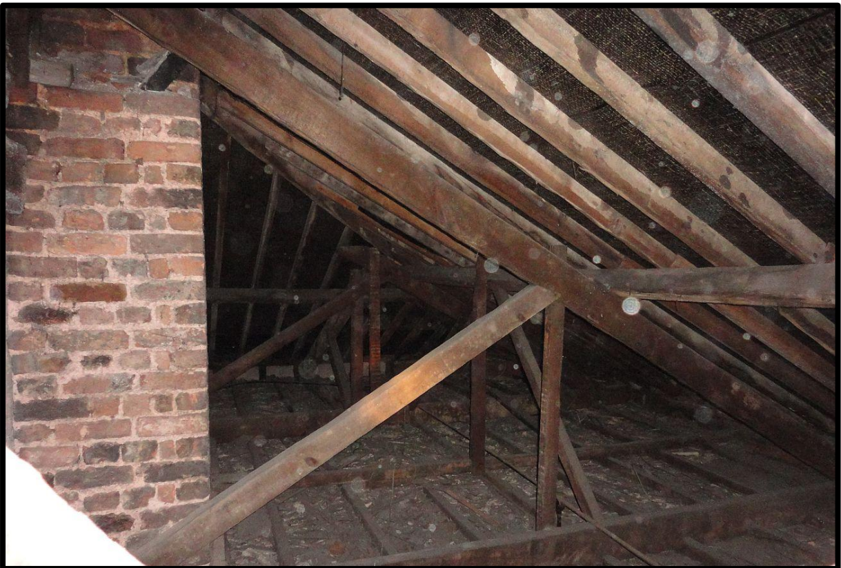
Fig. 34 View within the roof of the extension at the rear of the building showing crude 19th-century trusses and braces and the chimney rising against the rear wall.
