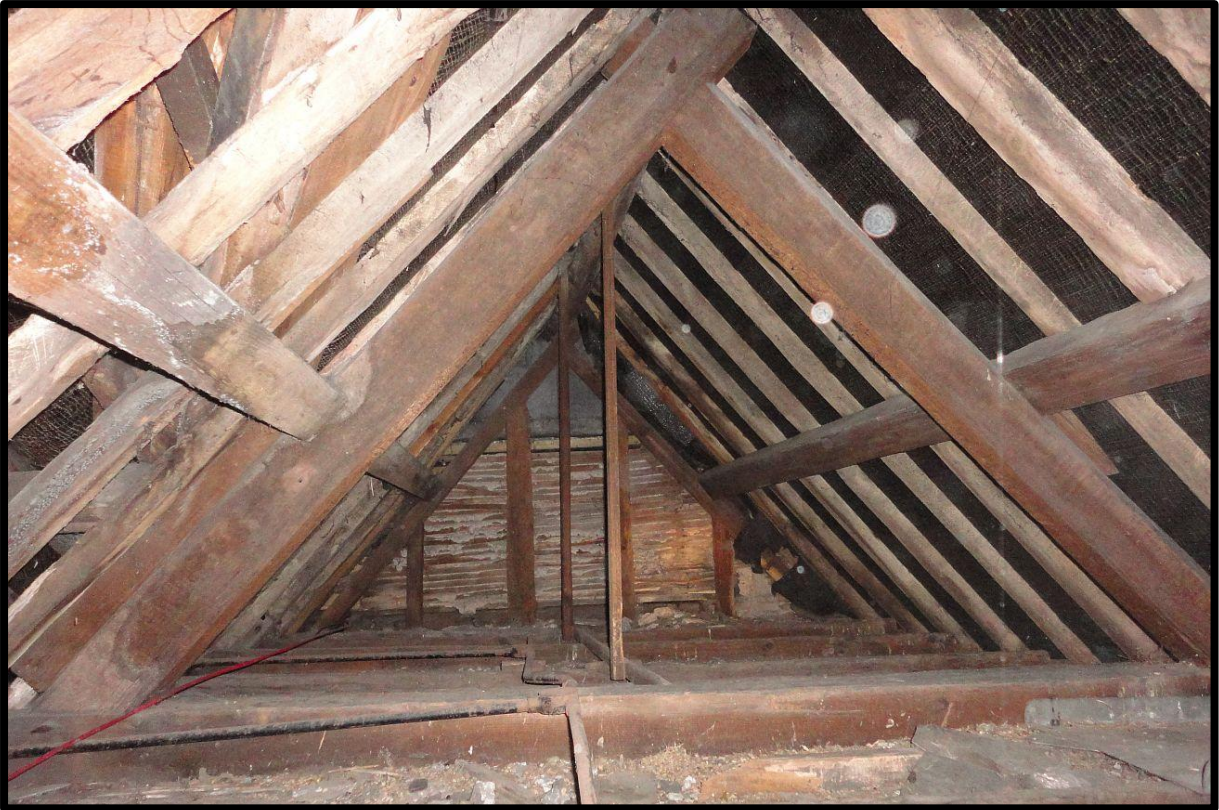
Fig. 33 View within the roof of the stair wing at the rear of the building showing typical trusses and the interruption of the end truss, perhaps to allow for a demolished chimney.
