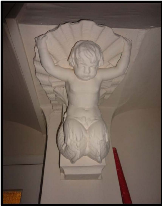
Fig. 25 Detail of the plaster caryatid representing a mer-boy supporting the arches between the rear stair wing and the main building
