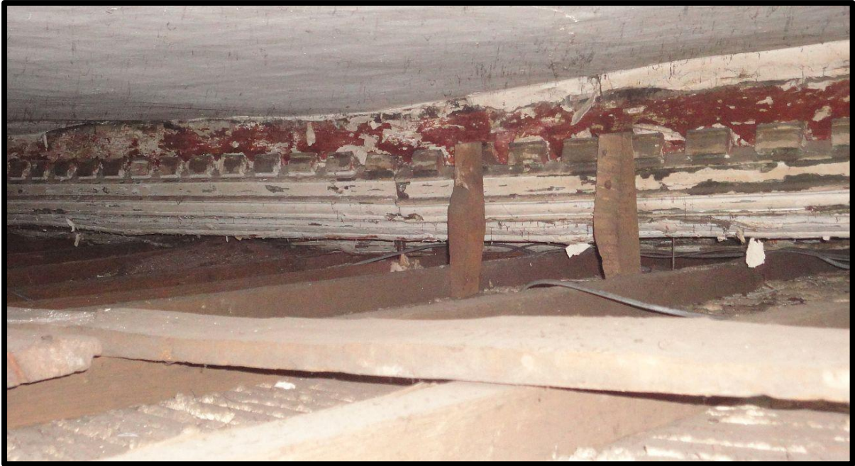
Fig. 27 View of the brattished beam crossing the large first-floor chamber at eaves level, now sandwiched between two later ceilings. The brattishing appears to be applied ornament decorating the structure, which probably crossed open space at eaves level and supported a crown post at its centre providing lateral bracing for the roof. The beam retains evidence of historic blue/green and red paint.
