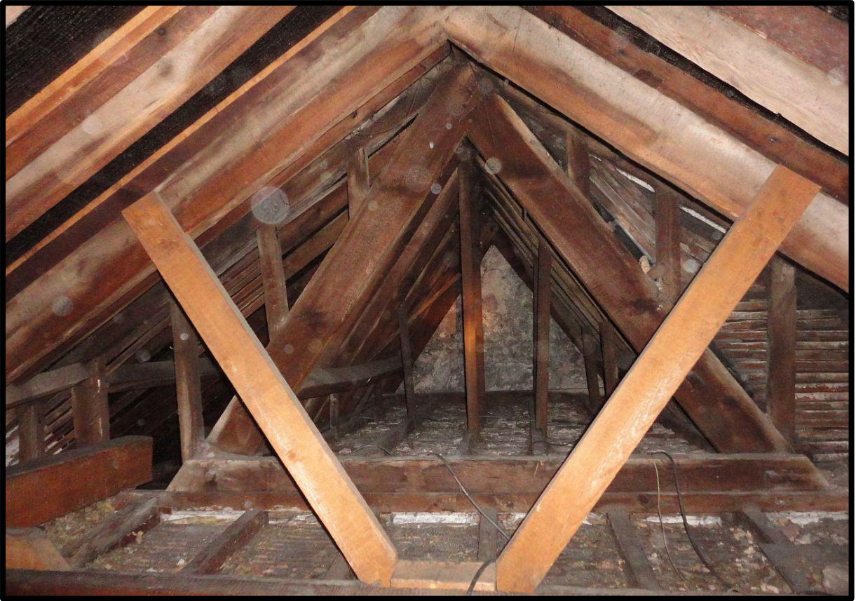
Fig. 31 View of the roof structure over the western attic rooms showing two phases of 18th- or 19th-century roofs replacing the original trusses over the western chamber.
