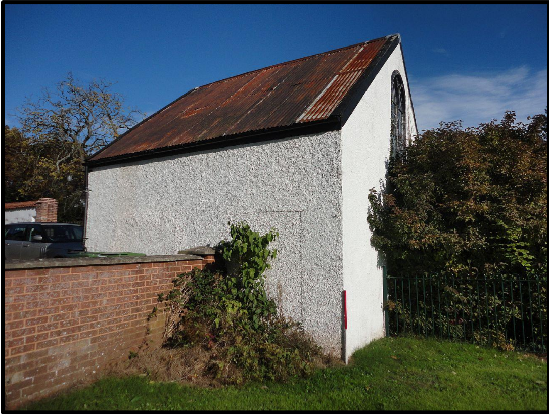
Fig. 10 Scars in the external render of the southern wall, showing the position of the original entrance (right) and a window alongside it.
