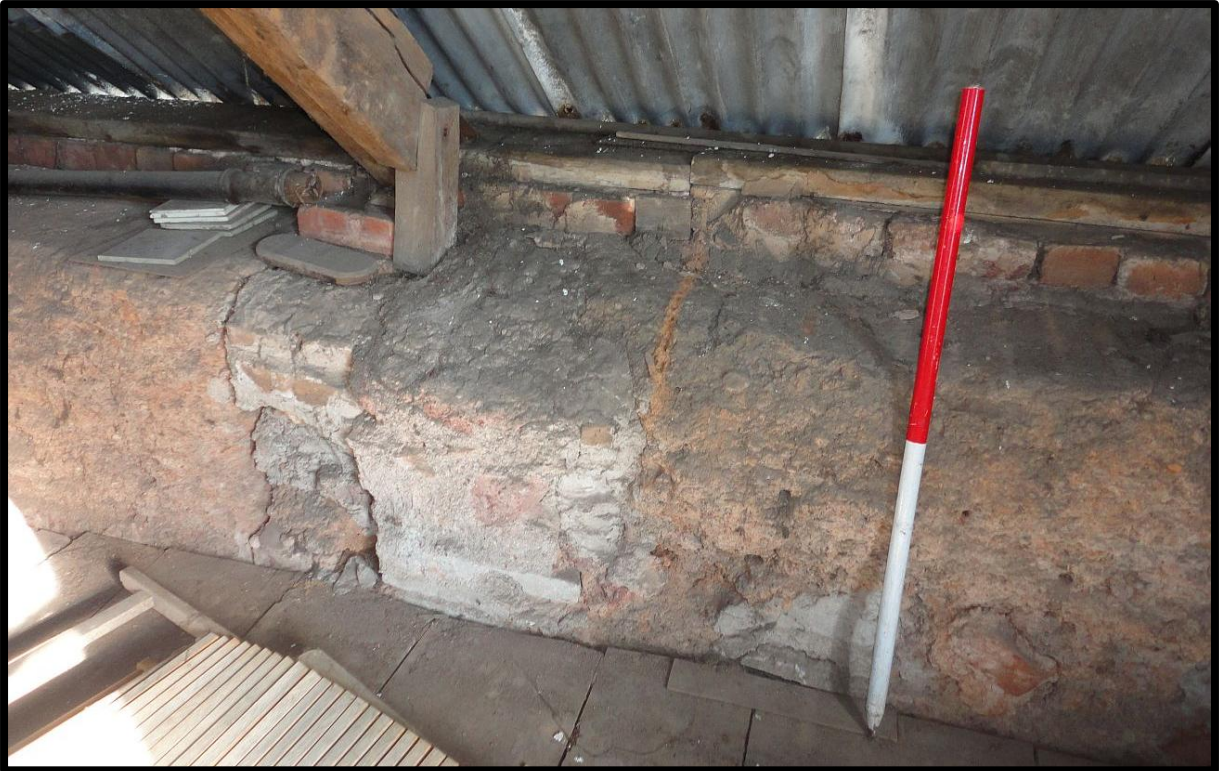
Fig. 12 View of the apparent wall scar and brick and stone intrusions above first-floor level.
