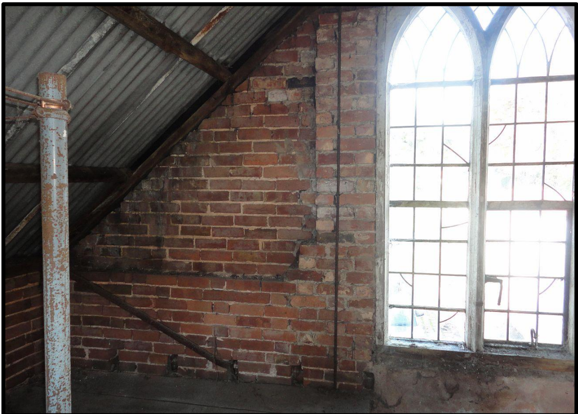
Fig. 9 Detail of the western gable wall above first-floor level showing the tall joist sockets and the evidence of insertion of the large Gothic gable window.
