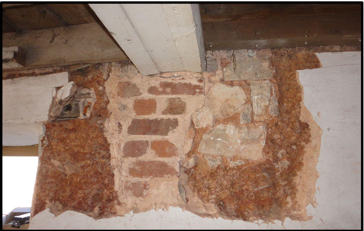
Fig. 13 View of the apparent wall scar and brick and stone intrusions below first-floor level, showing the stone patching interrupted at a height of 1.8m above floor level.
