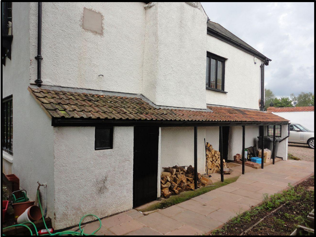
Fig. 14 The 19th- or 20th-century verandah on the south-east side of the house.
