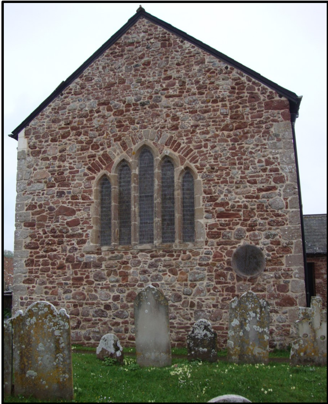
Fig. 18 The east wall of the church showing the best-preserved area of 13th-century masonry and the fine group of graduated lancets.
