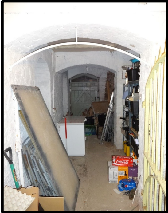
Fig. 28 The brick-vaulted passage to the south of the basement which may have been the access to the school.
