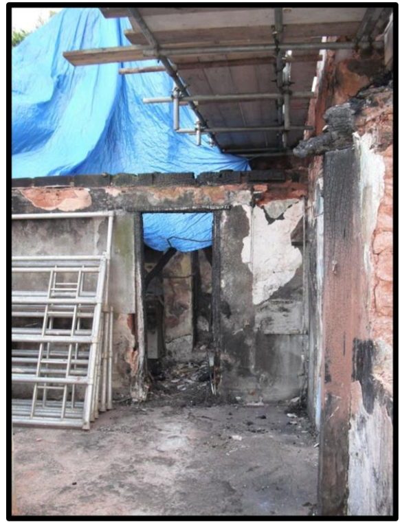
Fig. 21 The interior of No. 1, looking towards the 19th-century partition at its south-eastern end, showing the post and beam built into the north-western wall.
