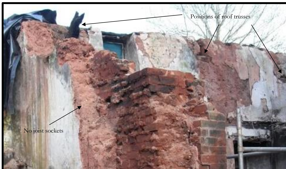
Fig. 25 Traces of three evenly-spaced roof trusses in the north-eastern wall of No. 1 Buller Square, two of which are without cruck posts (compare with Fig. 23).
