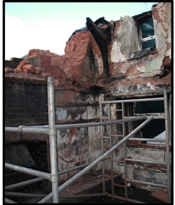
Fig. 23 View within the southernmost house, looking north, showing the remains of a jointed cruck truss with a curved blade surviving in the east wall close to the dividing wall.
