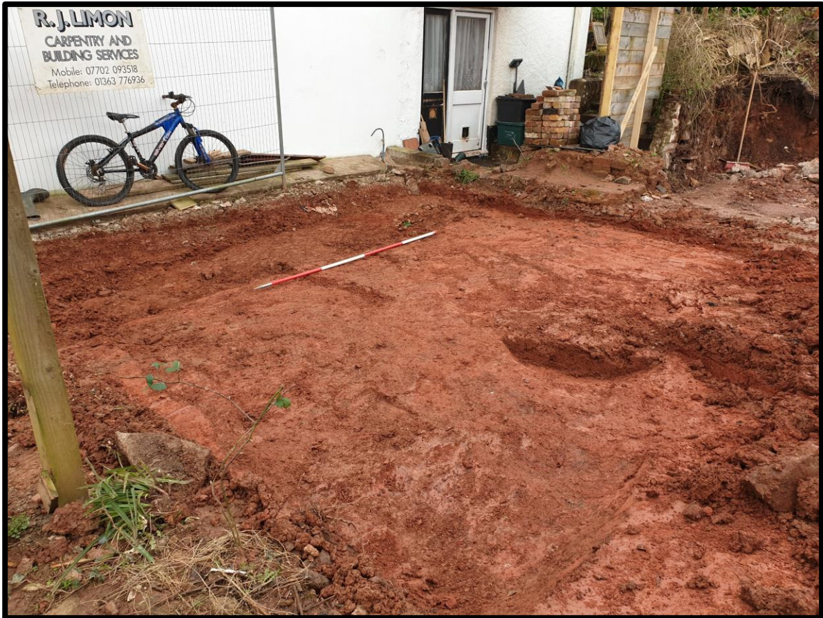
Fig. 33 General view of No. 2 Buller Square showing pit 102 in the foreground and cobbled floor (104) in the background. 2m scale. Looking north.
