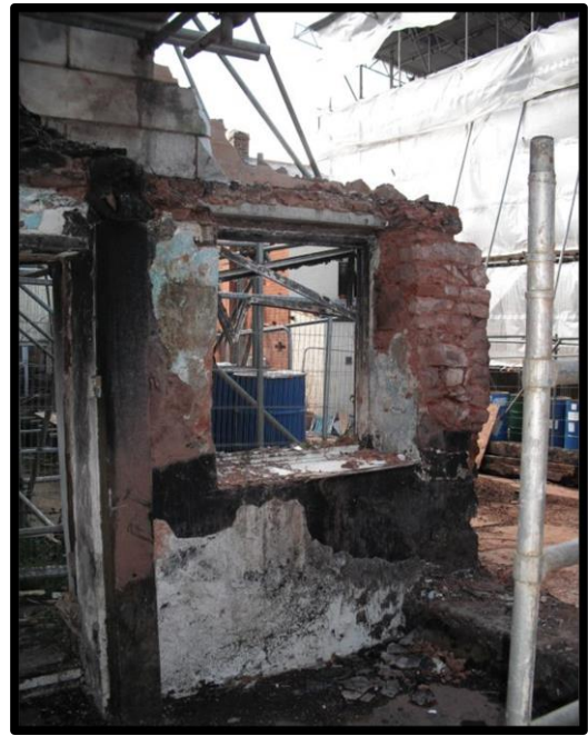
Fig. 19 View of the interior of the front wall showing the rebuilding of the jamb of the window and the post supporting a ceiling beam.
