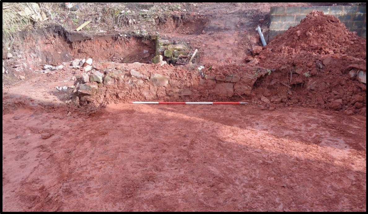
Fig. 26 The remains of the rear wall of the houses in 2020 during the reduction to the formation levels of the modern buildings, looking north east, showing the remains of stone underpinning to earlier walling, returning into the cross wall between the houses.
