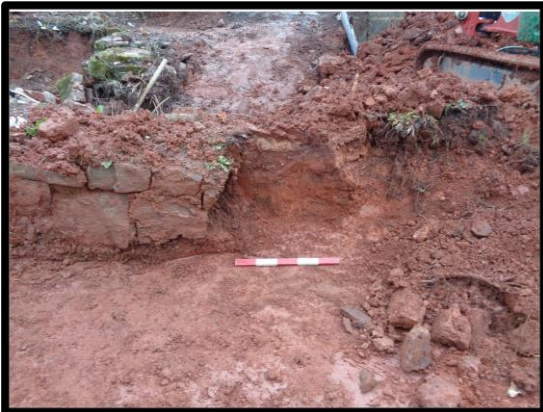
Fig. 27 Detail of the remains of the north-eastern wall during demolition showing the upstand of natural clay within the core of the wall.
