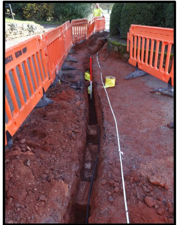
Fig. 48 A brick and stone feature lying to the north, seen looking south, interpreted as a possible culvert.
