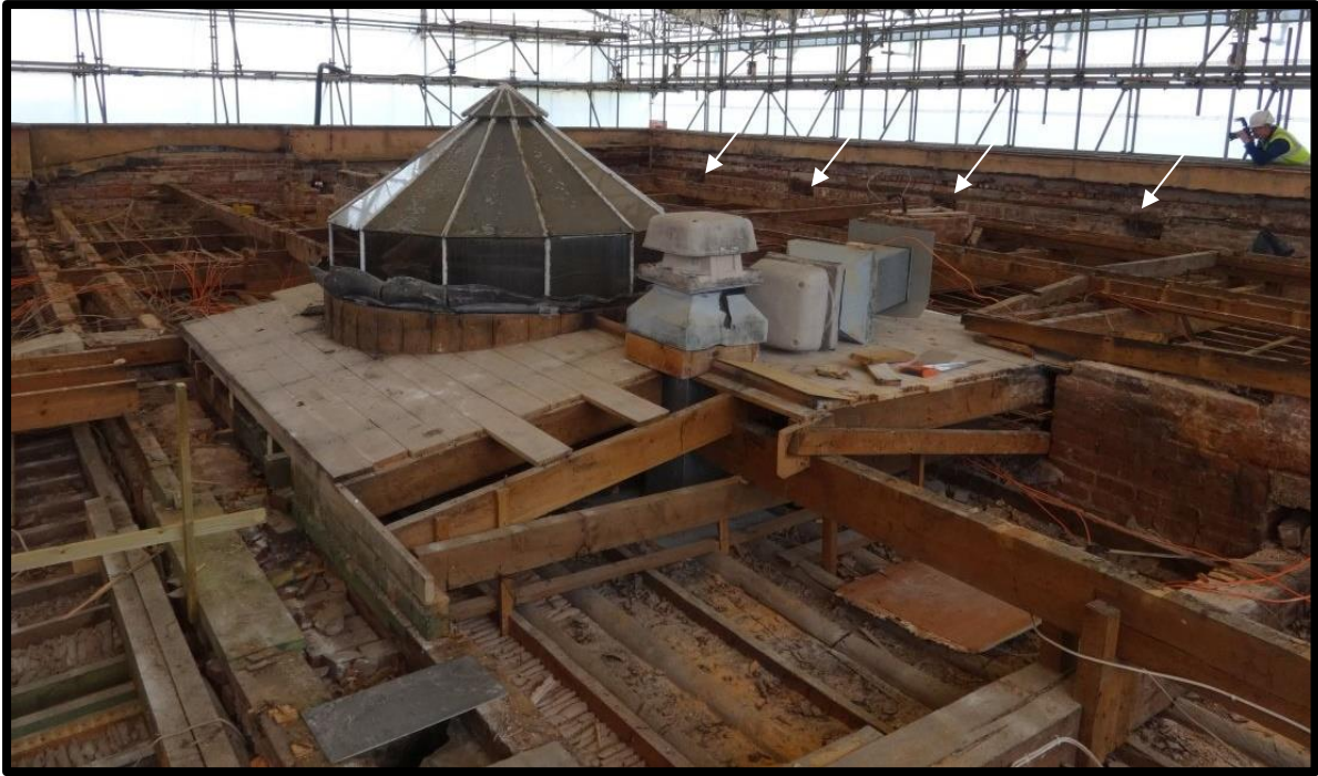
Fig. 27 General view of the south-western part of the roof looking south west, showing the central skylight of the first-floor corridor (before dismantling) and the regularly-spaced sockets (unrelated to either the 18th-century or modern roof structures) in the west wall (arrowed).
