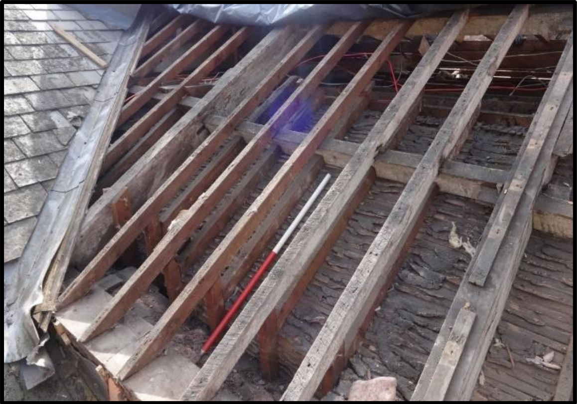
Fig. 43 Secondary rafters and plastering underlying the roof timbers of the service range at the eastern extremity of the northern plane of the roof.
