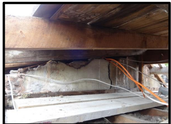
Fig. 42 The remains of wall plastering above the existing ceilings, showing that the rooms were formerly open to the roof.
