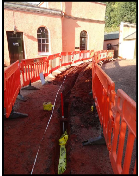
Fig. 46 the northern part of the trench curving towards the angle of the service range and the rear service court.
