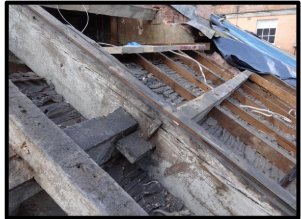
Fig. 40 The staggered purlins and plaster torching of the original roof on the northern side of the range.
