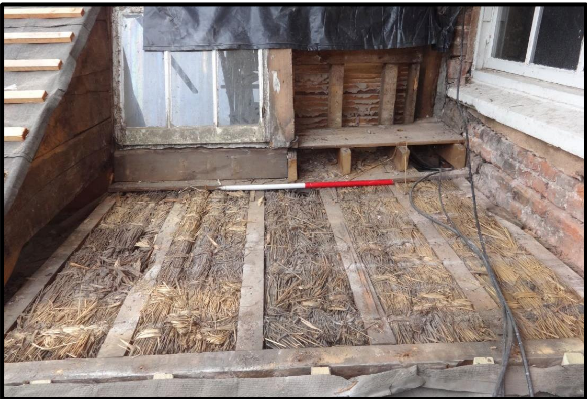
Fig 44 Straw bundles tightly packed between the joists of the flat roof at the extreme western end of the north plane of the service wing roof, presumably providing some form of insulation.
