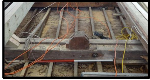
Fig. 32 Detail of one of the original king posts supporting the trusses, with sockets for diagonal braces. The later tie is shown behind the original.
