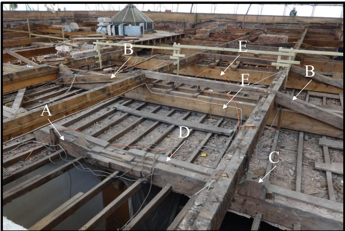
Fig. 30 General view of the western part of the roof looking south, showing the deflection of the original tie beams (A) and the weak construction at the centre due to original and later mortices; the remains of the 19th-century trapezoidal roof structures (B); the truncated king-post trusses of the 18th-century roof (C); the additional tie beams (D) and further additional ties reinforcing them (E).
