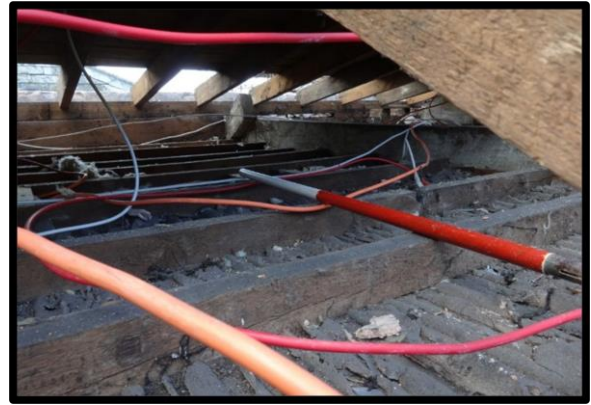
Fig. 38 Evidence of earlier trusses, sawn-off short, from a roof with two equal pitches, surviving beneath the roofline, above the 19th-century ceilings.
