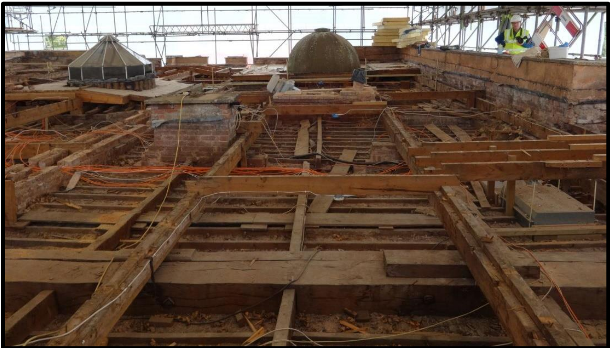
Fig. 20 The removal of the modern roof structure in April 2017, looking north, showing the remains of the modern roof represented by chases in the rendering, and beneath this an earlier structure, the joists remaining, which stepped down in three broad shallow inclines toward gutters flanking the central raised flat over the first-floor spine corridor.
