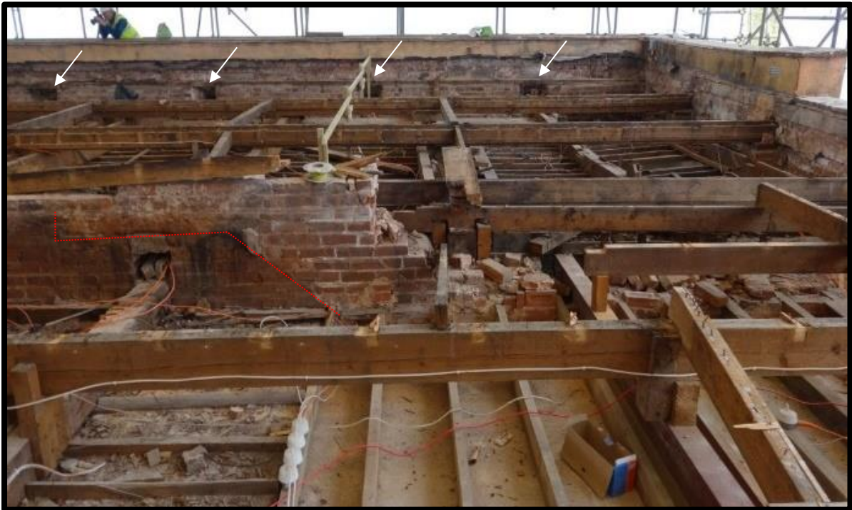
Fig. 28 General view of the north part of the roof looking west, showing modern interventions in the area of the main staircase (right foreground), a curious angled scar resembling the string of a staircase on the chimney in the spine wall, rising to a higher level than the 18th-century roofs (red) and, beyond this, regularly-spaced sockets (unrelated to either the 18th-century or modern roof structures) in the west wall beneath the later parapet (arrowed).
