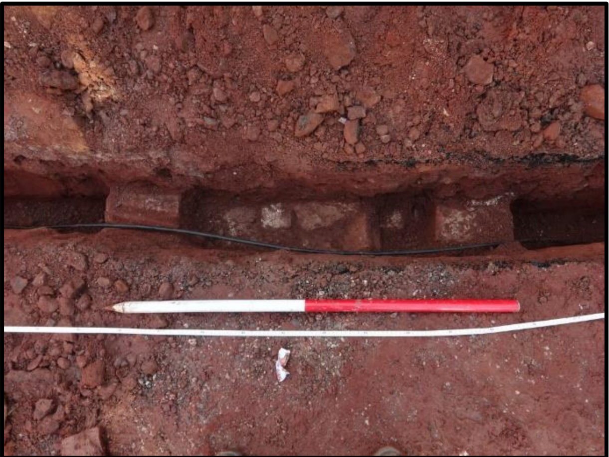
Fig. 50 The possible culvert with masonry sides and a central channel, observed in the electrical trenching.
