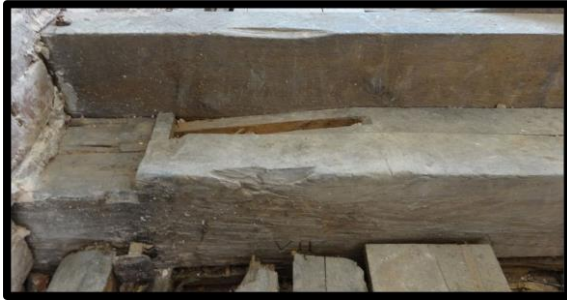
Fig. 31 The end of one of the tie beams showing the socket for one of the original principal rafters. A later tie is shown bolted against this, marked 'VII'.
