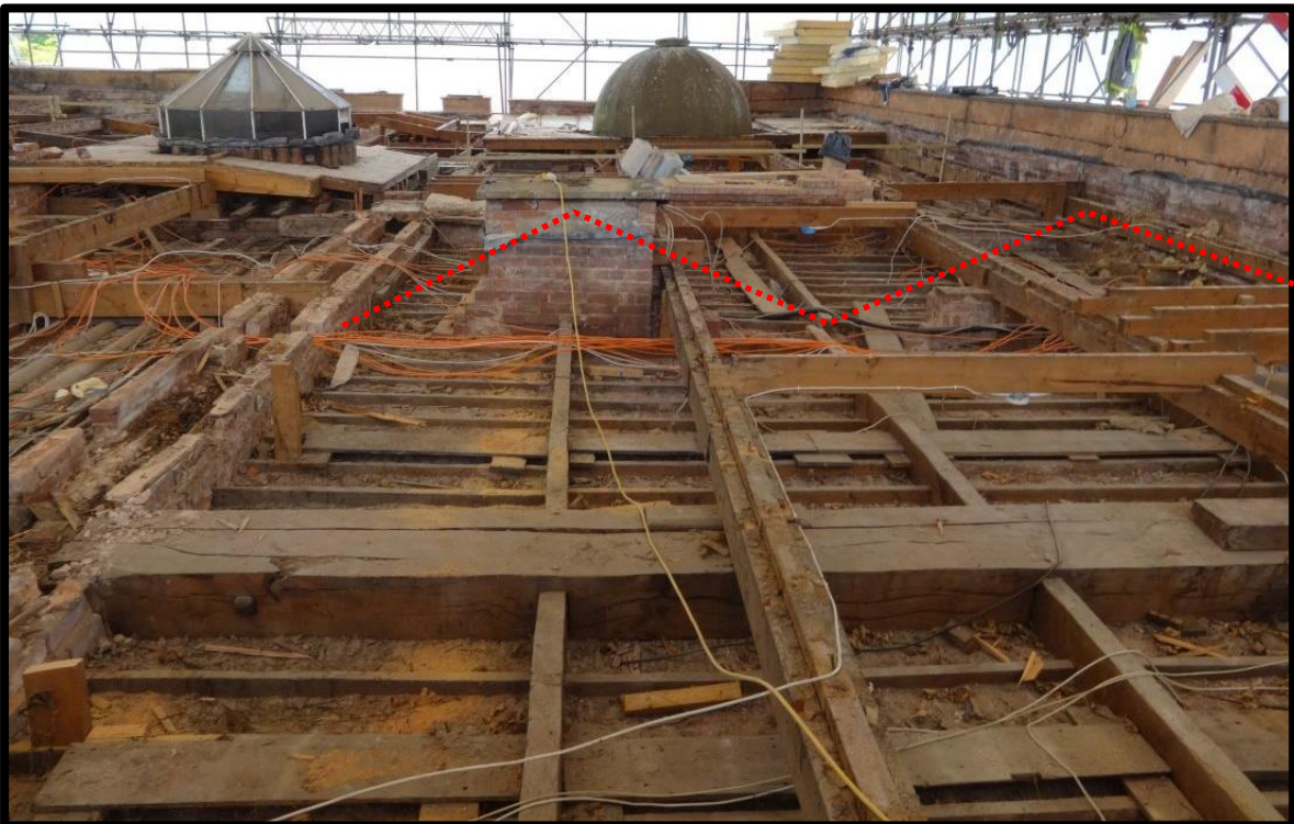
Fig. 24 View of the eastern part of the roof looking north towards the dome over the staircase, showing the scar of the double roof on the drawing room chimney and the flashing for the flat roof structure which succeeded it (the approximate profile of the pitched roof is indicated in red).
