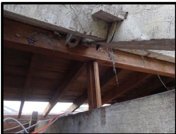
Fig. 41 The whitewashed surfaces of the timbers of the northern side and also the tusk-tenoned and wedged peg of one of the purlins.
