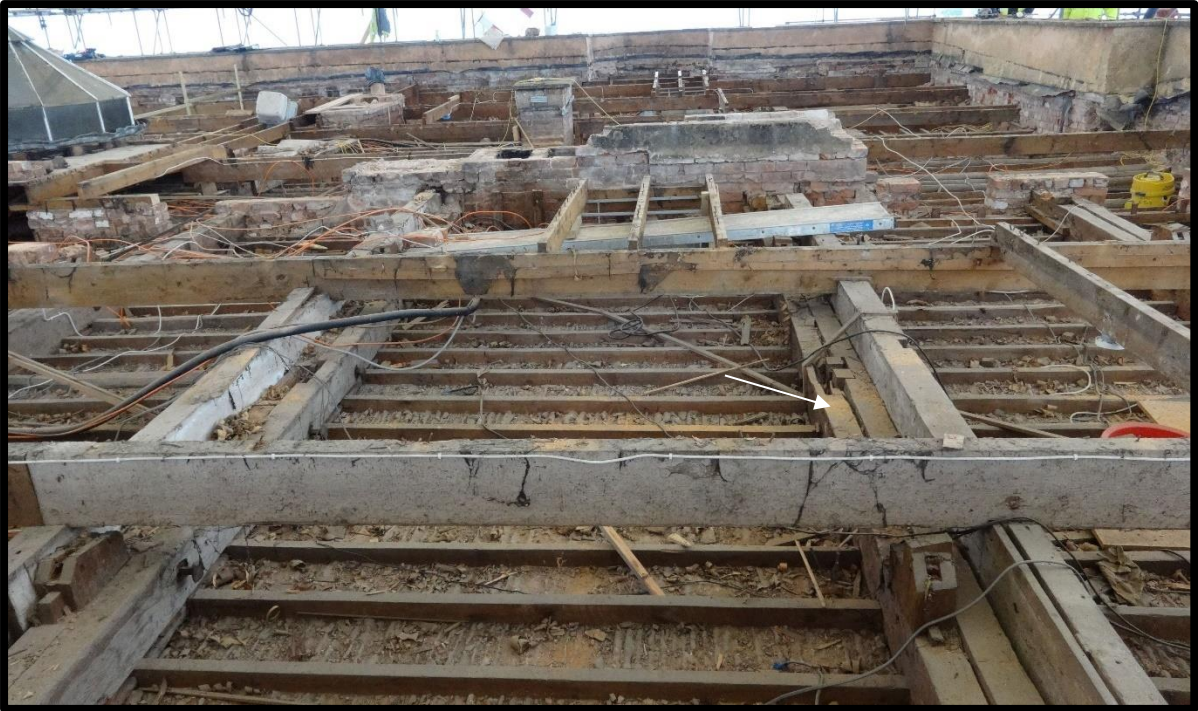
Fig. 29 General view of the south part of the western roof looking east, showing the trebled ties of successive attempts to reinforce the 18th-century roof (arrowed) and the remains of sawn-off king-posts and mortices relating to the original structure.
