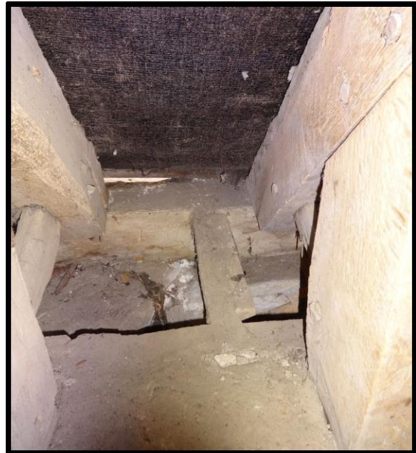
Fig. 28 Detail of the short dovetail ties linking the wall and eaves plates across the wall tops. Note the apparently good condition of these members.
