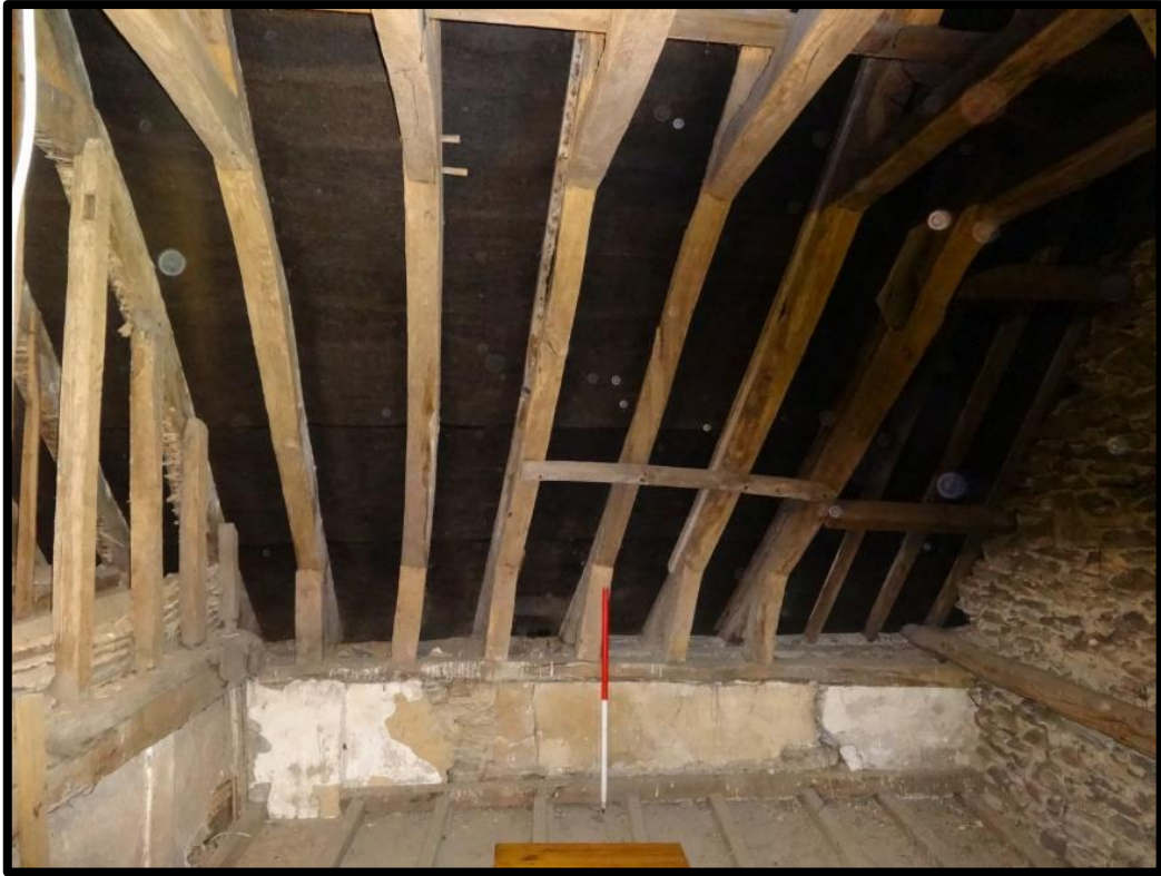
Fig. 24 View of the roof structure, looking west, showing the evidence for historic partitions and plaster finishes to the smaller first-floor room; also the complete rebuilding of the northern gable above this level.
