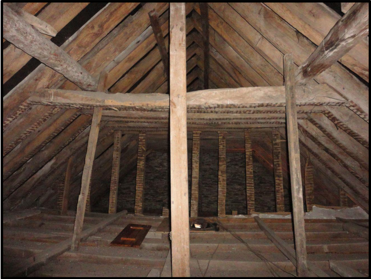
Fig. 26 View of the roof structure over the west wing showing the inserted flat ceiling in the southern part of the first floor and the evidence for lath and plaster forming a high, canted ceiling. The 'purlins' on either side are modern insertions.
