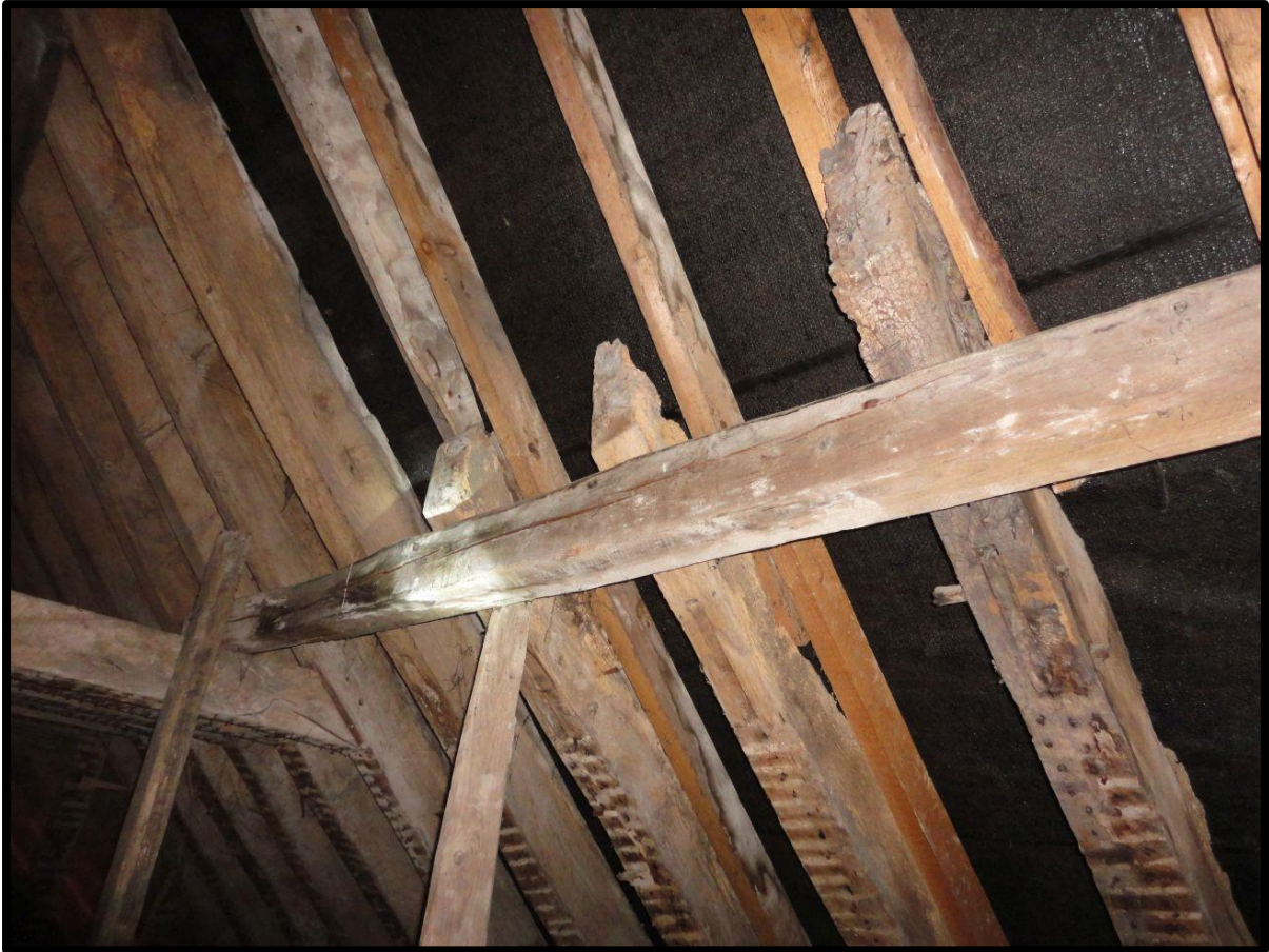
Fig. 29 Detail of the truncated rafters at the centre of the roof showing sockets for the collars, now sawn short, inserted purlins and re-shaped ends to each rafter allowing them to rest against the chimney.
