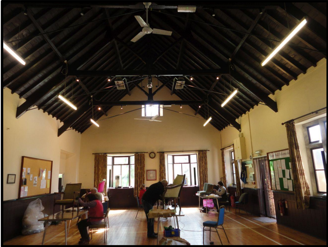
Fig.34 View of the hall looking east, showing the character of the roof.
