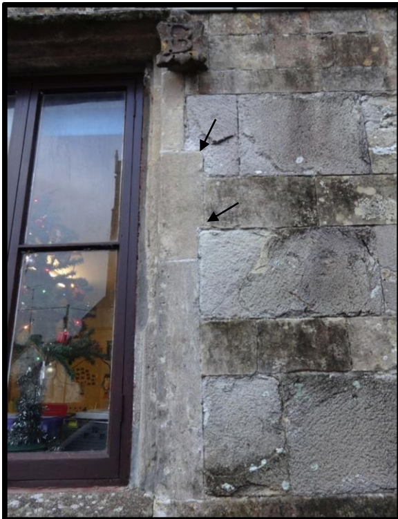
Fig. 17 Detail of one of the ground-floor windows showing inconsistencies in the jointing of the masonry, suggesting that the windows are inserted.
