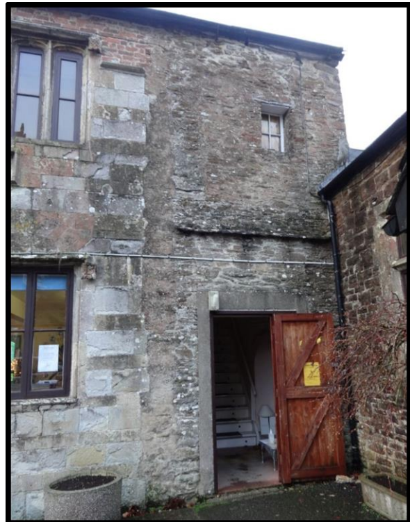
Fig. 18 Detail of the northern part of the façade showing the scar of the demolished porch and the modern entrance to the staircase.
