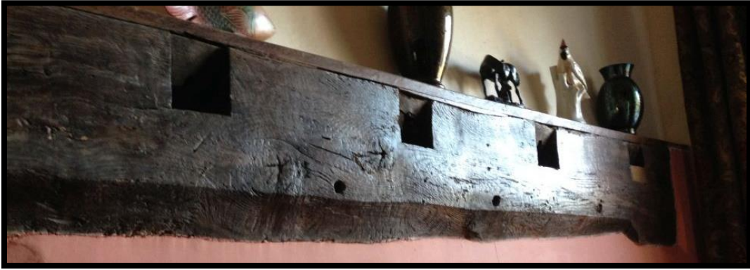
Fig. 21 The beam on the south-western side of the cross passage, supporting the floor of the chamber over the entry, showing the character of the sockets for the floor joists and the peg-holes, perhaps for a short spere, beneath them.
