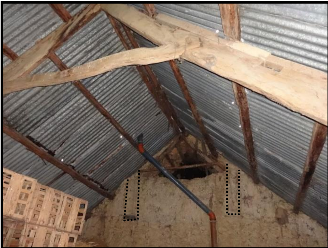
Fig. 16 The upper part of the wall separating the house from the shippon showing two vertical chases (dashed) for short wall posts, probably for braces to purlins or perhaps 'arcade plates' in the lost medieval roof.
