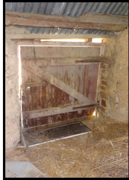
Fig. 18 The plank door to the loft of the shippon, showing reused hinges.
