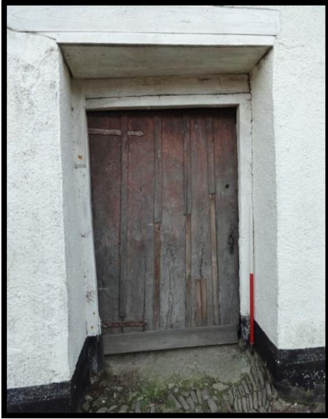
Fig. 17 The plank door to the shippon, possibly dating from the 18th century.
