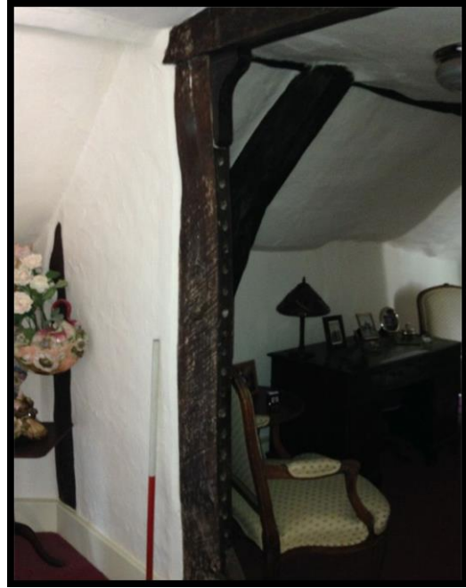
Fig. 25 Detail of the partition between the chamber over the entry and the hall, showing the hall roof truss beyond.
