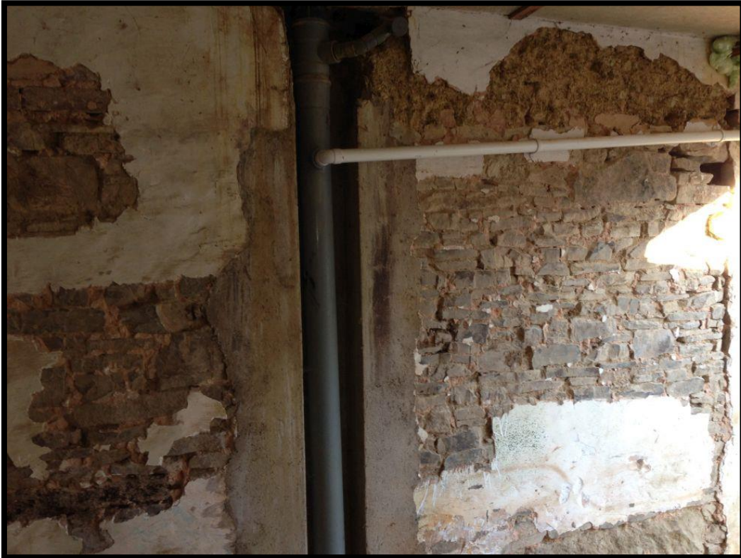
Fig. 15 The stone and cob wall separating the house from the shippon, probably a 17th-century insertion, showing modern intrusions into the fabric.
