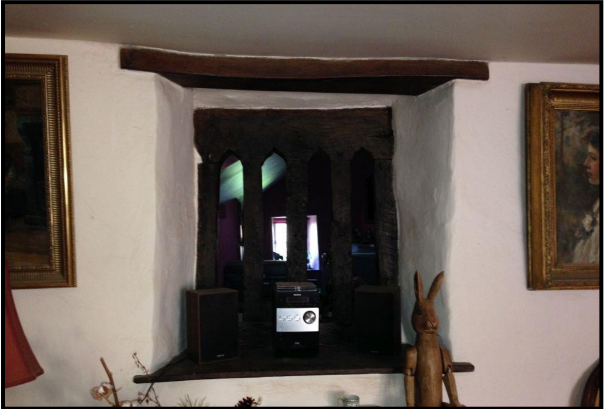
Fig. 27 The rear window of the hall, possibly of 14th- or early 15th-century date, now opening onto the later outshut at the south-western side of the rear wing
