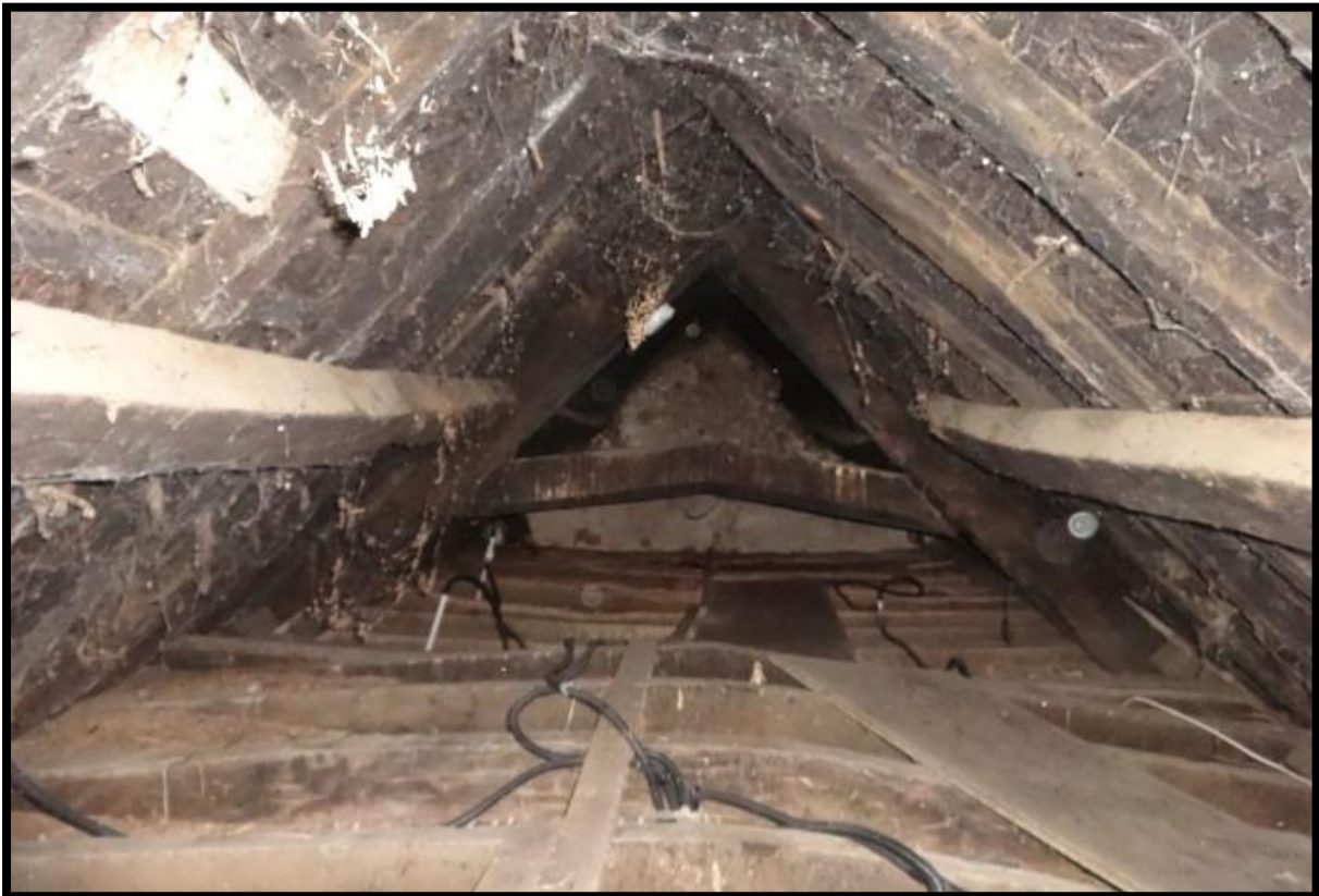
Fig. 26 The roof of the hall seen from the void at the end of the shippon, showing smoke-blackened medieval roof timbers, including a main truss with a high cranked collar, diagonally set purlins and exposed, blackened thatch. Beyond, plaster extends to the apex of the roof and, in the foreground, the cranked timbers of the ceiling over the chamber over the entry show light smoke-staining from the open hearth.
