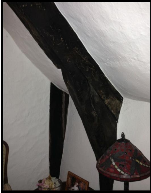
Fig. 24 Detail of one of the hall roof trusses showing its relationship with the partition behind.
