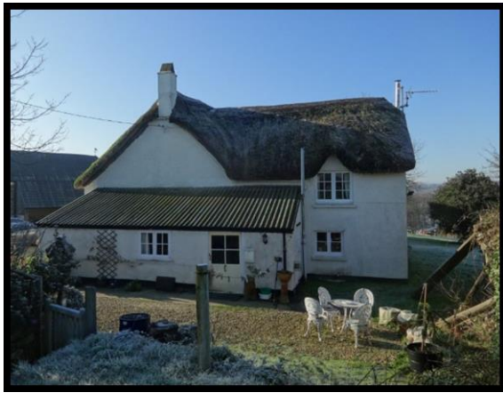
Fig. 13 The north eastern gable of the farmhouse showing the rear extension, lean to and the collapsing walls of the ruined building to the north (extreme right).
