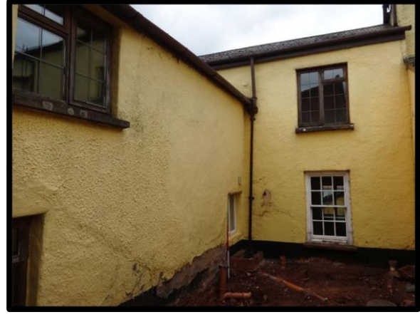
Fig. 7 Elevation of the rear range from the rear courtyard showing the substantial masonry wall (left) and the surviving sash window in the south-western part of the main range, (right).
