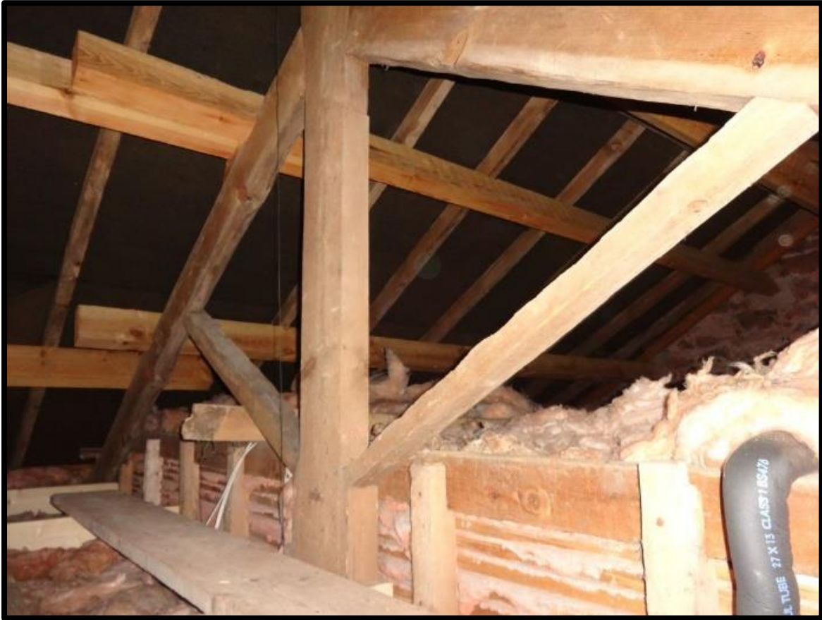
Fig. 19 The roof space over the main range showing King-post trusses, replacement purlins and the raised ceiling over the south-western rooms.
