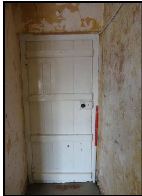
Fig. 11 The plank door to the north west of the 'kitchen' now hung on modern hinges.
