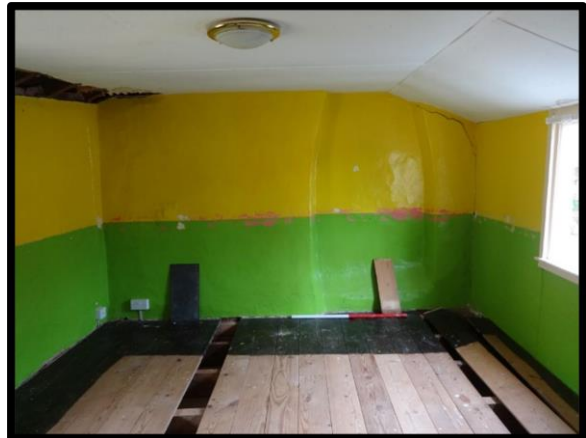
Fig. 21 View of the first-floor room in the rear range showing the recess for a demolished chimney.
