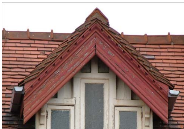
Plate 11: Detail of decorative bargeboards as seen on south, west and north elevations
