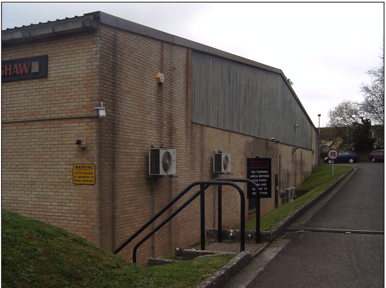
Plate 2: View showing reduction of ground surface of main factory building looking south
